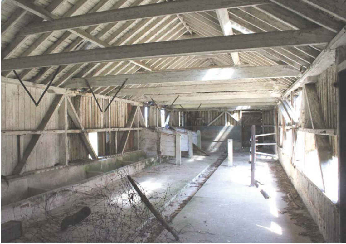
Illus. 5. Interior of early-20th century milking parlour (5) from west showing the original wooden stalls and secondary concrete feeding trough to left.
