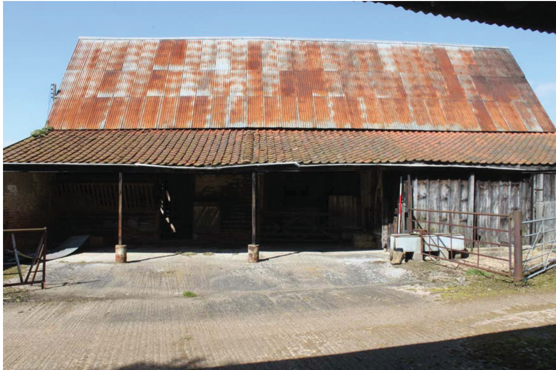
Illus. 3. Exterior of barn (1) from south showing the 20 th century shelter shed (3) to left and the enclosed 20 th century loose boxes (4) to right. The Ordnance Survey of 1927 appears to show a central porch flanked by open shelter sheds here.
