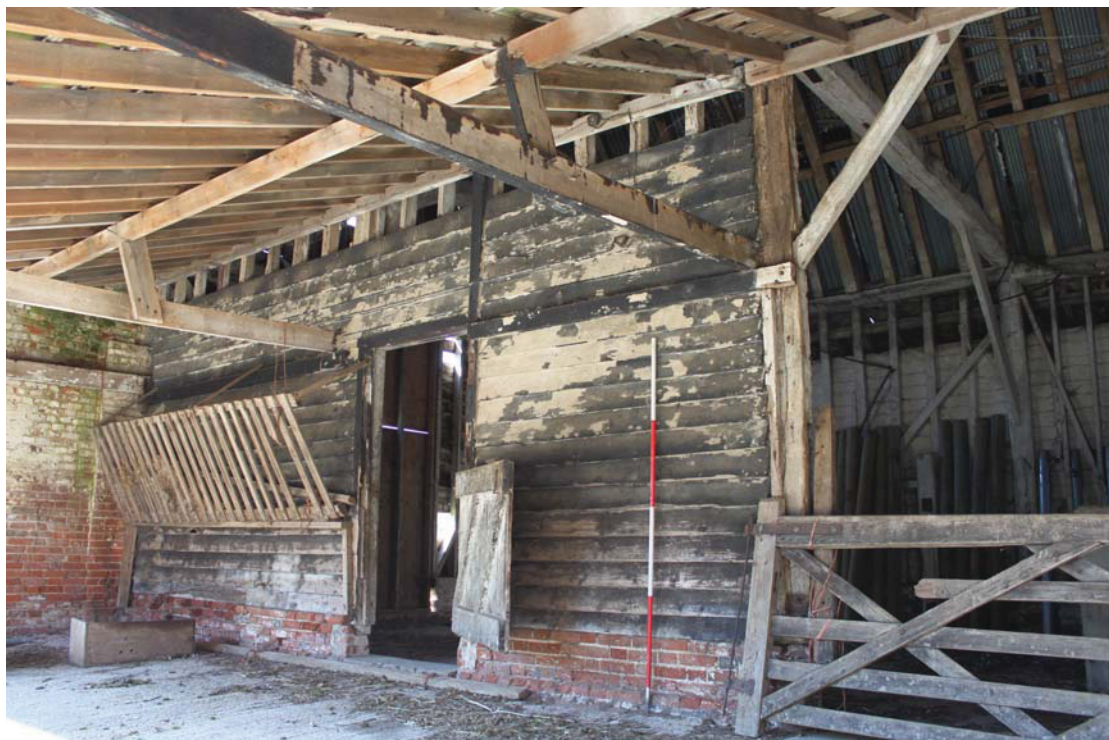
Illus. 4. The western end of the barn's southern external elevation within the 20 th century lean-to shelter shed (3), showing the principal entrance to right and a secondary door to the left. Note the 20 th century hay rack for cattle and the grey pigment to the apparently original weatherboarding
