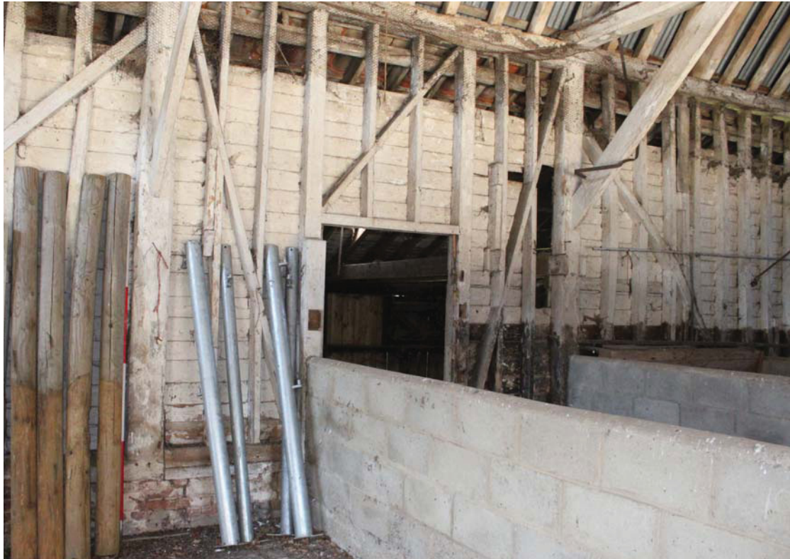
Illus. 9. Central bay of northern internal elevation of barn (1) showing the narrow, secondary timbers of the late-19 th century which block the original full-height doorway in this position (matching that to the south). The original ground sill to the left terminates at the storey post.
