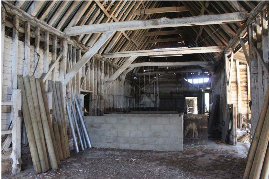
Illus. 7. Interior of barn (1) from west showing southern entrance to right and arch-braces of threshing bay to left. Note the empty mortises in the tie-beams for the missing southern braces and the inserted cement-block loose boxes for pigs or calves.
