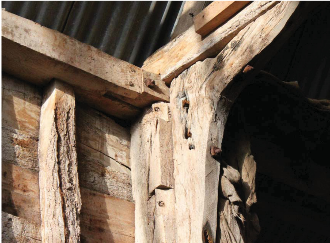
Illus. 9. Detail of face-halved and bladed scarf joint of northern roof-plate behind knee-brace to west of central bay. Rafter housings are visible in the re-used storey post (originally a roof-plate).
