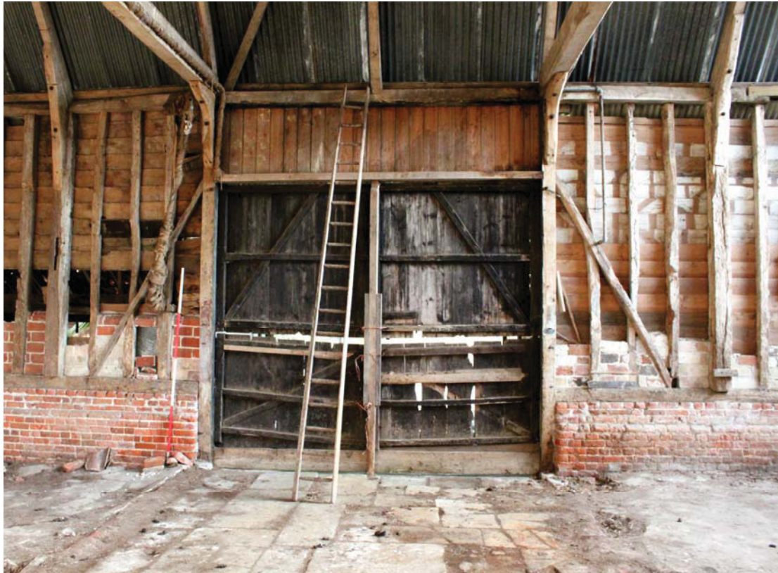
Illus. 7. Interior of southern entrance doors in central bay of barn (1) showing the stone floor and double-hung doors with retaining board. The original doors rose to the roof-plate, as indicated by mortises for door jambs in the roof-plate.
