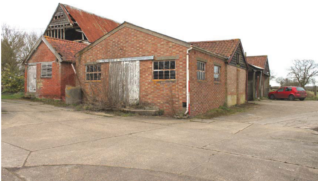
Illus. 2. Exterior of farm complex from south-west showing the brick loose box (7) in foreground and the brick feed store (4) to left. The barn (1) is visible in the rear to left, and the southern shelter shed (8) and covered cattle yard to right.
