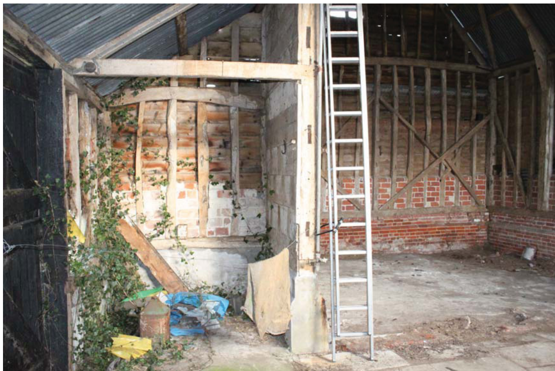
Illus. 10. Interior of lean-to porch (1a) from west showing eastern grain storage bay with butted boarding to wall of barn. The northern doors are visible to left, and the interior of barn to right.
