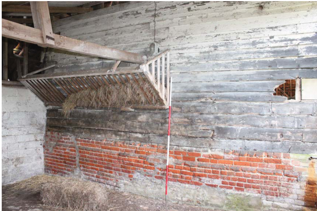
Illus. 3. Eastern external gable of barn within the 20 th century cement-block lean-to bullock shed, showing the hay rack and original grey pigment to the weatherboarding (beneath secondary whitewash).
