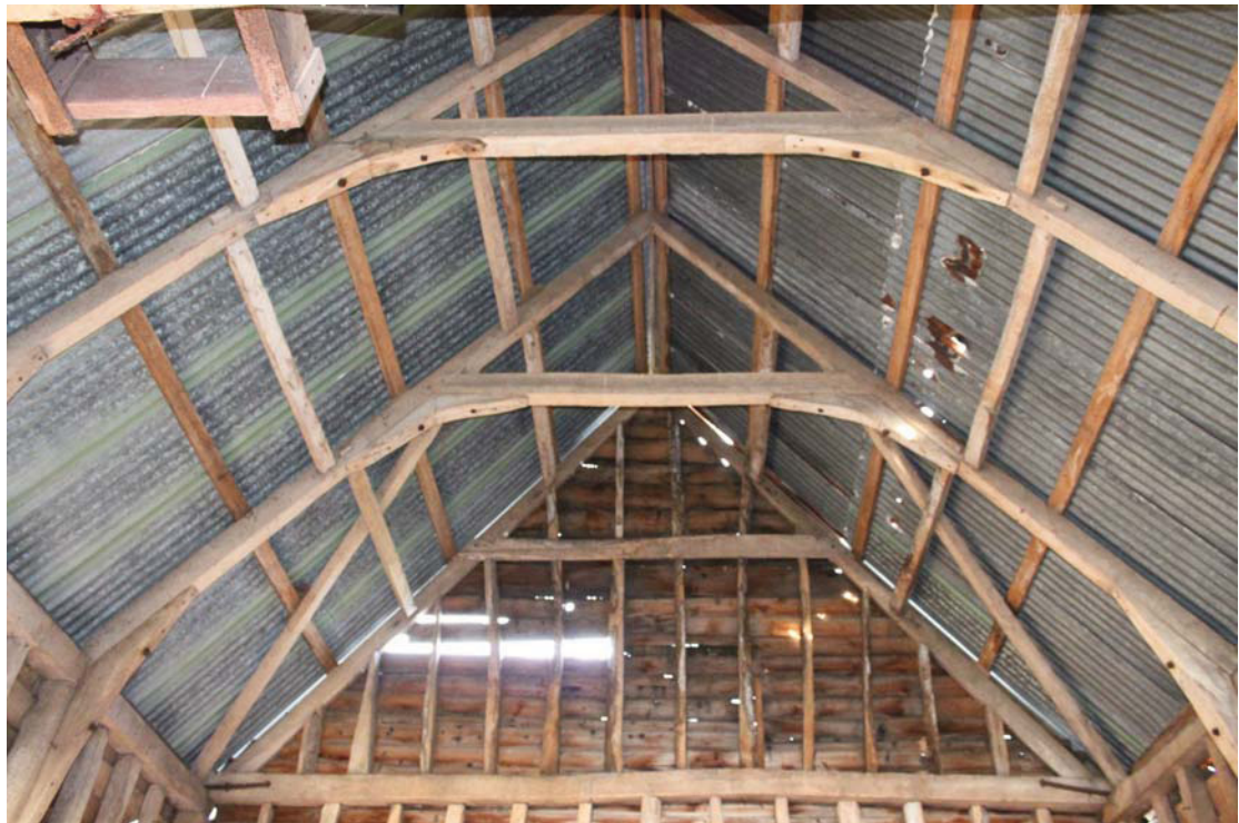
Illus. 6. Eastern roof gable of barn (1) showing the A-framed roof trusses with bolted knee-braces found in both end-bays. Note the original staggered butt-purlins and the secondary rails of the corrugated iron which replaced the thatch.
