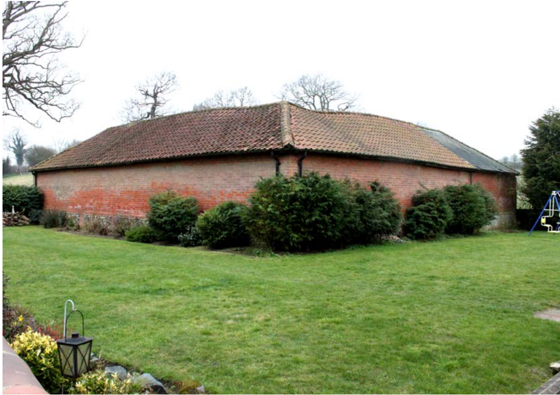
Illus. 3. Exterior of complex adjoining garden of Rivers Farm Cottage to north showing remaining section of original slate to right.
