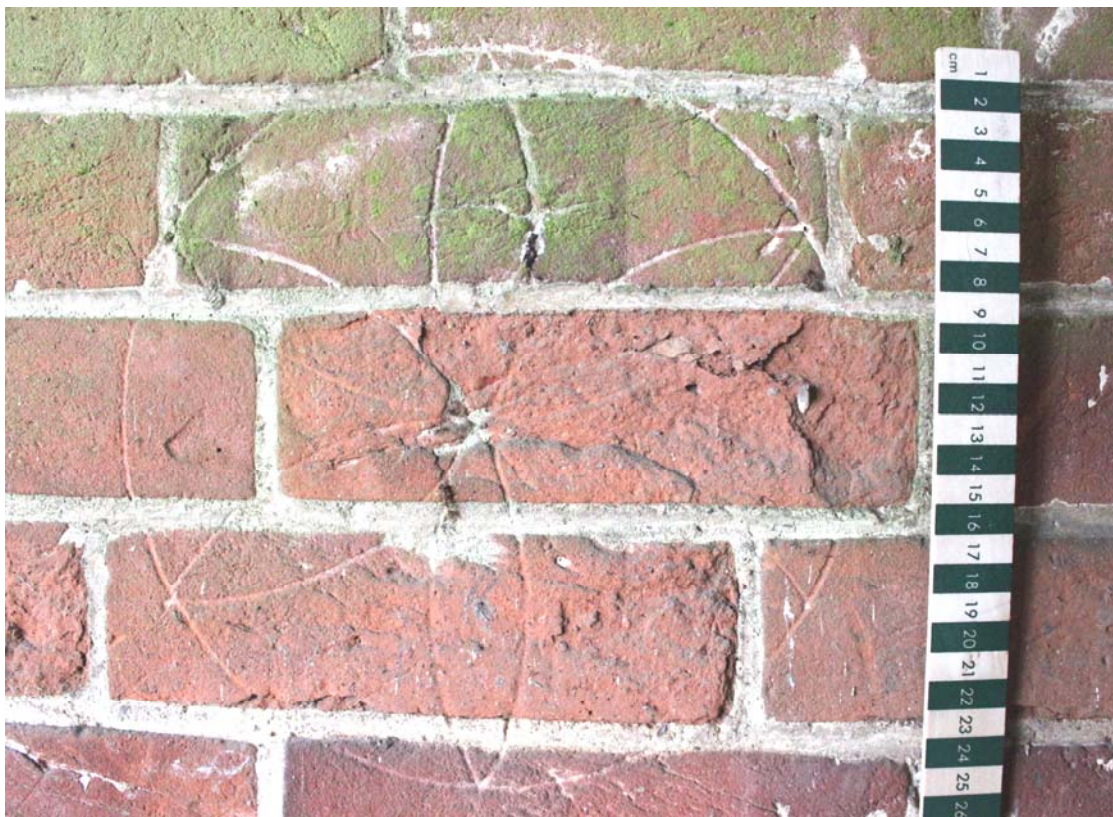
Illus. 6. Detail of 'daisy wheel' apotropaic (evil-averting) mark inscribed on brickwork at southern end of eastern exterior of barn (1) close to the yard entrance.
