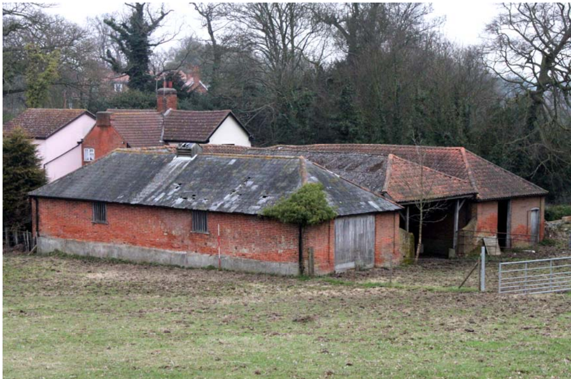
Illus. 2. Exterior of barn complex seen from adjoining high pasture to south-west showing original slate roof of feed barn (1) to left and secondary pantiles of 20 th century yard roof in centre (5) and shelter shed with feed store (3 & 4) to right.
