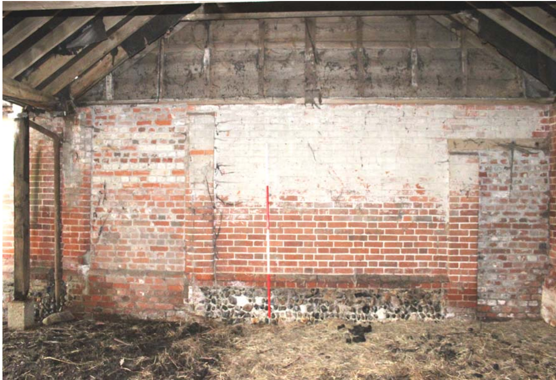
Illus. 7. Eastern exterior of calf shed (2) seen from shelter shed (3) to east showing flint plinth between blocked original doors to right and left.
