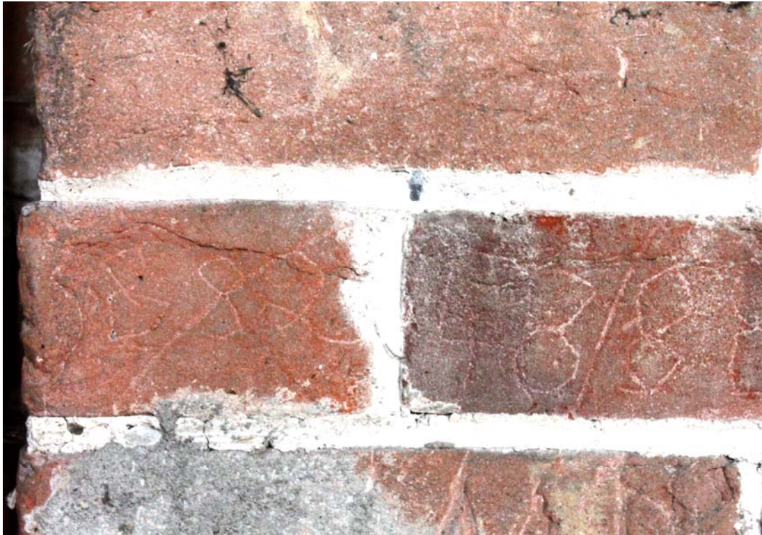
Illus. 9. Detail of inscribed date 1882 on internal brickwork to north of door between barn (1) and yard (5).
