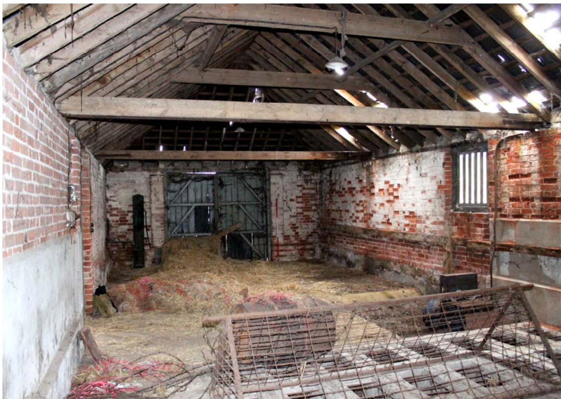
Illus. 8. Interior of barn (1) from north showing 20th century grain dryer in foreground with original gable doors (with decorative cast-iron brackets) and water pump in rear. The sliding louver to the right is also an original feature.
