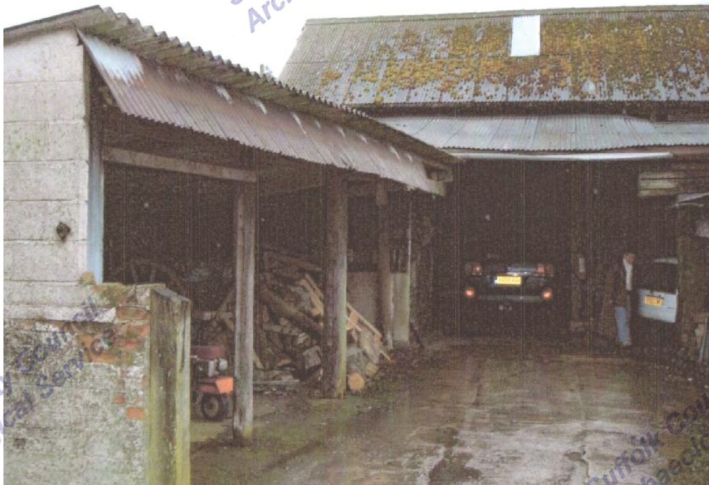
Illus. 10. Circa 2008. Eastern exterior of barn showing lean-to shed (2) with shelter shed (4) to left before demolition work began.
