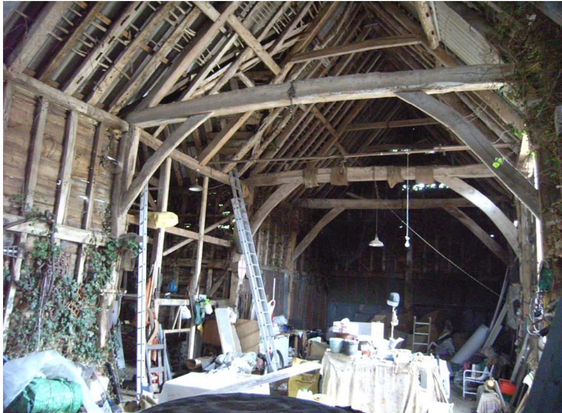
Illus. 7. Interior of barn from south showing central porch (1a) to left.
