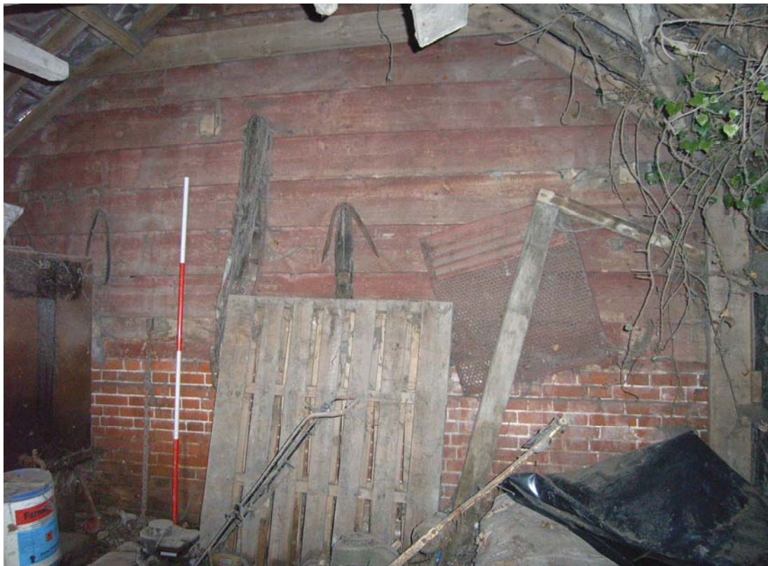
Illus. 4. Eastern exterior of barn exposed within northern shed (4) showing the extensive and apparently original red ochre to the weatherboarding.
