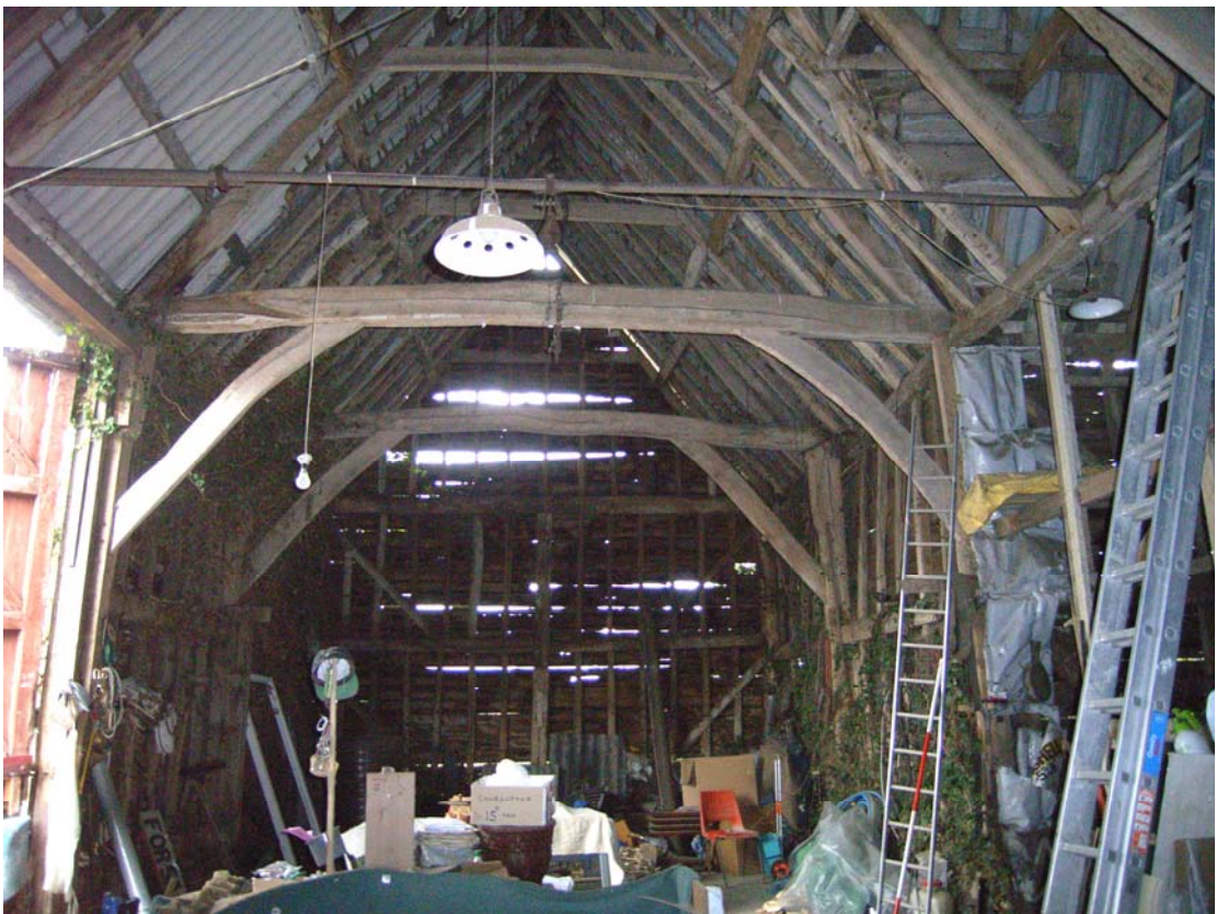
Illus. 6. General view of barn interior from north showing eastern entrance in central bay to left and intact arch-braces to tie-beams.
