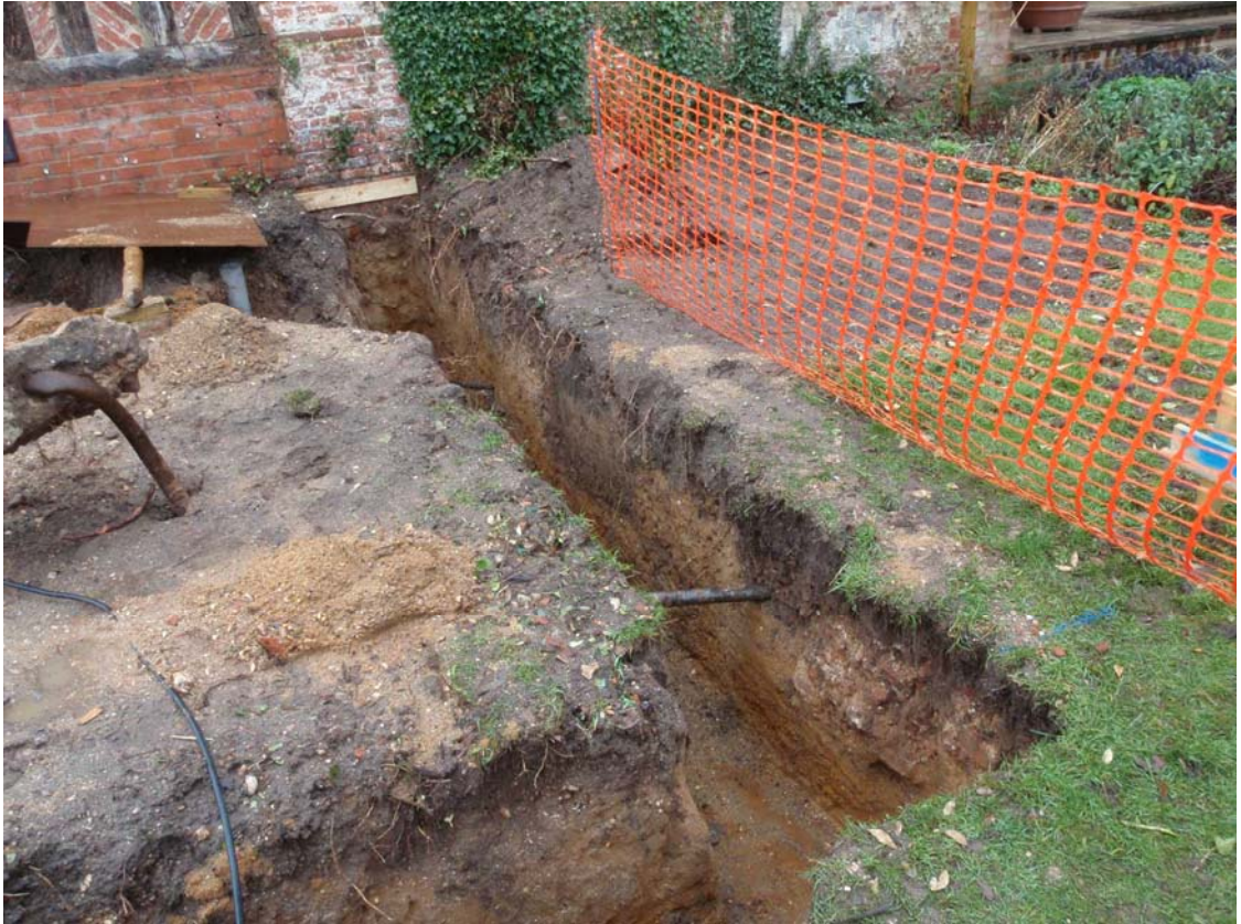
Plate 3. View of the trench recorded as Section S1, looking northeast (1m scale)
