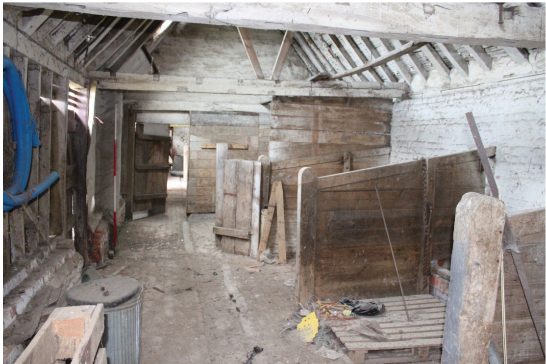
Illus. 6. Interior from south of southern cow-shed (4) of Barn 1 showing 19 th century boarded stalls to right and door to northern shed (3) in rear. Note the brick floor with axial drain and yard elevation of boarded studwork to left (replacing an original open arcade).
