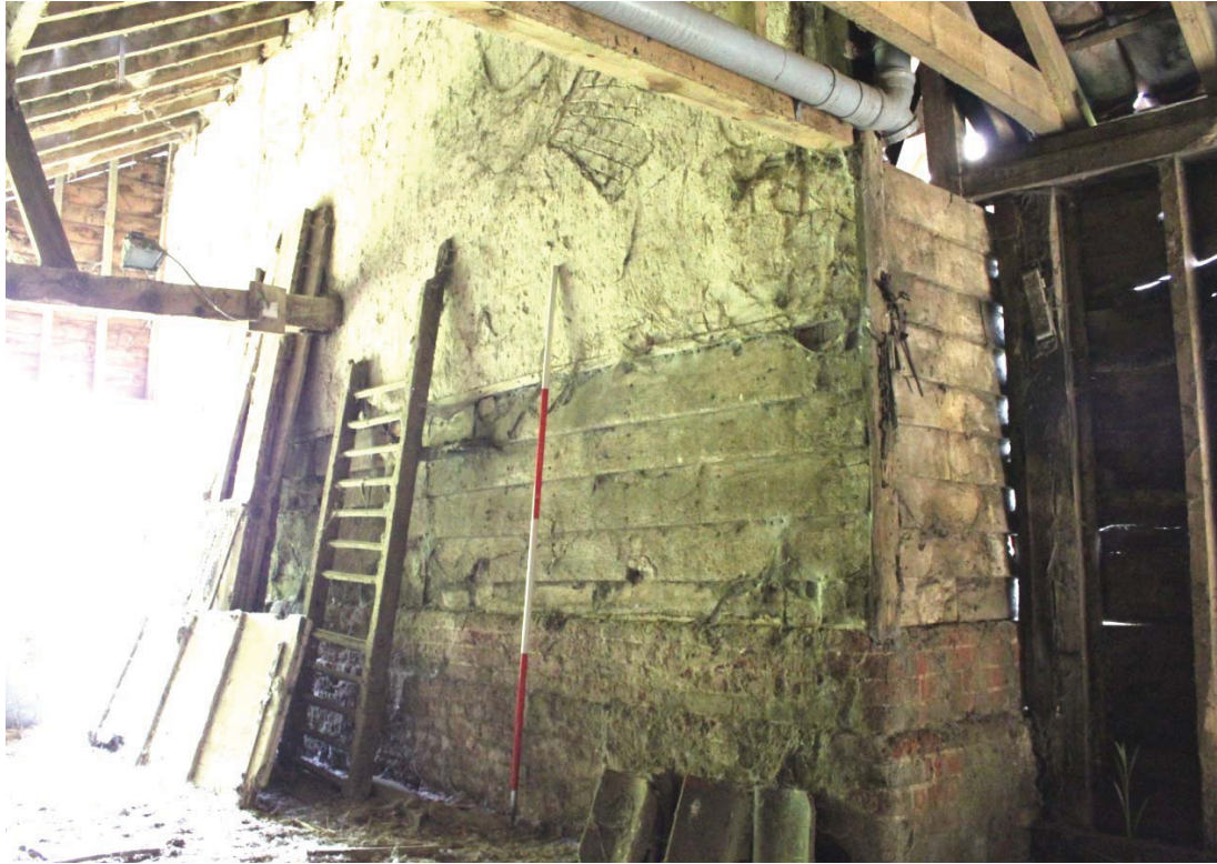
Illus. 11. Northern external gable of main barn (1) of Barn 2 seen from adjoining open shed (3a) to north-west, showing the original two-tier cladding of render above weatherboarding.
