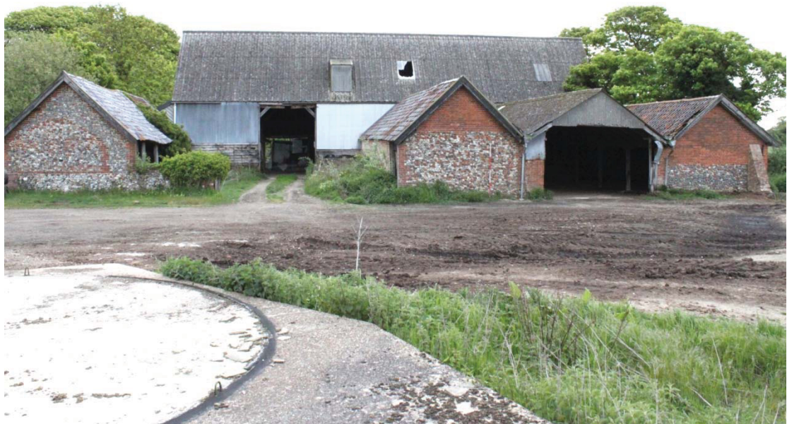
Illus. 10. Western exterior of grade II-listed Barn 2 showing main barn (1) in rear (originally thatched but now with a corrugated asbestos roof) and sheds 3, 4 & 5 from left to right in foreground. The roof over the cattle yard between sheds 4 & 5 to the right is an addition of the mid-20 th century.
