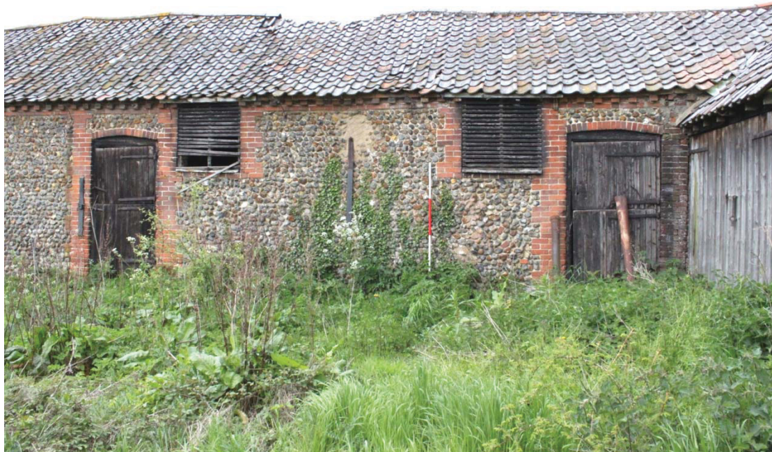
Illus. 7. The original double-hung doors and louvered windows in the eastern exterior of the northern stable (9) which was originally divided in two. The secondary doors of the main barn (1) of Barn 1 are shown to the right.
