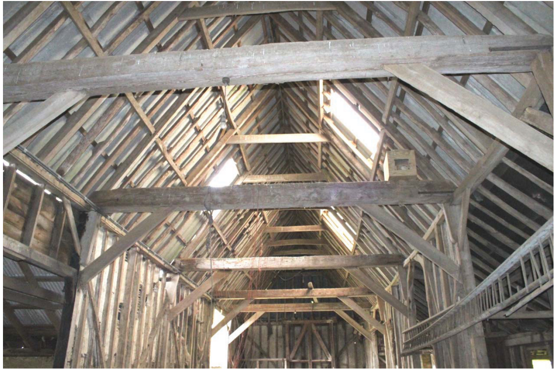
Illus. 13. Detail from south of roof of main barn (1) of Barn 2 showing intact horizontal tie-beams and braces with two tiers of linear butt-purlins above. The roof is steeply pitched for thatch.
