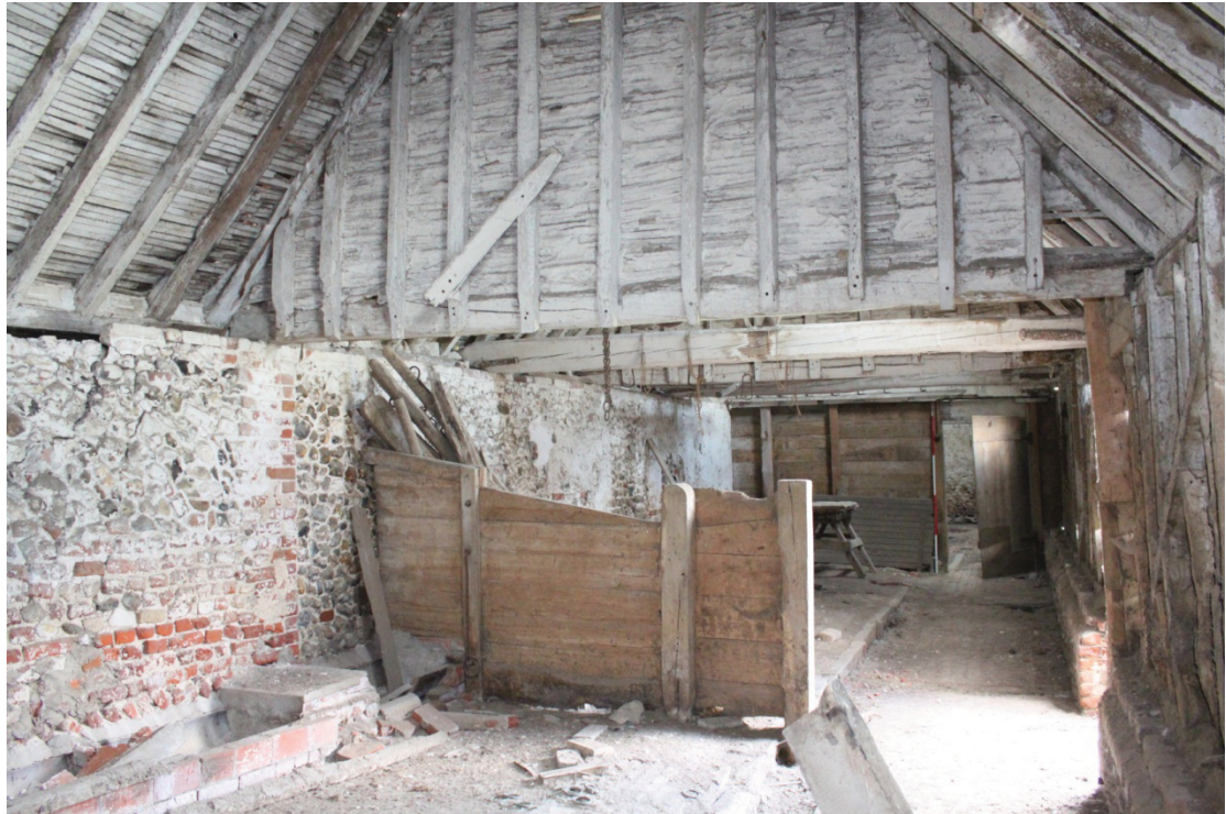
Illus. 5. Interior of northern cow-shed (3) of Barn 1 from north showing low secondary brick manger to left and door to southern shed (4) in rear. The two blocked doors of the eastern elevation are visible to the left, and the two associated lateral partitions still survive above the tie-beams.
