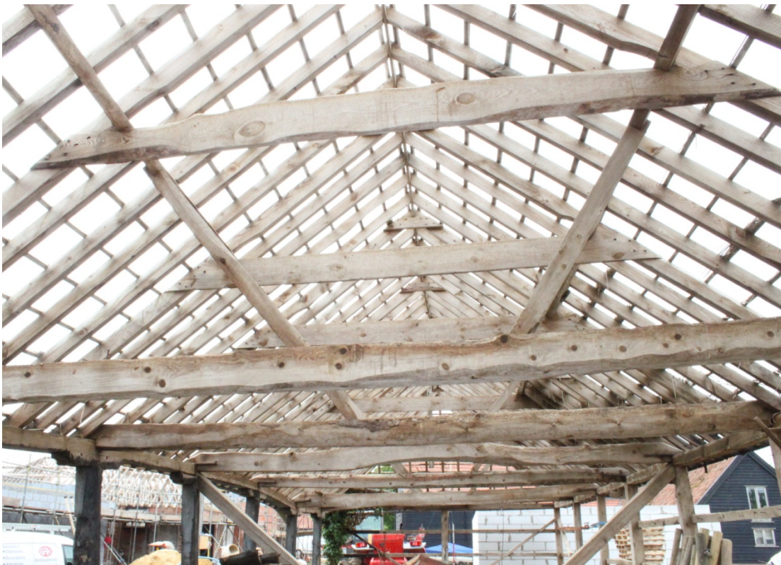
Illus. 10. Internal roof structure seen from north showing clasped-purlins with nailed deal roughwood collars and tie-beams. The tie-beams are secured to the roof-plates with original iron straps.
