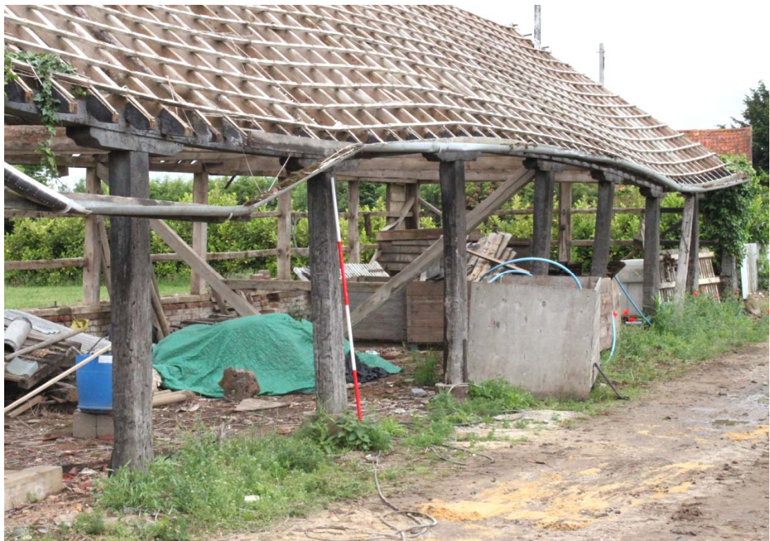
Illus. 6. Open arcade of the eastern elevation seen from south-east showing the undulating roof and the shaped lintels of the arcade posts.
