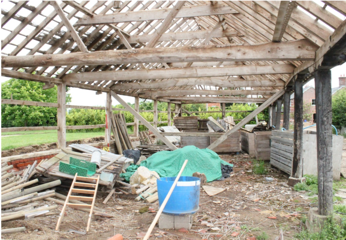
Illus. 9. General view of interior from south showing open arcade to right and enclosed western elevation to left. The diagonal braces are modern insertions.
