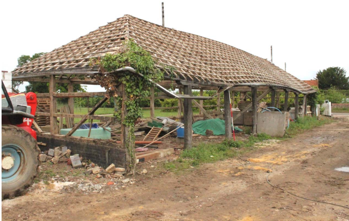
Illus. 4. Exterior of cartshed from south-east showing open eastern elevation and site entrance to right with southern gable to left. The building had been entirely stripped of its external cladding and tiles prior to inspection.
