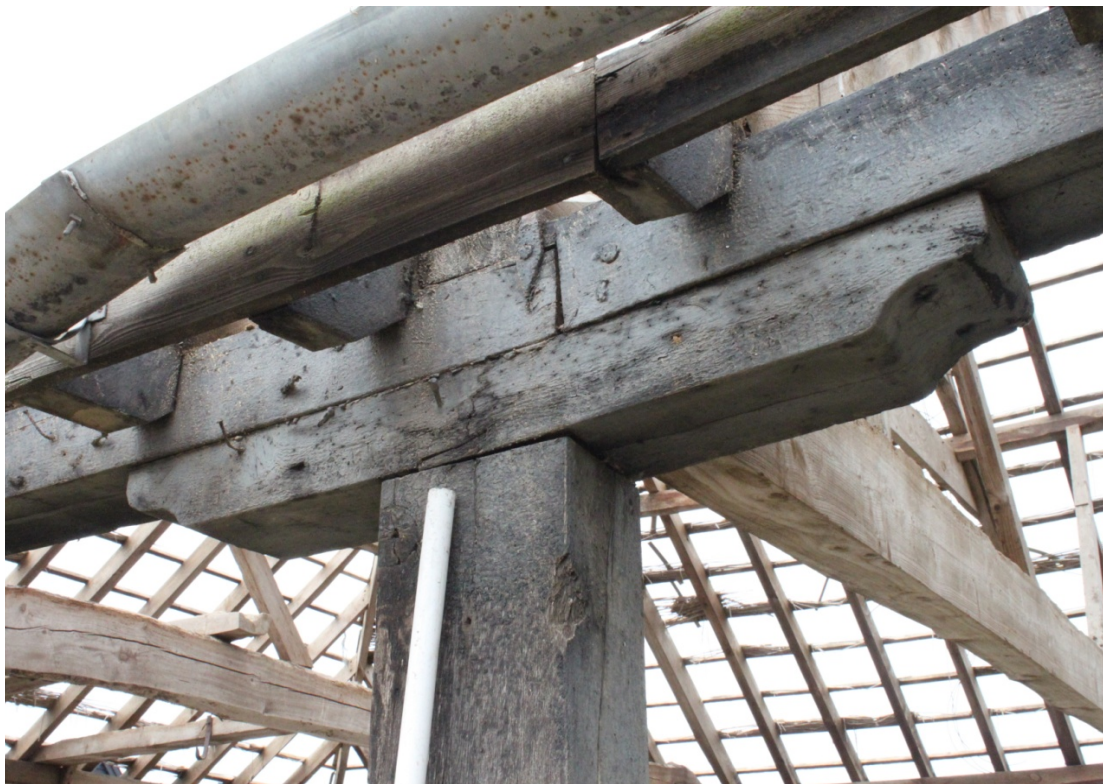
Illus. 8. Detail of shaped lintel to arcade post of eastern exterior showing scarf joint in roof-plate and original grey pigment.
