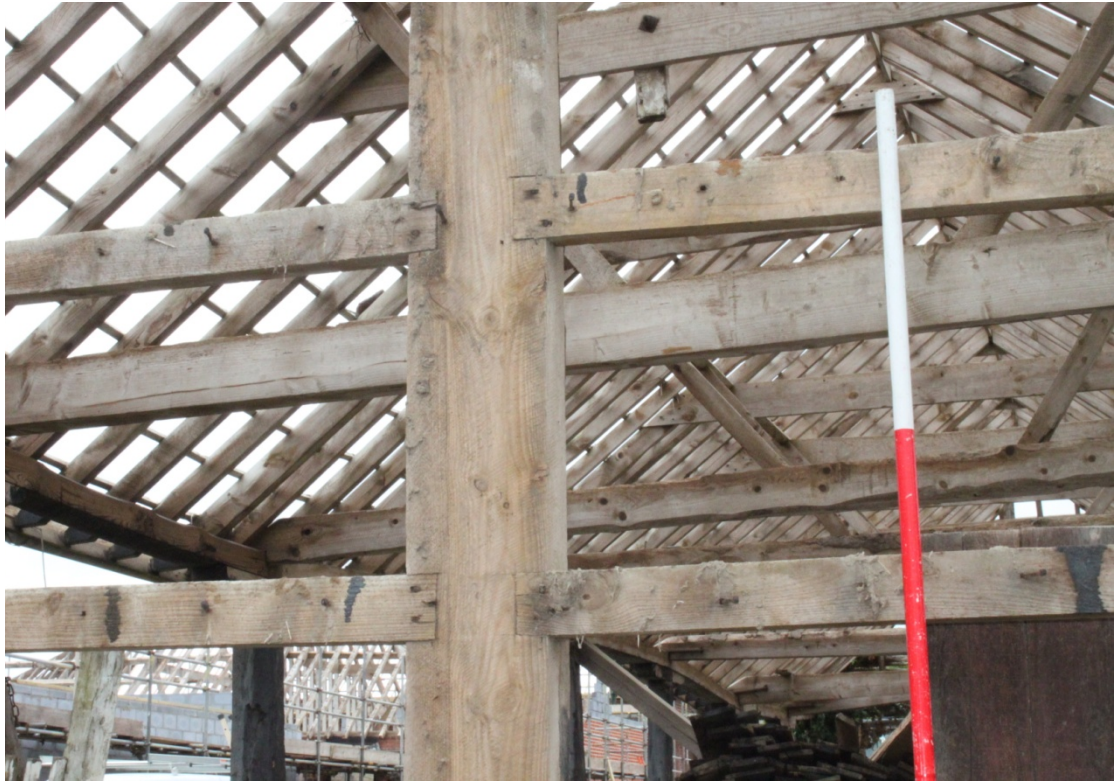
Illus. 7. Construction detail of northern external gable showing softwood horizontal rails nailed to central post.
