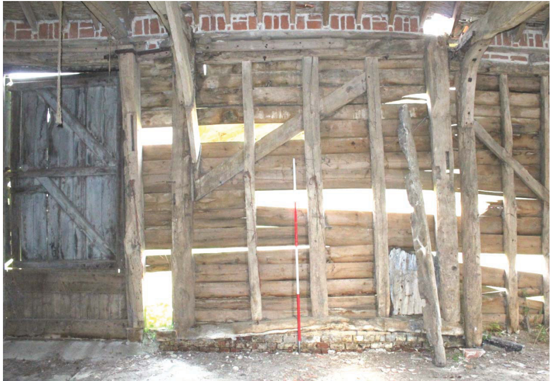
Illus. 9. Northern interior of single 17th century bay (1) showing stud mortises in tie-beam to left with entrance bay of 3-bay barn (2b) beyond.
