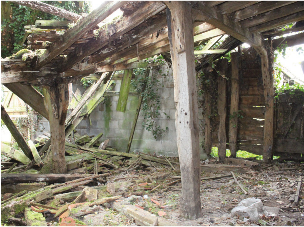
Illus. 13. Interior of collapsed granary (5) from north-west showing the Sampson posts supporting the loft ceiling and the rebuilt cement-block walls.
