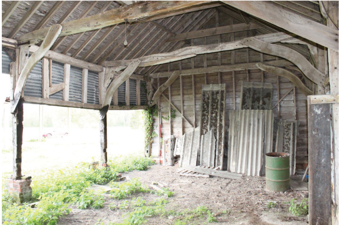
Illus. 5. Interior of the 17th century 3-bay barn (2a) from the west showing the later curved tie-beam braces and the empty mortises of the original western gable in the foreground. The 17 th century studs and wall brace to the left were truncated in the 20 th century to form a vehicle shed.
