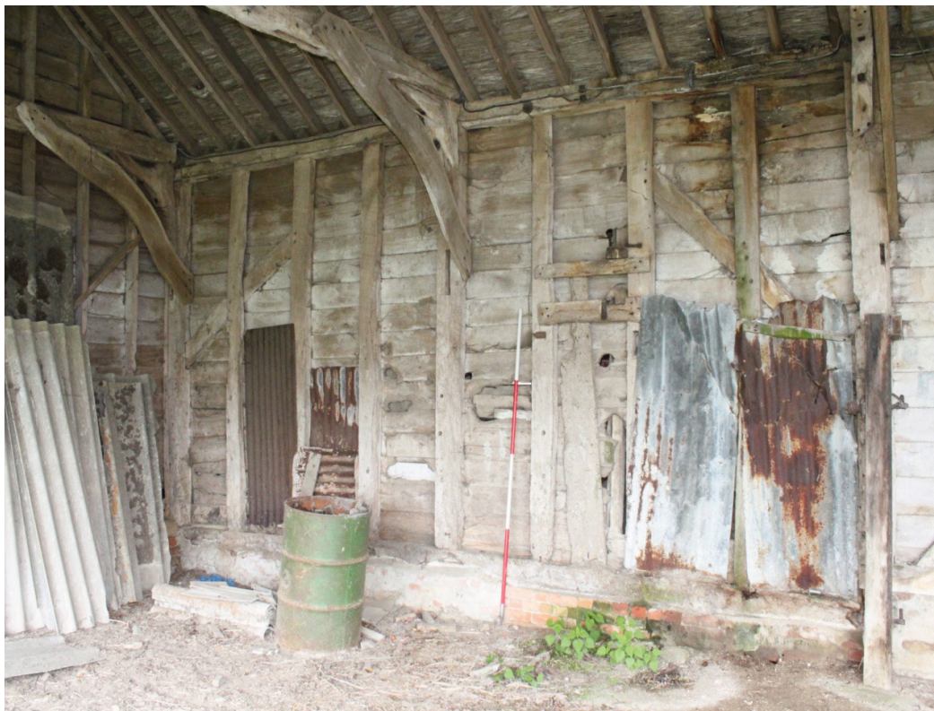
Illus. 6. Internal southern elevation of 17th century barn (2a) showing its externally trenched tension braces with the position of the original western gable to right.
