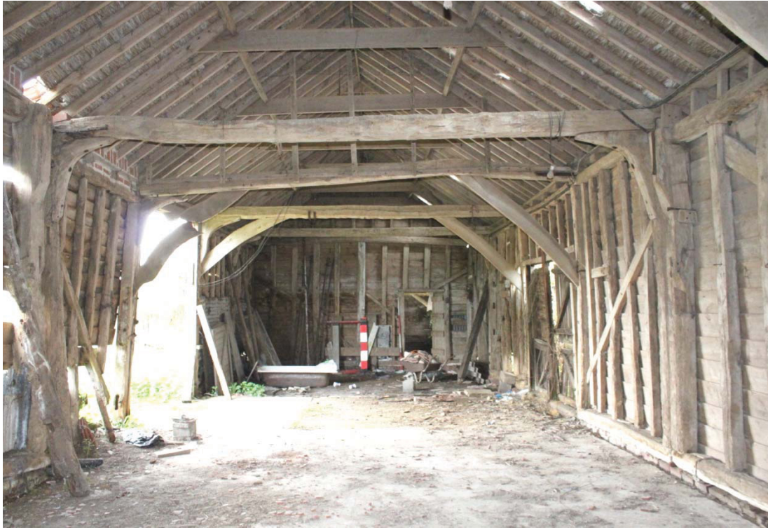
Illus. 7. Interior of main barn from 17th century bays (2b & 1) to west showing original arch-braces to threshing floor of 19th century barn (3) to right and later replacements to left. An original brick threshing floor survives between the two doors.
