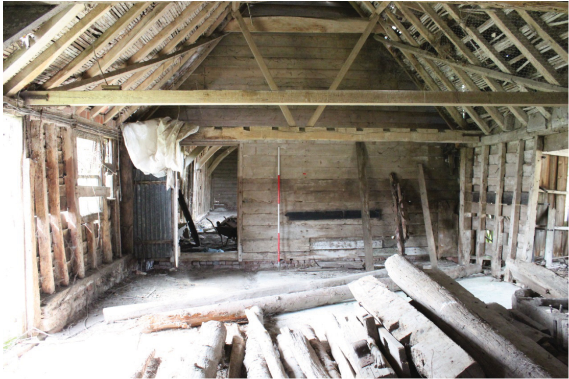
Illus. 11. Interior of stable (4) from east showing door to 19th century barn (3) in rear and notches of missing hay loft in original tie-beams. The roof is original to the early-19 th century structure but the tie-beam in the foreground is an insertion.
