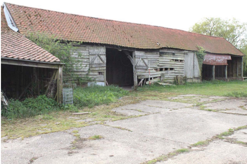
Illus. 4. Northern exterior of multi-phase barn with two entrance bays showing early-19 th century bays to left (3) with early-17 th century structures to right (1 & 2). The western bays have been converted into an open-sided vehicle shelter. The shallow-pitched pantiled roof is a later 19 th century addition.
