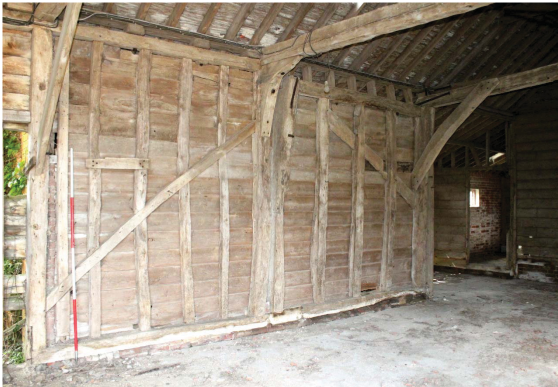
Illus. 10. Southern interior of western bay of 19th century barn (3) showing lowered entrance to left and single 17th century bay (1) to right with rebuilt southern entrance (2b) beyond. Each of the three bays is of a different period.
