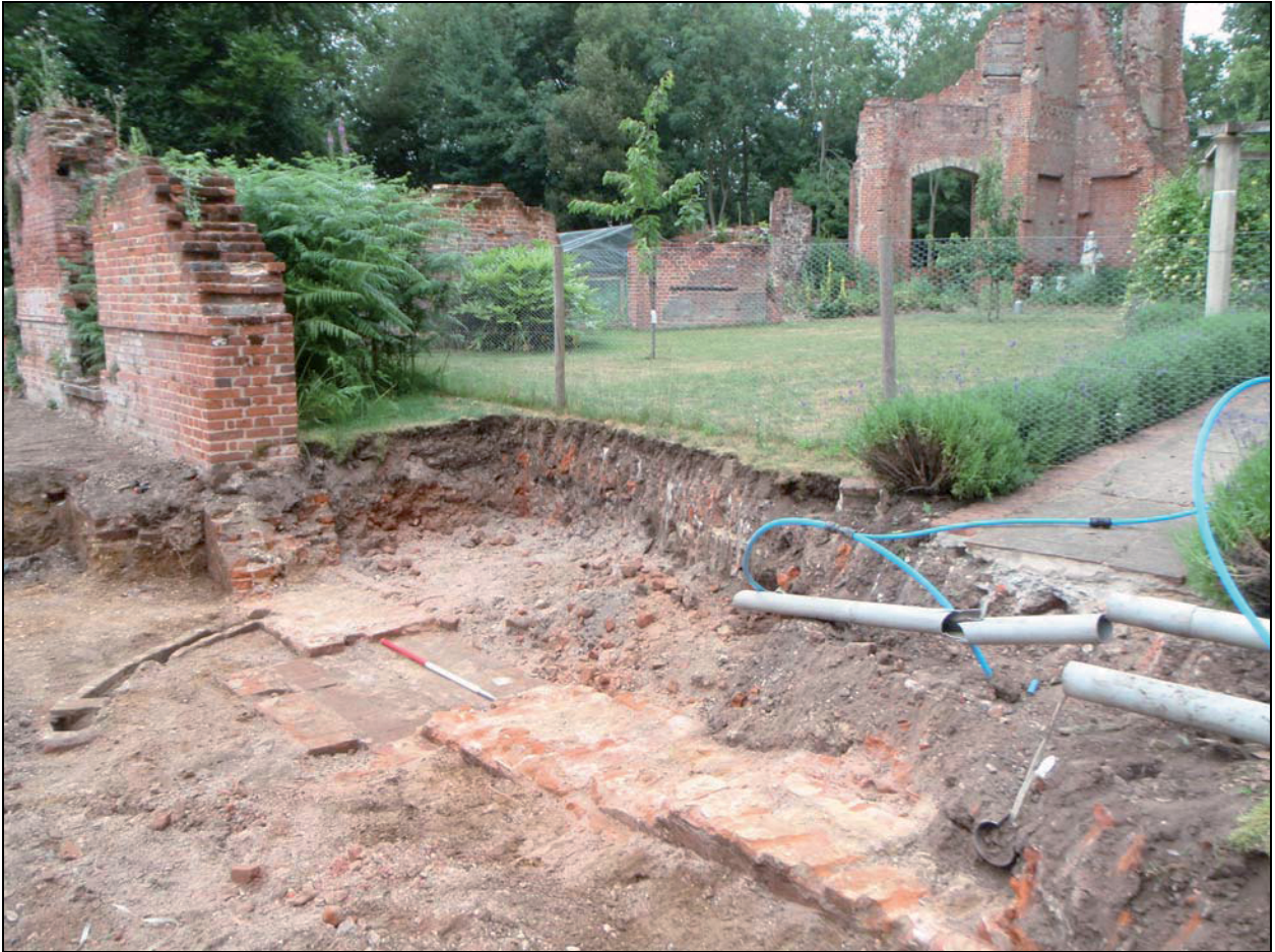
Figure 4. Northwest site corner showing existing walls of Barton Hall and exposed wall foundation
