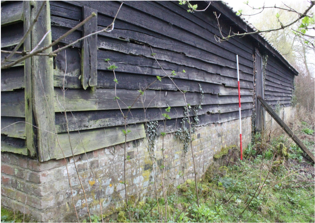
Illus. 9. Eastern exterior showing the rebuilt brick plinth and the external door to the open shed (2b).
