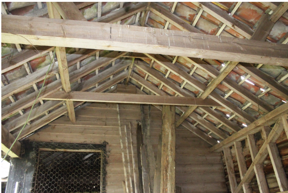
Illus. 6. Softwood roof structure of open shed (2a) from west showing its clasped-purlins with nailed collars & the door and boarded partition to the enclosed shed (2b).
