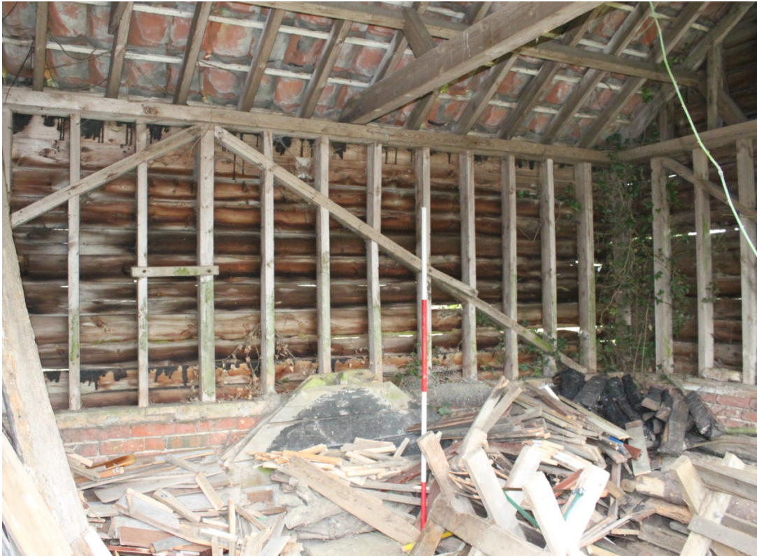
Illus. 7. Southern interior of the western open shelter-shed (2a) showing the diagonal primary stud bracing and brick plinth with the western gable to the right.
