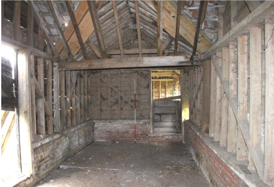
Illus. 10. Interior of enclosed feed store or loose box (2b) from the east showing the external door to the left and the door to the open shed (2a) to right.
