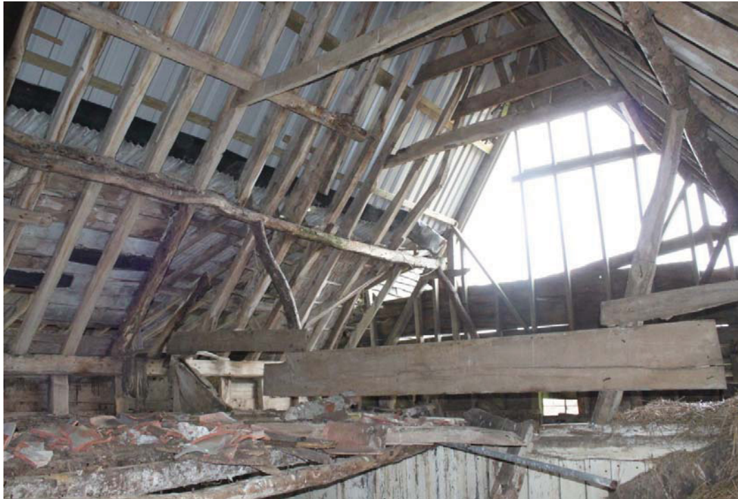
Illus. 11. Clasp purlin roof structure of stable (2) seen from south and showing an inverted bolted knee-brace to a binding joist to left. The rough-wood lower purlin is secondary with the original visible above. The broken pantiles on the loft suggest the original thatch had been replaced before the addition of the present metal sheeting.
