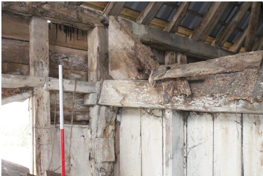
Illus. 12. Detail from north-west of central compartment of stable (2) showing inverted knee-brace to the binding joist of the collapsed hay loft ceiling and the boarded partition to the southern compartment to right. The ceiling has been raised by 0.25 m as shown by the wooden wedge between the joist and the corbel block on the storey post (and by the scar of an earlier clamp on the adjacent stud to left).
