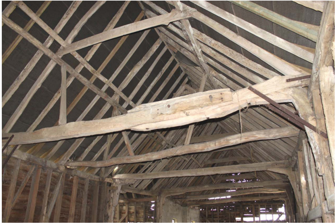
Illus. 5. Roof structure of barn (1) from west showing clasped-purlins of western half with butt-purlins of eastern half in rear. The snapped tie-beam in the foreground was repaired in the 19 th century with bolted wooden plates.
