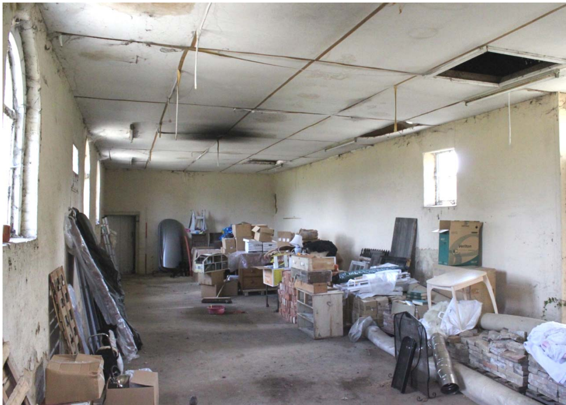
Illus. 6. Interior of coach house (1) from west showing modern ceiling and render. The space has been stripped of its original partitions, fixtures and fittings.
