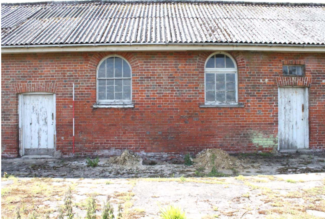
Illus. 5. Detail of original arched windows and doors at southern end of northern facade.
