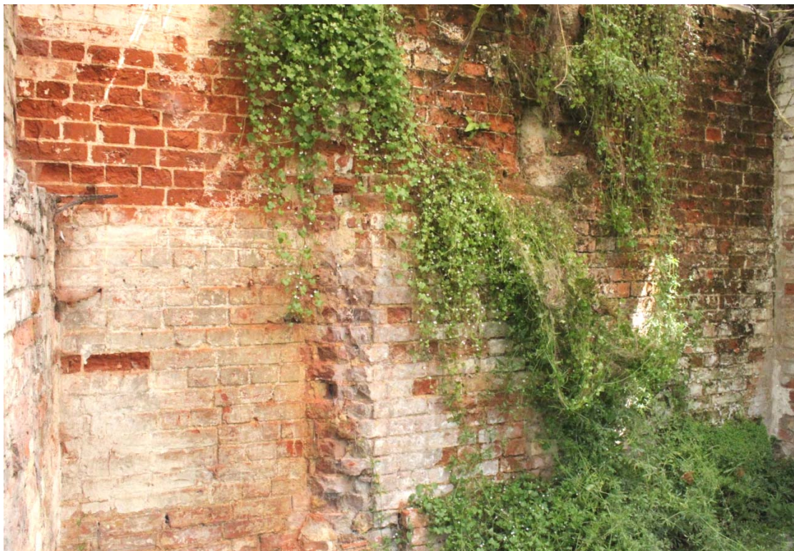
Illus. 10. Northern interior of central section of conservatory (5b) showing scar of demolished original projection from coach house wall.
