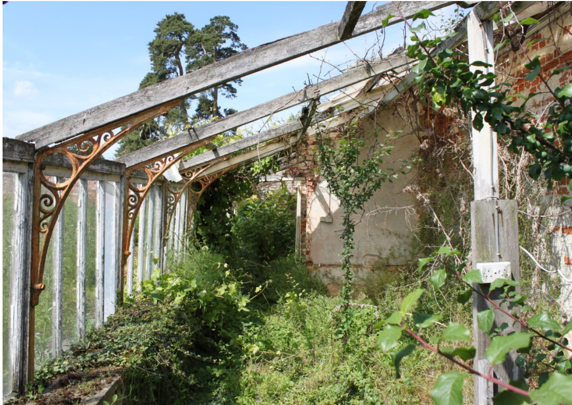
Illus. 9. Interior of conservatory (5c) from east showing doorway to central section (5b) with decorative cast iron brackets to left.
