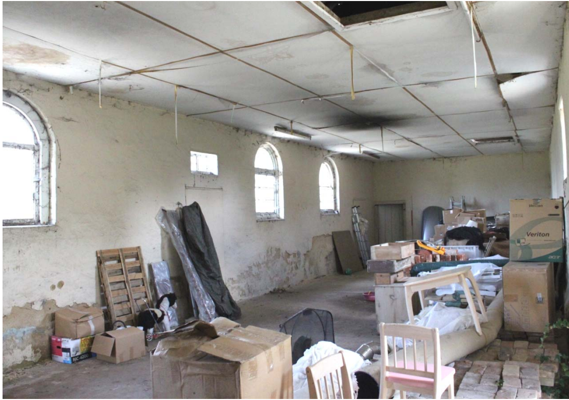
Illus. 7. Interior of coach house (1) from west showing blocked doors of northern facade to left.
