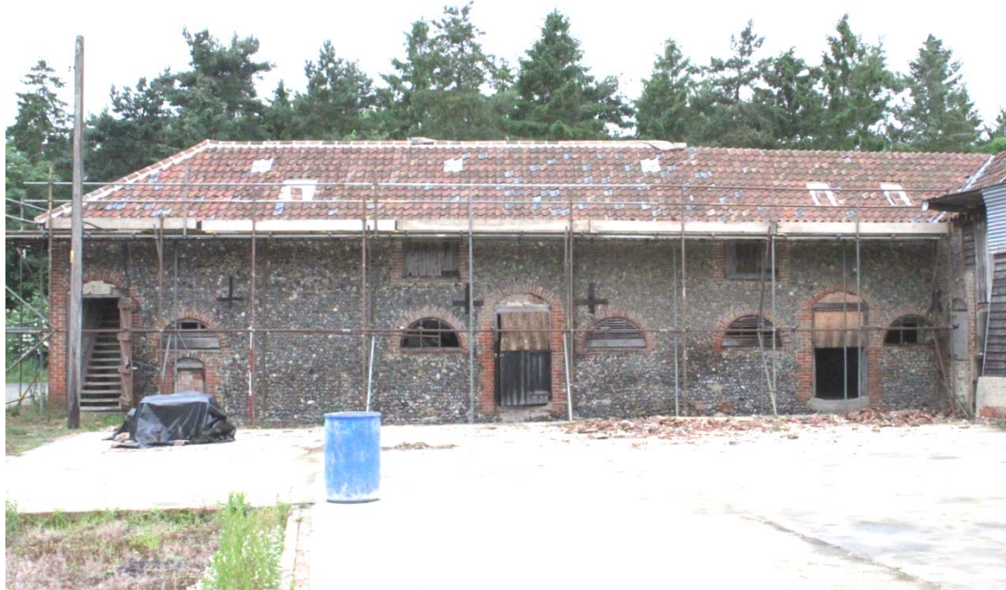
Illus. 2. Eastern exterior of granary (1) showing its symmetrical arrangement with arched doors and windows dressed in red brick. The tall stair door lies to the left and the each stable entered by a central door flanked by windows on each side.
