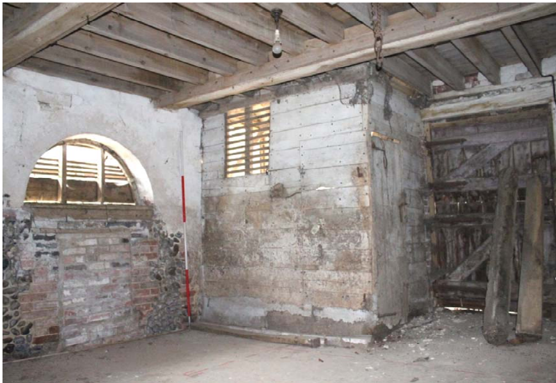
Illus. 8. Boxed stair in south-eastern interior of southern stable (1a) with pintles for the door of demolished box in the foreground that would have been served by the secondary hatch beneath the window to the left (now blocked again).
