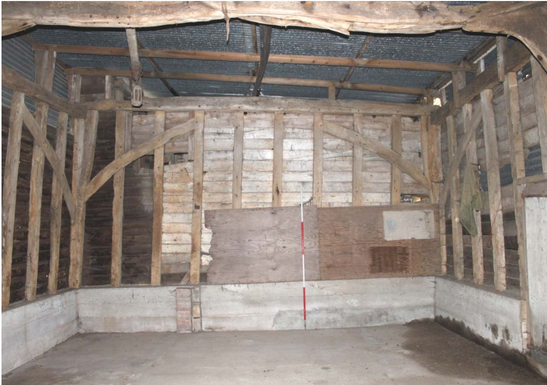
Illus. 13. Internal western gable of barn (4) showing the intact original framing with internally trenced corner braces.
