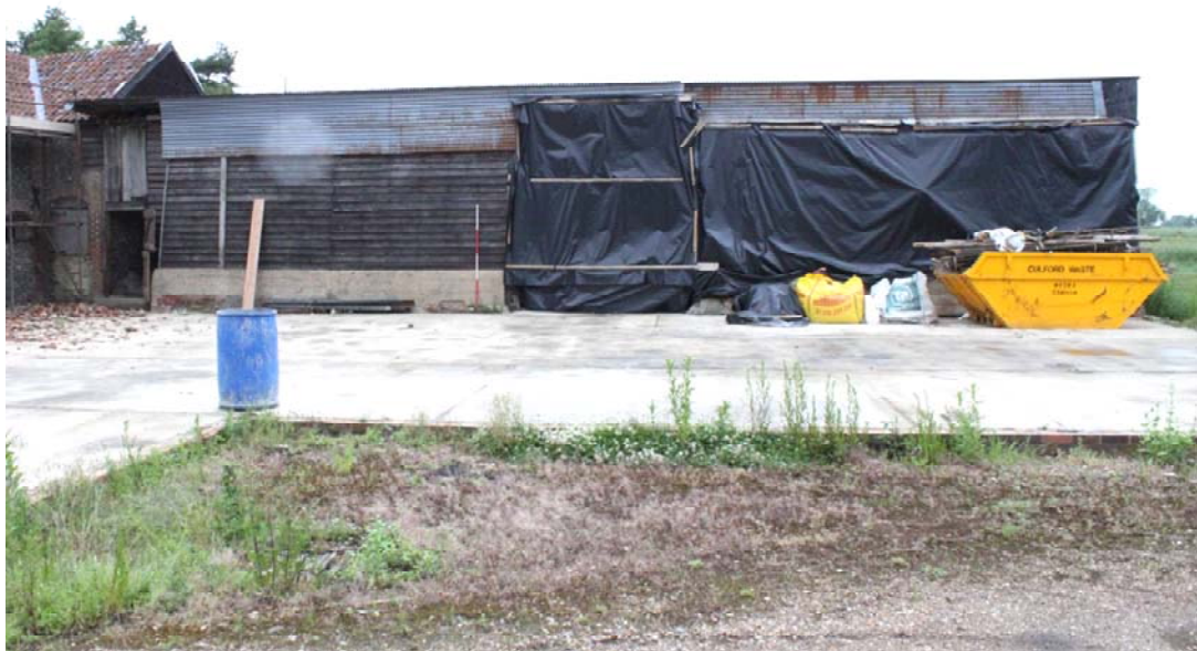
Illus. 4. External southern elevation of the early-17 th century timber-framed barn (4) barely recognisable beneath its 20 th century single-slope roof and showing the granary (1) to left.
