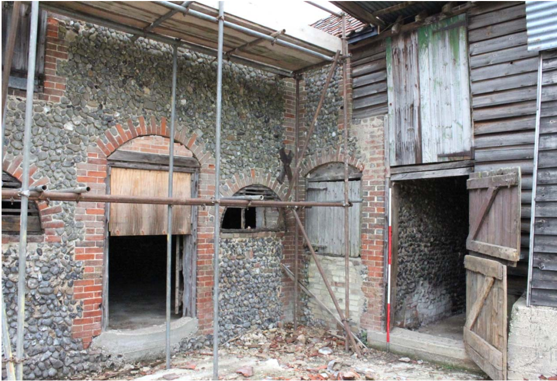
Illus. 3. Junction of granary (1 left) and barn (4 right) from south-east showing the entrance to the northern stable (1c) left, the former hatch to the chaff house (1e) in centre (later converted into a door) and the covered passage between the barn and granary to the right (2).
