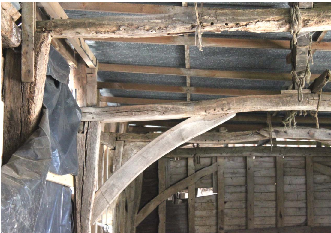
Illus. 14. Detail of original arch brace to west of southern entrance of barn (4) seen from east with empty mortises for a second arch brace in the foreground.
