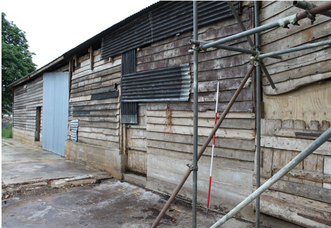
Illus. 5. Northern exterior of barn (4) from the partly demolished brick shed to the north-west showing 18 th or early-19 th century redde (red-ochre pigment) to the boarding of the western bay (right).
