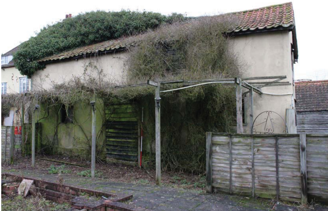
A2.4 External southern elevation of stable (1) showing modern render with original central door flanked by ground-floor windows to right and left. The left window (obscured by vegetation) is also original.
