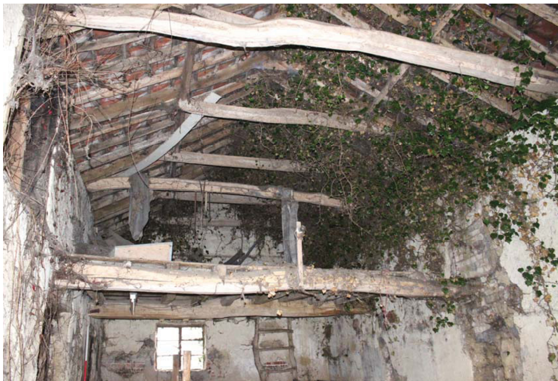
A2.6 Stable interior from east showing original roof structure and remains of original hay loft to west (joists removed from foreground). The window in the western gable is a secondary insertion.
