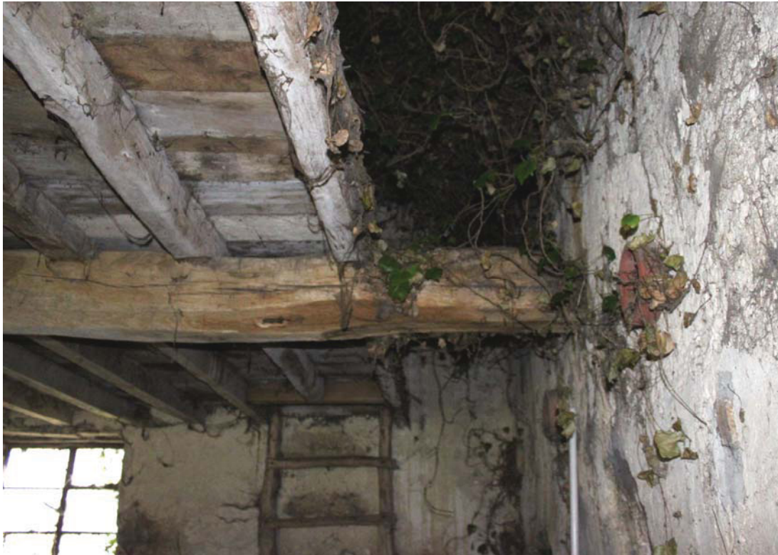
A2.12 Detail of original original loading aperture above former hay rack (seen from east). Note the pipes which penetrate the northern elevation to the right
