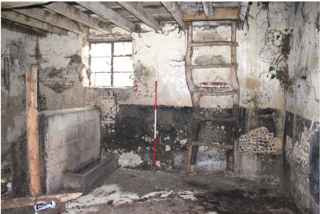
A2.10 Interior of western gable showing loft ladder and inserted window with position of removed hay rack against northern elevation to right. The wall of a 20 th century stall with low feeding trough is visible to left.
