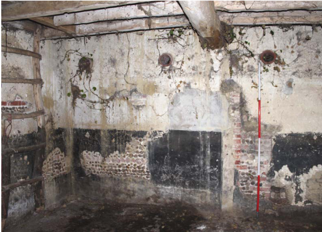
A2.11 Western end of northern internal elevation showing pipes penetrating wall behind position of former hay rack. Note tall flint plinth to left, terminating in brick dressing to right with clay lump fabric beyond. These features were probably retained from an earlier structure on the site.
