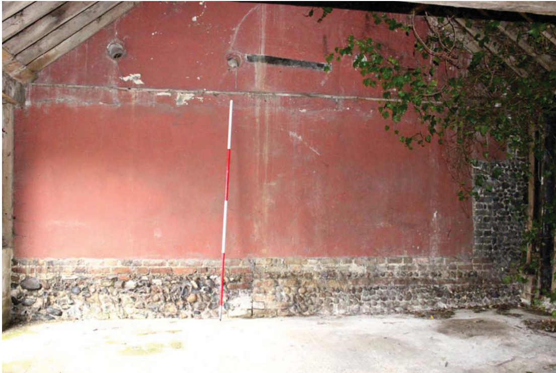
A2.5 Northern exterior of the stable (1) within the later shelter shed (2). Note the change in height of the flint plinth to right, and the abuttal of two corners in the centre. The series of pipes which penetrate the painted clay-lump wall adjoining the internal hay rack is visible above.
