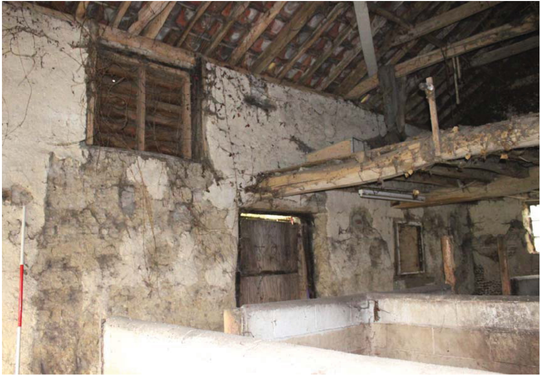
A2.9 Internal southern elevation from north-east showing 20 th century block-work cattle or pig stalls in foreground. Note clay-lump wall fabric. The door and loft window are original features, but the hay loft has been removed to the left.
