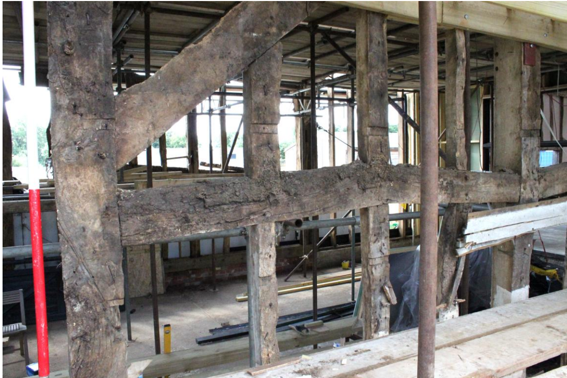
Illus. 9. North-eastern external corner of eastern barn (1) showing wall brace with mid-rail and notches of original daub cladding.
