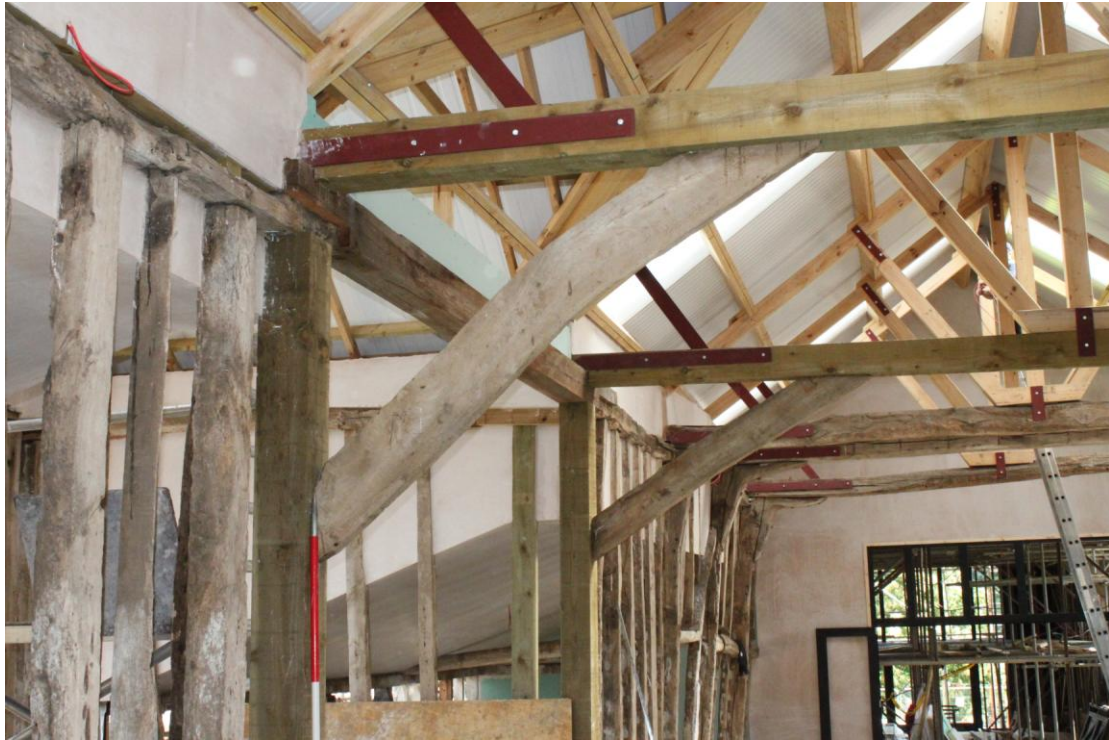
Illus. 7. Detail from west of re-set arch-braces flanking porch (2a) of western barn (2). The tie-beams and storey posts are new softwood timbers, but the arch-braces are understood to have been reinstated in their former positions.
