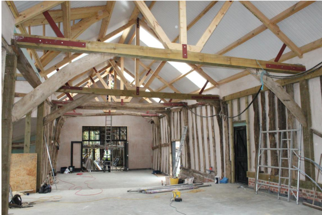
Illus. 5. Western section of barn (2 & 1b) from west, showing partition to eastern section (1 & 4) in rear. The entire roof structure and many principal timbers have been replaced in softwood in recent months.
