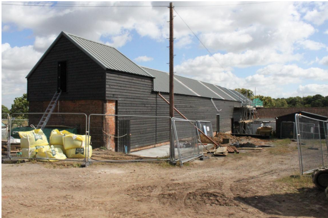
Illus. 4. Exterior from south-west showing modern cladding of ongoing conversion with taller western bay of granary (3) to left.
