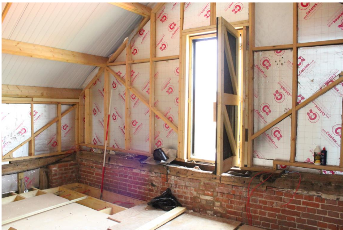
Illus. 10. Internal south-western corner of two-bay first-floor granary (3) showing brick gable with upper walls of new softwood. The original roof-plate is visible to the left but the walls of the western bay have been raised.
