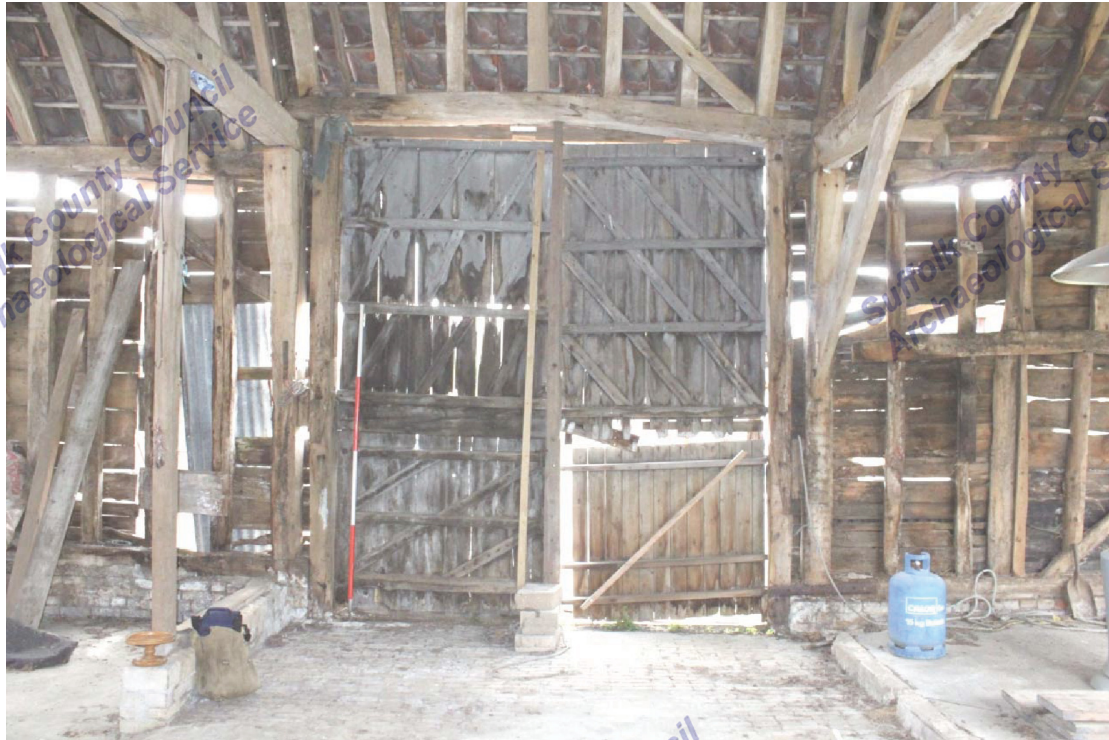
Illus. 11. Southern interior of central bay showing brick threshing floor and grey pigment to barn doors. The original arch-brace to the left-hand tie-beam has been removed and the vertical post is a modern insertion.
