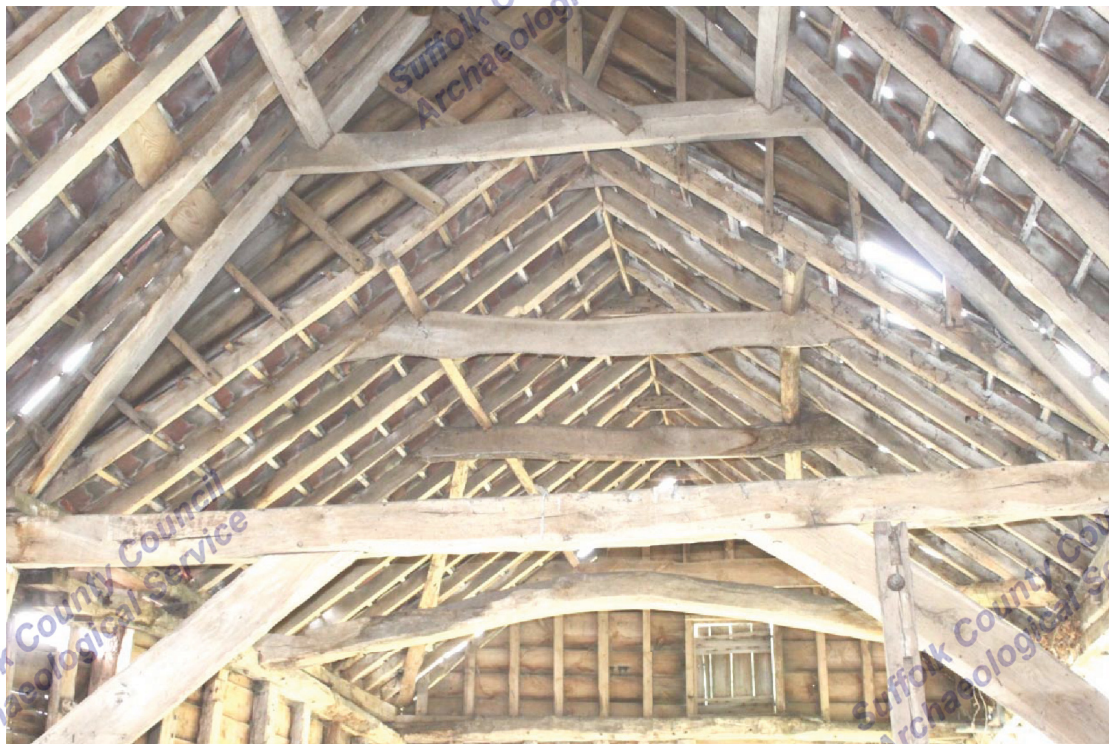
Illus. 8. Roof structure of barn from east showing steeply pitched 17th century roof in foreground and low pitch of 19th century western bays in rear.
