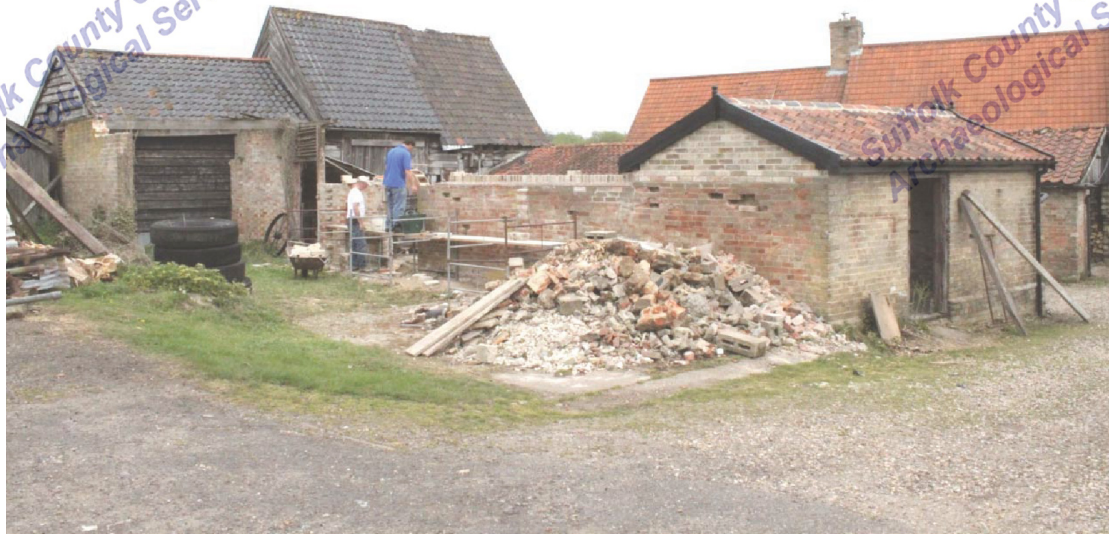
Illus. 3. Exterior of southern yard complex from south-west showing barn in rear to left, brick feed shed (5) to right and site of demolished western range in foreground.
