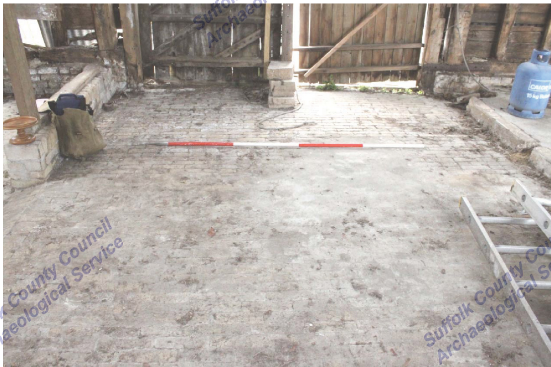
Illus. 12. Gault (white) brick threshing floor to central bay of barn seen from north.
