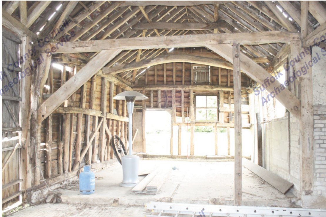
Illus. 7. Interior of barn from east showing rebuilt western end on different alignment with central threshing bay in foreground.
