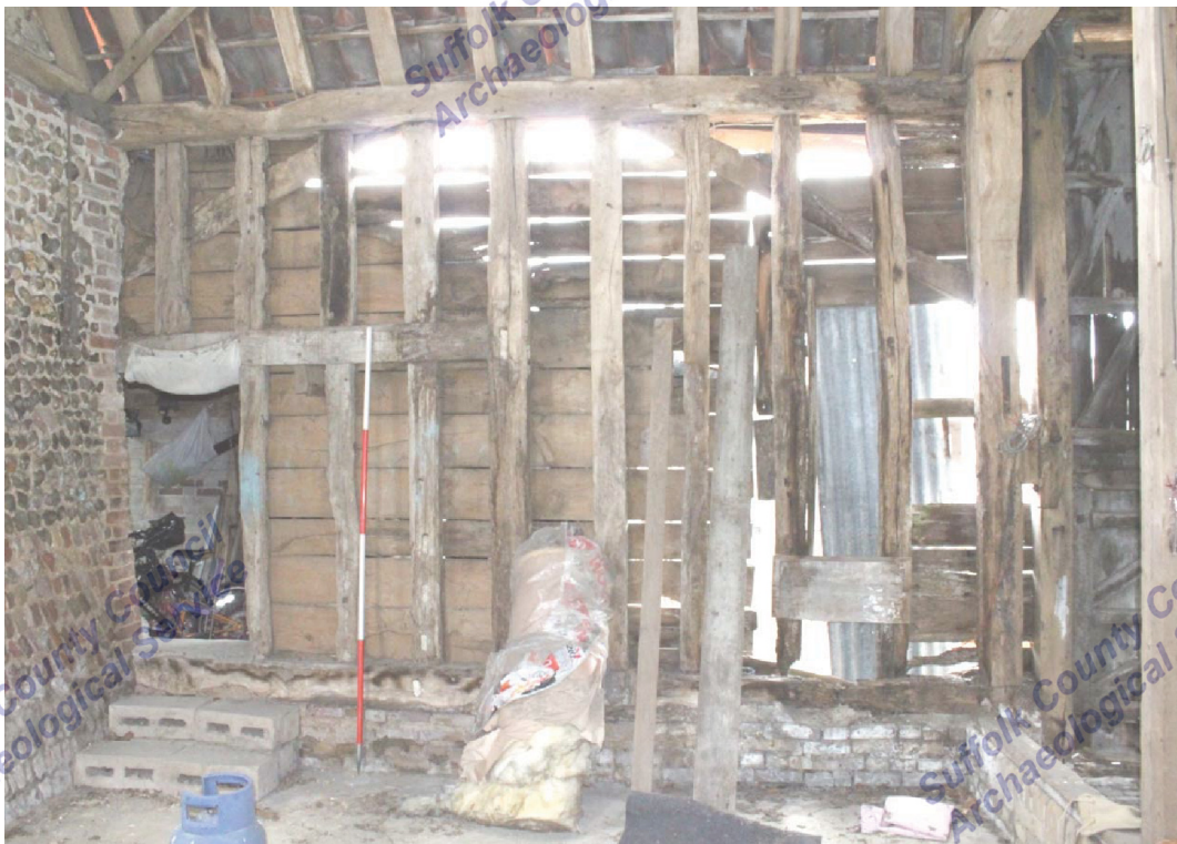
Illus. 10. Southern interior of eastern bay showing re-used timber with unusual partial mid-rail to left and externally trenched wall braces.
