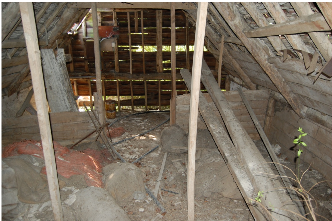
Illus. 10. First floor granary (8 & 9) viewed from the door in the eastern gable showing the staggered butt-purlin roof structure.
