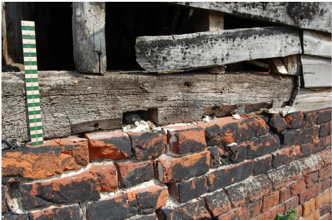
Illus. 4. NW corner sole plate made up of reused wall plate chamfered for rafters. Plinth damaged by impact.
