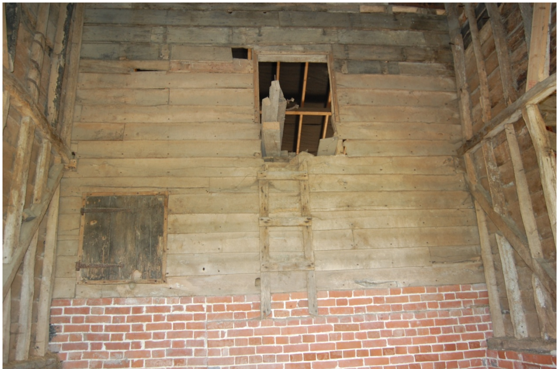
Illus. 8. Hatches connecting the barn and loft to the eastern feed store (4) seen from the feedstore.
