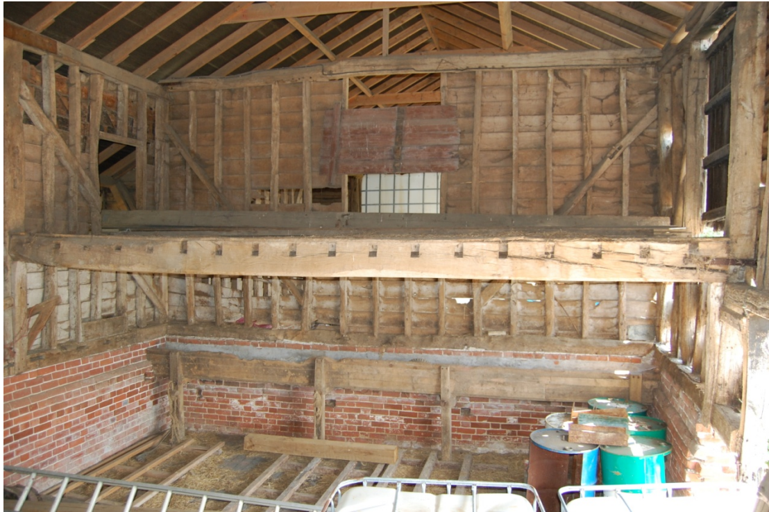
Illus. 5. Loft floor over stable (2) viewed from north, showing empty mortices where the floor has been truncated to the south.
