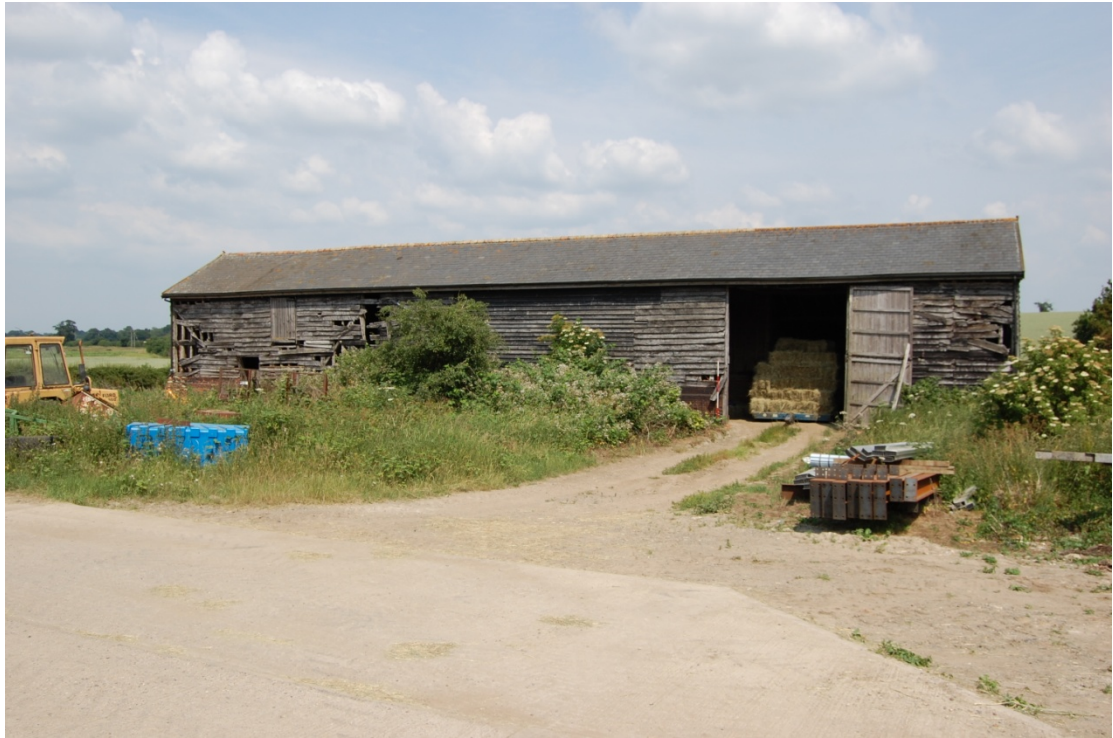
Illus. 1. General view of the barn's external western elevation showing the stable to the left and the twin entrances of the barn to the right
