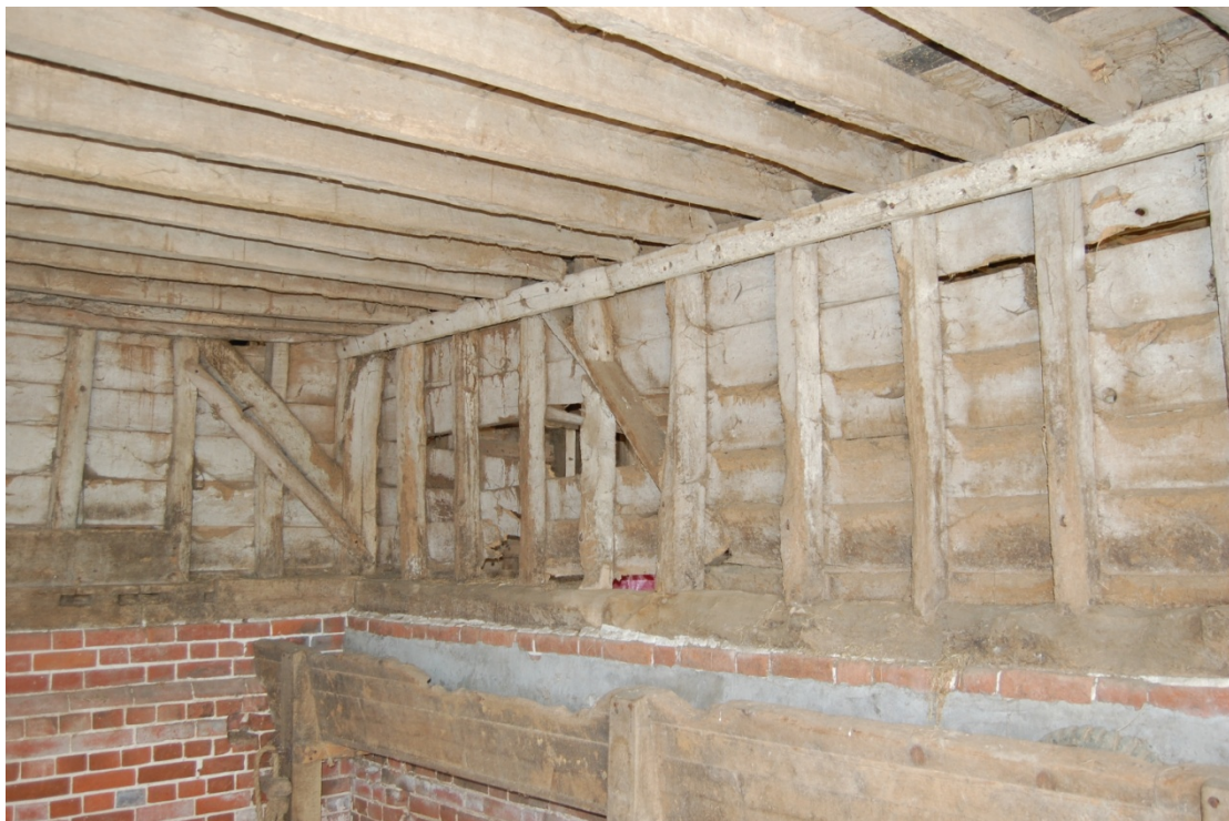
Illus. 6. South-eastern internal corner of stable (2) showing trough against southern interior and end-rail of missing hay rack. The joists of the loft are supported on a clamp nailed to the studs.
