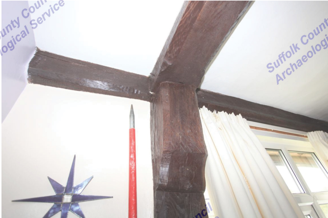
Illus. 7. Detail of finely shaped and chamfered jowl of upper storey post in southern elevation of no. 2 (9). This structure was added to the original house in the mid-17 th century to increase its height.
