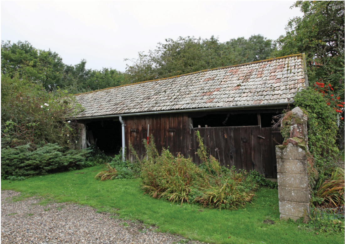
Illus. 3. Southern exterior of shelter-shed (1) from south-east showing 20th century boarded loose boxes to eastern section (1a) and pantiled roof.
