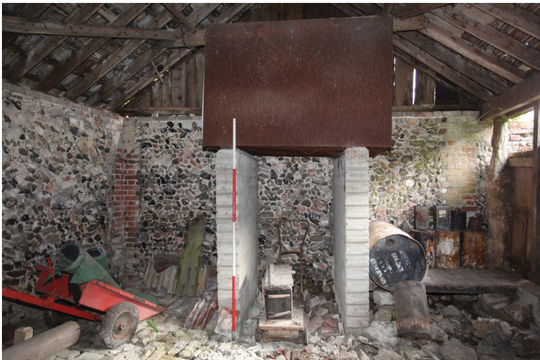
Illus. 6. Internal eastern gable of shelter shed (1a) showing original flint-rubble fabric with brick dressing to corners and contiguity with yard wall to right. The roof structure shown here is also original, with softwood joists and rendered laths against the pantiles.
