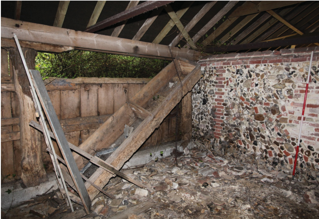
Illus. 7. Detail of boarded cattle trough hanging in south-western internal corner of eastern section of shelter-shed (1a), showing internal partition to right.
