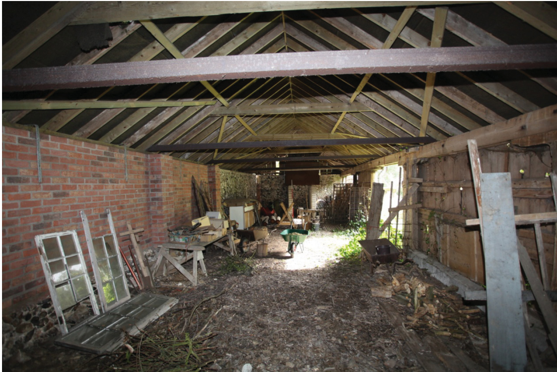
Illus. 5. Interior of eastern section of shelter-shed (1a) showing modern roof and northern brick wall to left (rebuilt after collapse in 1980s) with small section of original flint fabric and roof in rear.
