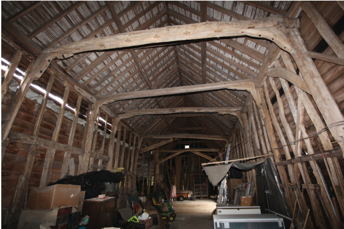
Illus. 9. Interior of barn (3) from east showing arch-braces of formerly open northern elevation to right with fully-framed southern elevation to left & tie-beam with empty stud mortises of original gable above. The roof is a late-19 th century replacement that may be contemporary with the shelter-shed (1).
