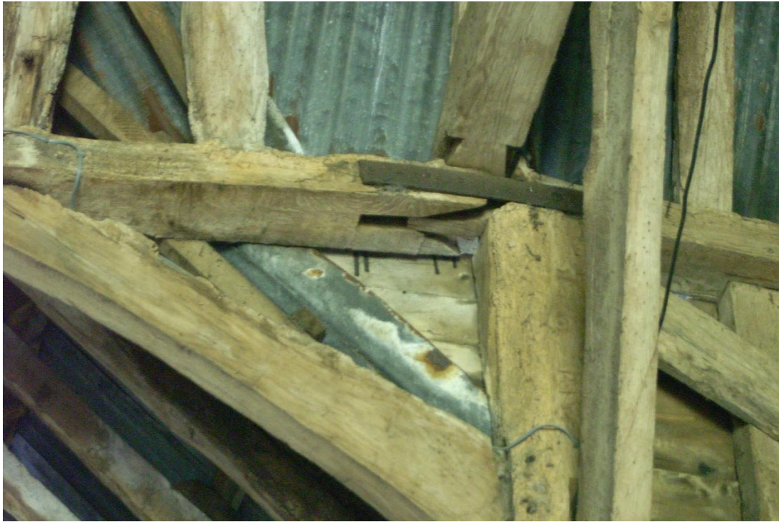
Illus. 9. Barn (1). Detail of an original edge-halved and bridled scarf joint with splayed abutments in the roof-plate adjacent to the western porch. The arch-brace to the roof-plate of the entrance bay (left) is also an original feature.
