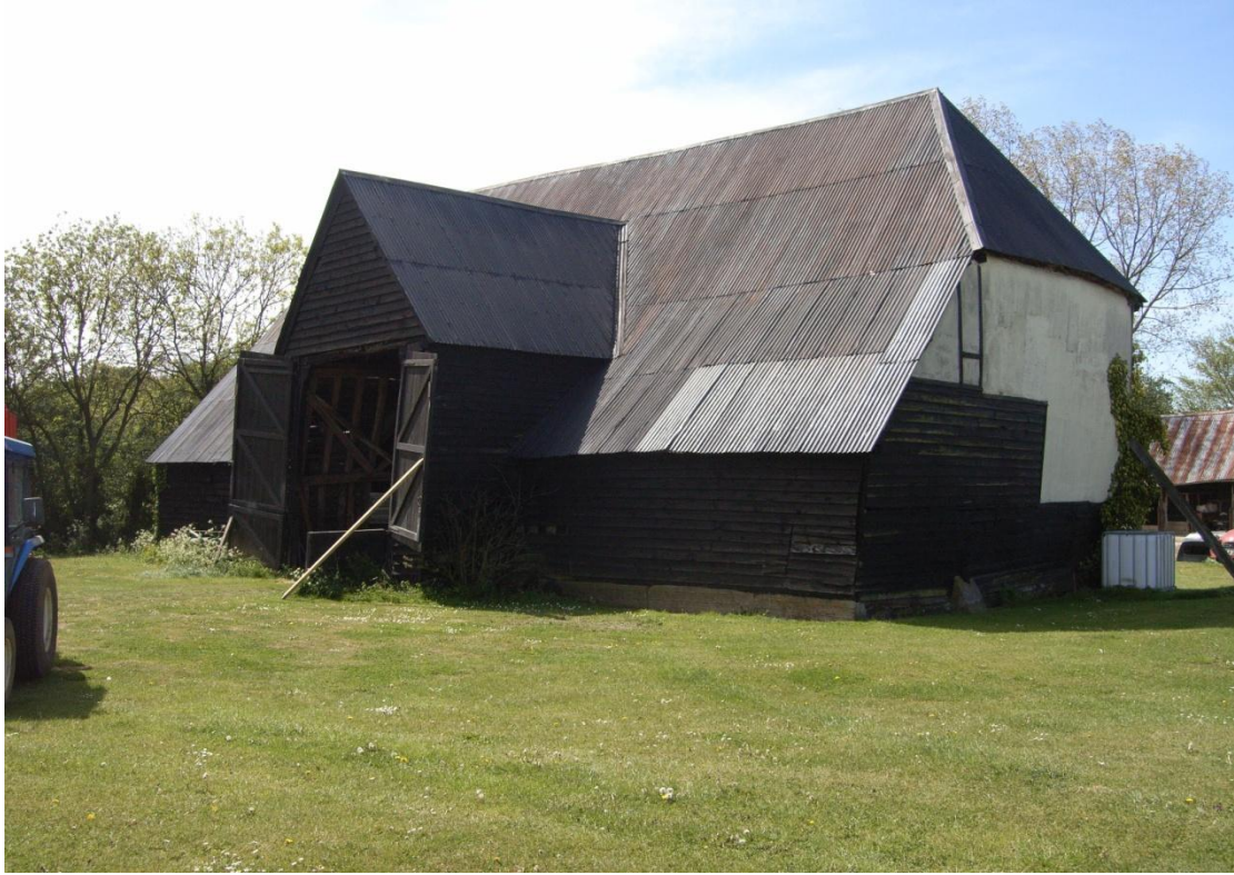
Illus. 3. Exterior of barn (1) from north-east showing secondary aisle and gabled porch with original hipped northern gable (lacking its gablet) to right.
