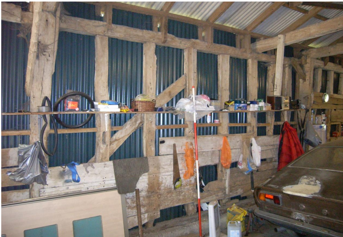
Illus. 18. Stable (2). Northern interior of central bay showing intact studs & eternally trenched brace of the mid-17th century extension, with the original stable's western gable to the right.
