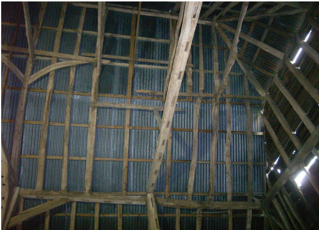
Illus. 10. Barn (1). The southern end of the clasped-purlin roof structure showing the original wind-braces and the tie-beam of the original hipped southern gable with mortises for the framing that was removed when an end-aisle was added in the 17 th century. This end-aisle was later raised to form the additional bay visible to the right.
