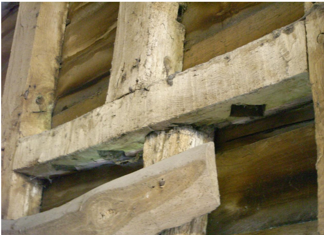
Illus. 14. Stable (2). Detail of diamond-mullion mortises in soffit of window sill in southern interior of eastern bay.
