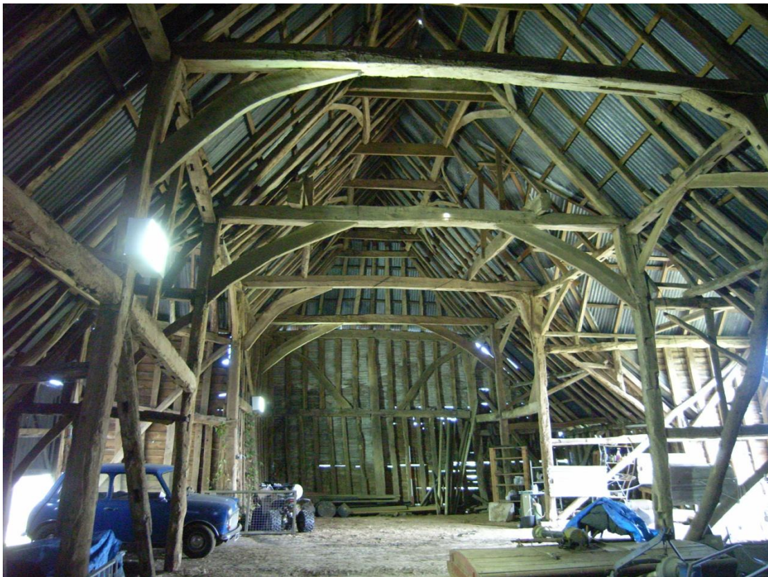
Illus. 6. Barn (1). General view of interior from south showing the original storey-posts, arch-braced tie-beams and clasped-purlin roof with the later aisles to right and left (removing the original wall studs).
