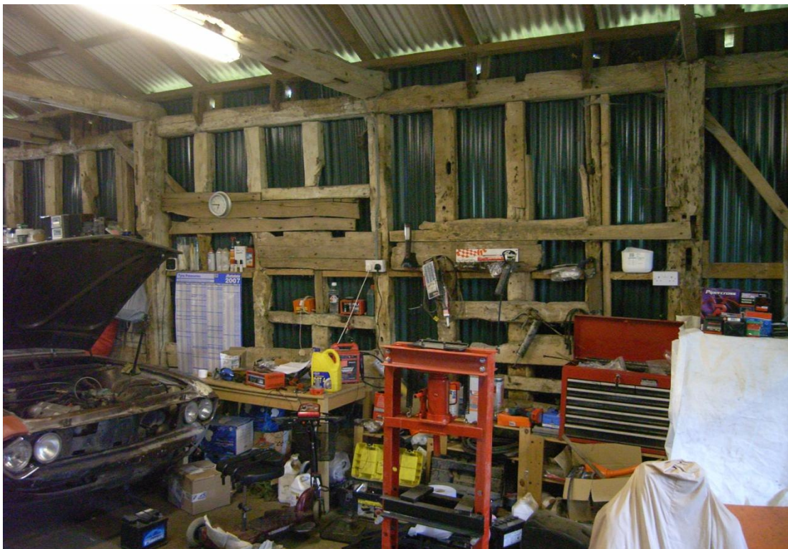
Illus. 16. Stable (2). Northern interior of penultimate eastern bay showing position of original stable entrance to right and original window to left.
