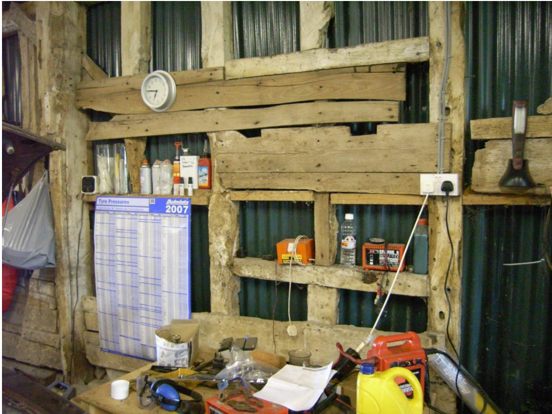
Illus. 17. Stable (1). Detail of the original window lintel and sill in the northern interior of the penultimate eastern bay, partly hidden by 18 th or 19 th century boarding.
