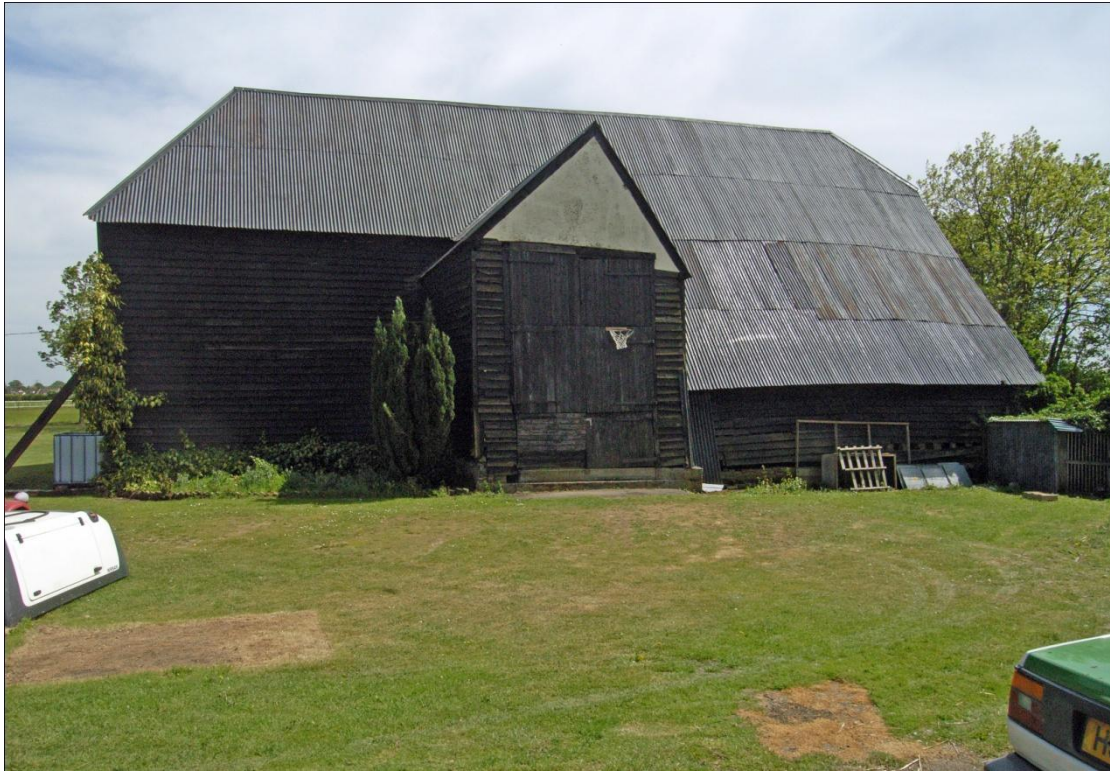
Illus. 5. Western external elevation of barn (1) from the yard showing the original porch and wall height to the left with the later aisle to the right.
