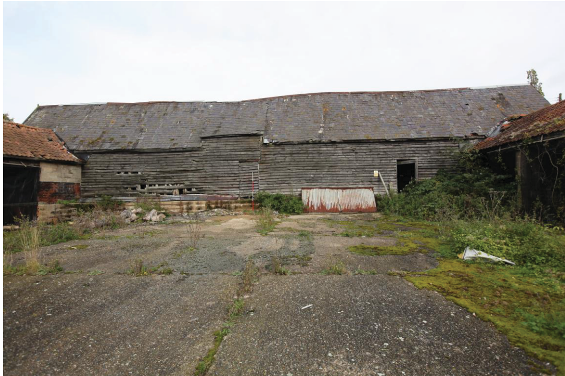
Illus. 3. Southern exterior of barn (1) from yard showing blocked original entrance with raised roof-line in centre & original doorway of later stable (3) to right.
