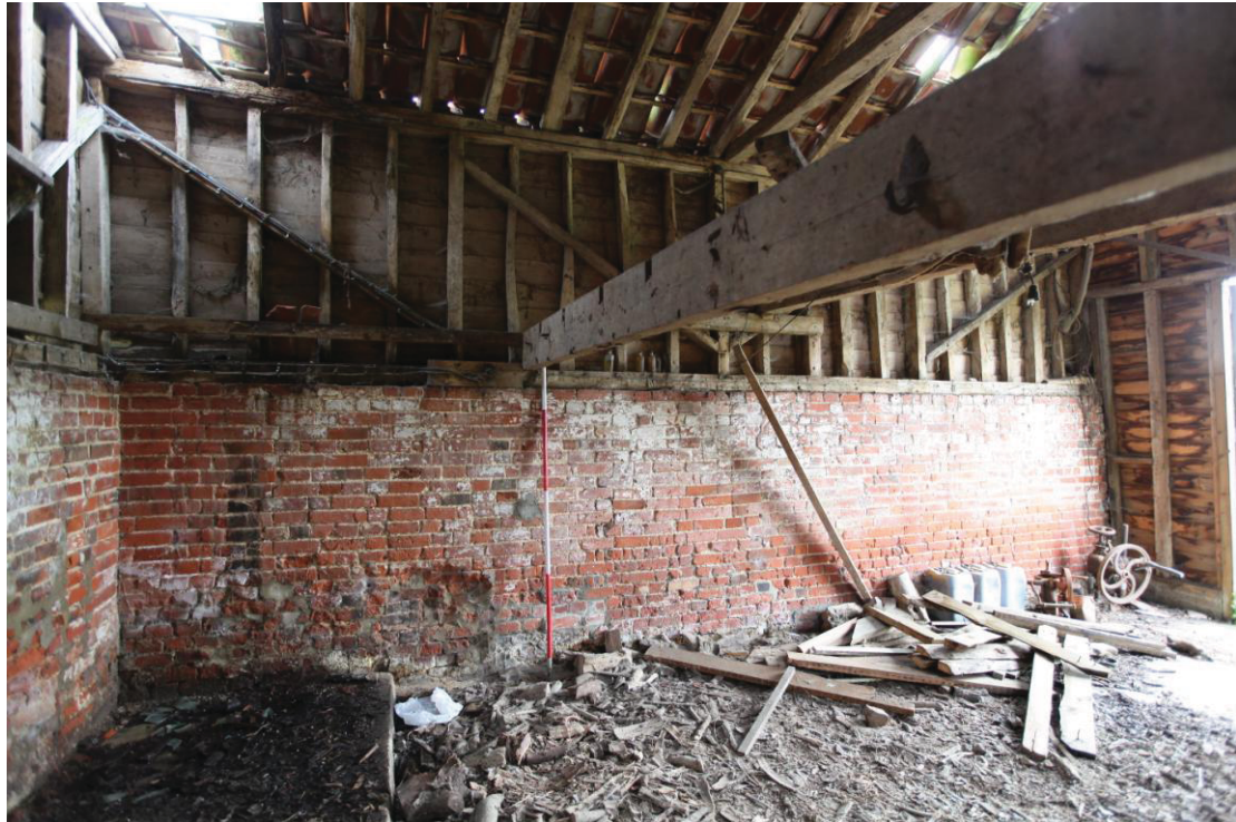
Illus. 11. Eastern interior of enclosed shed (5a) showing binding joist of partial loft (probably for a feed mill or water tank) with rail against studwork and & common joist mortises.
