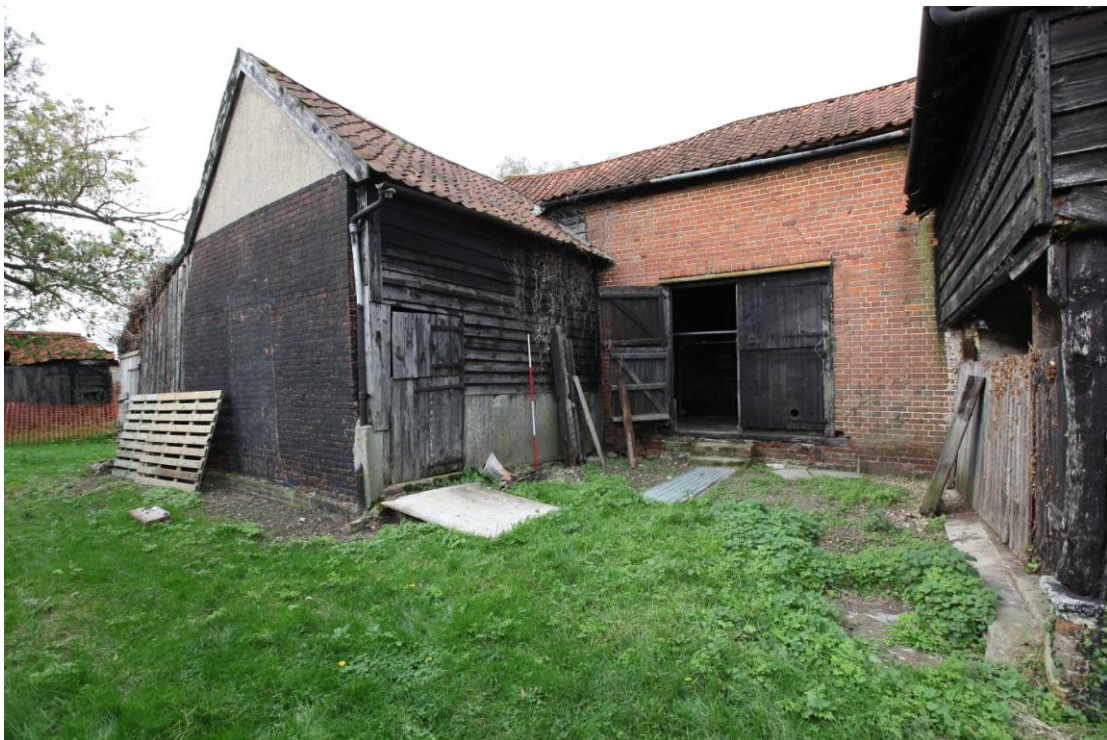
Illus. 4. Exterior from south-east showing the stable wing (2) to the left & the granary wing (3) with its open-sided lower storey to the right. The rear door of the barn lies in the centre and the outline of a blocked stable door can be seen in its brick gable. The detached pig swill shed is visible in the rear to the left.
