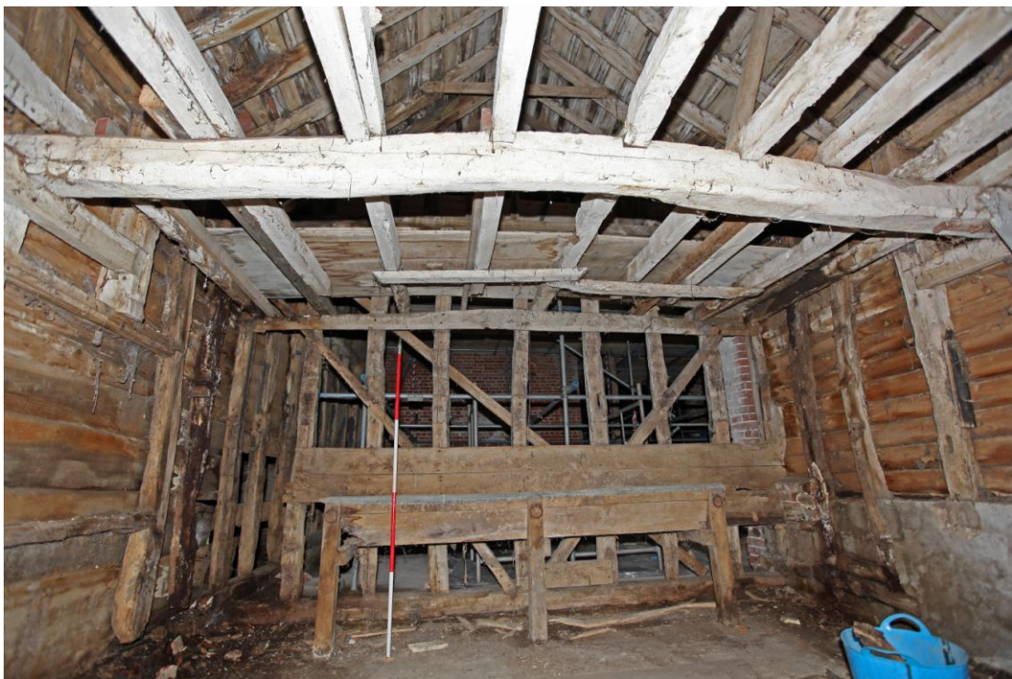
Illus. 10. Northern interior of the stable (2) showing the boarded manger against the barn (1a) and the inserted joists of its hay loft. The framing to right and left is part of a three-bay early-17 th century structure with externally trenched wall braces.
