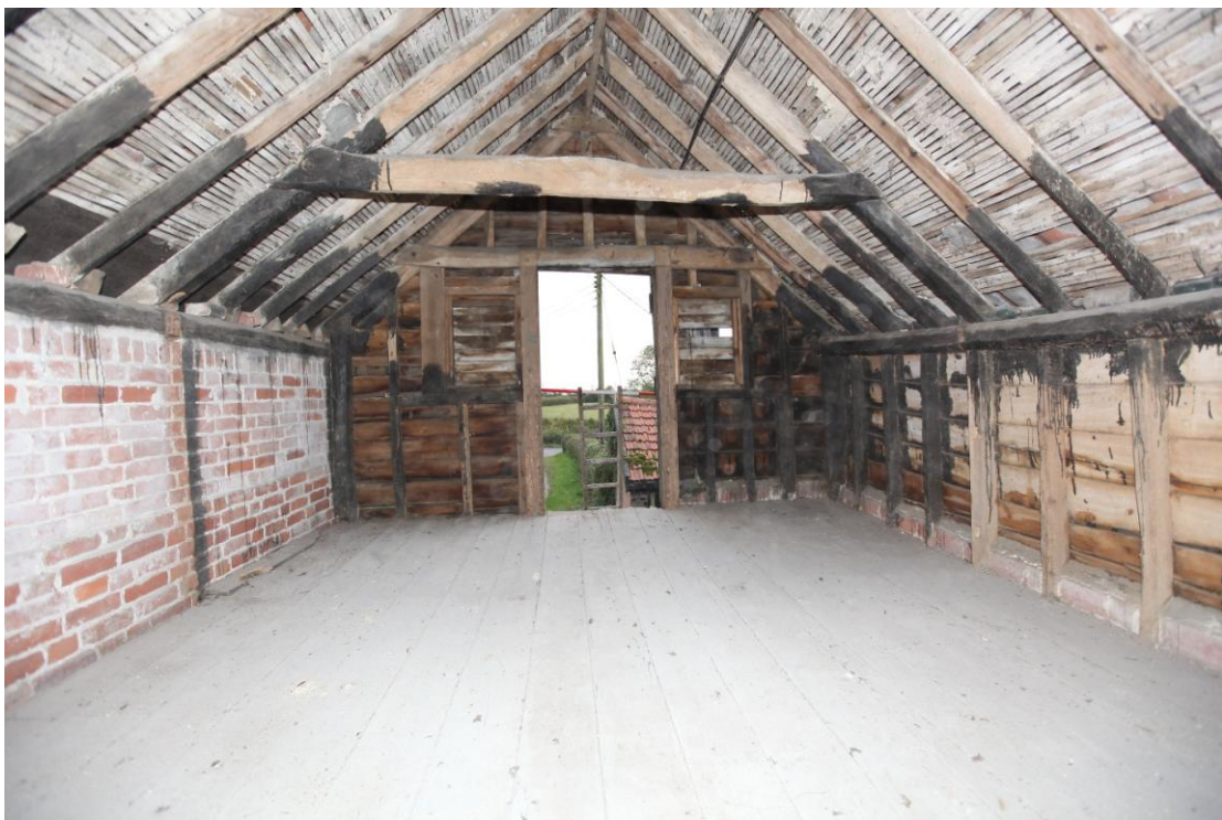
Illus. 12. Interior of the first-floor granary (3) from north showing its entrance door in the southern gable and the original roof structure.
