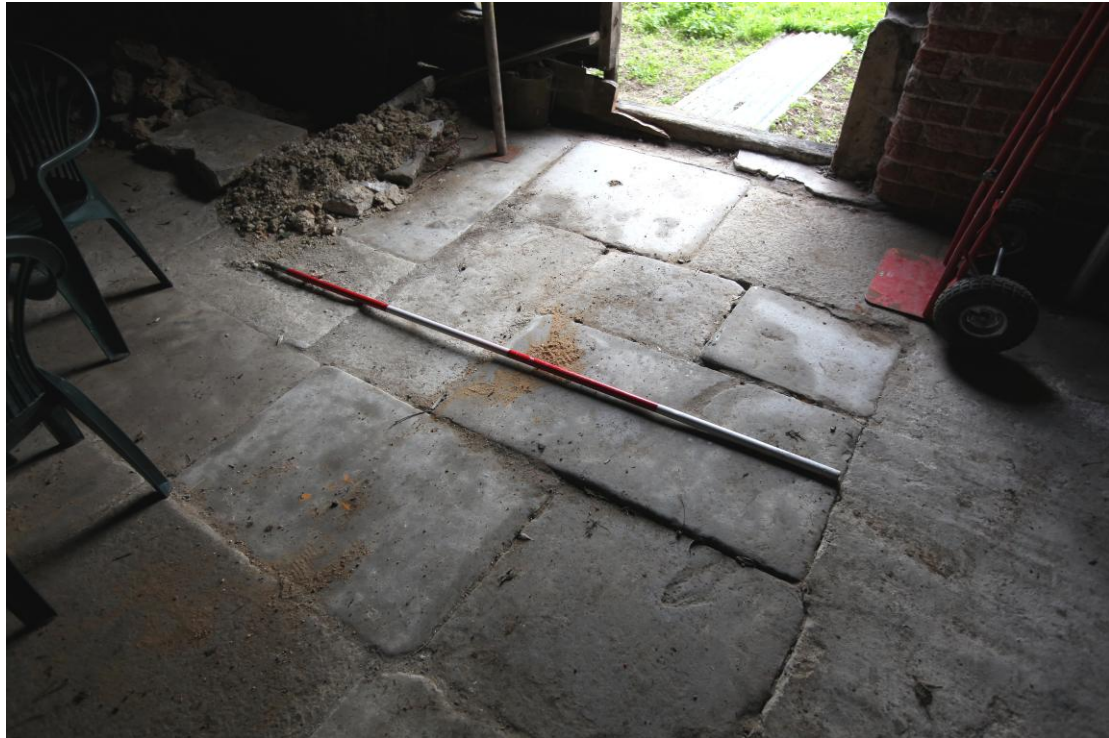
Illus. 7. Detail of the stone flag floor in the entrance bay of the barn (1) showing its southern doors to the yard. These slabs are probably re-using York paving stones and are not uncommon within a narrow radius of Ipswich.
