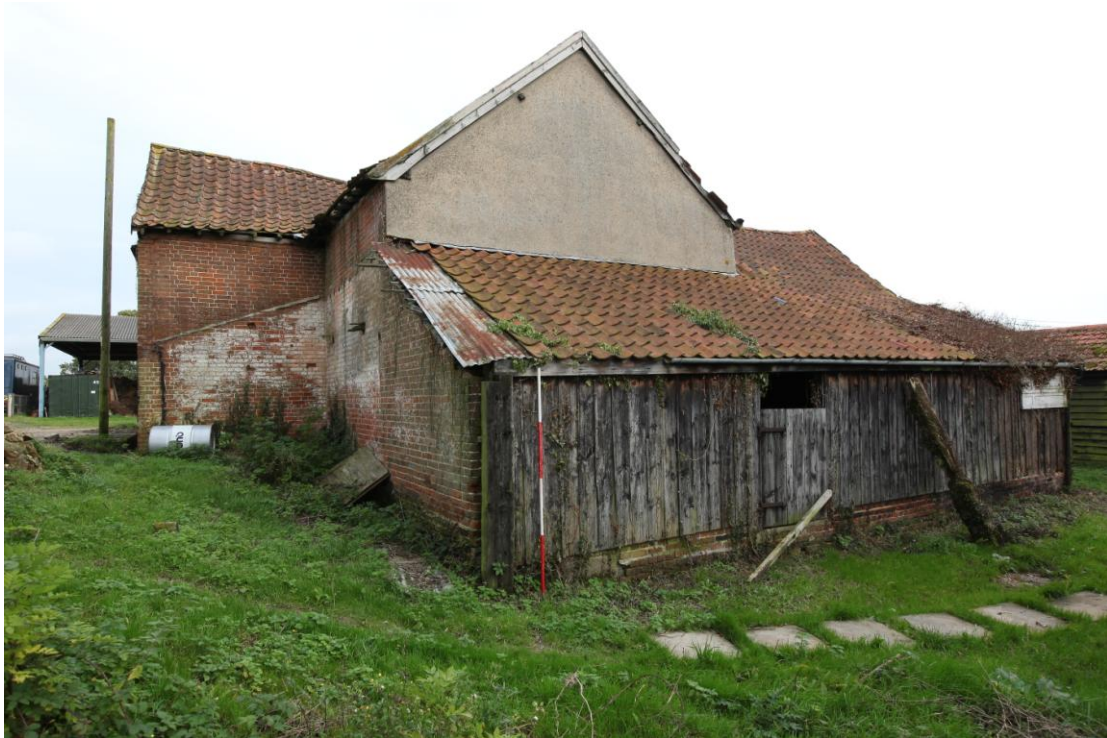
Illus. 3. Exterior from west showing the western lean-to sheds (7 & 8) in foreground with the scar of a demolished additional lean-to (6) visible on the porch.
