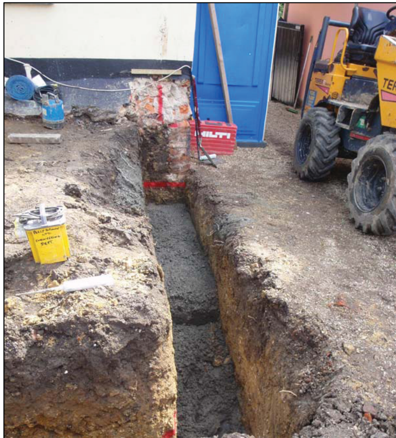
Plate II: western footing trench showing earlier underpinning of the main house (camera facing southeast)
