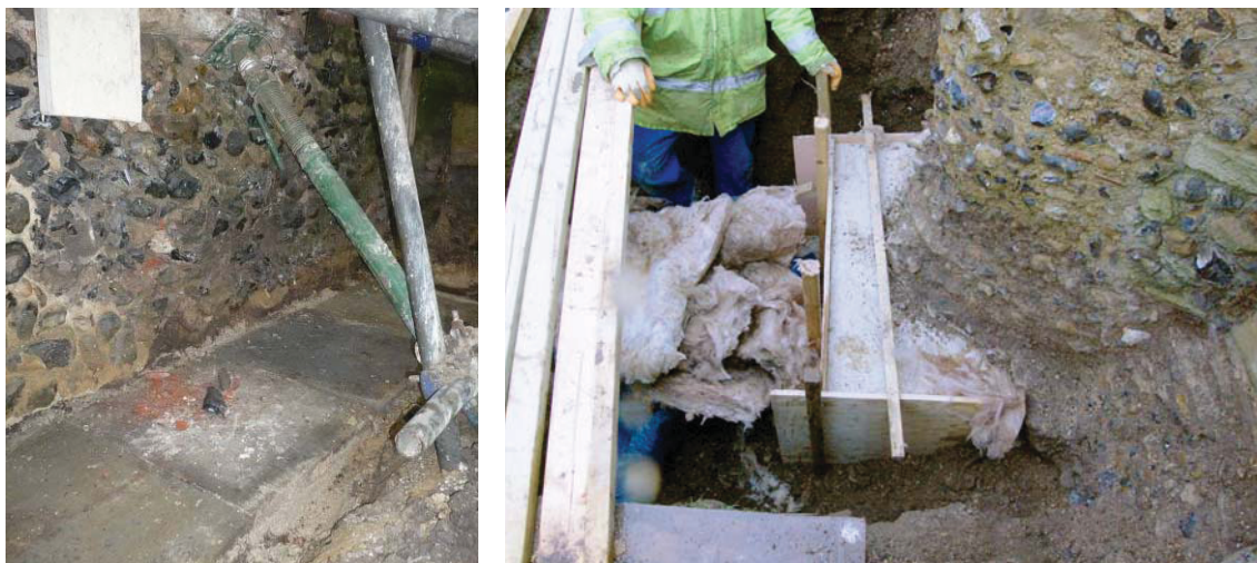
Area 1 Paving slabs at the base of the south side of the wall prior to the breaking out of the face and underpinning of the north face reveal
