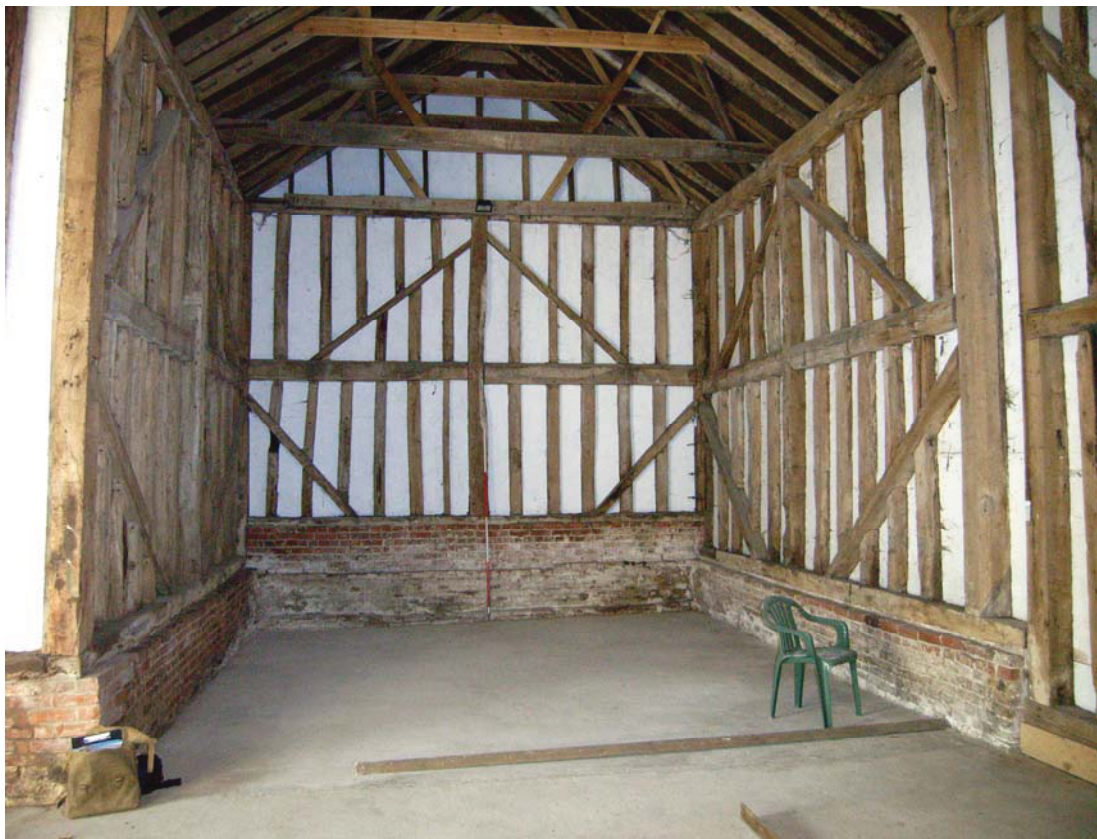
A2.4 Interior of barn from east showing primary wall bracing with re-used timbers and the southern porch to left.
