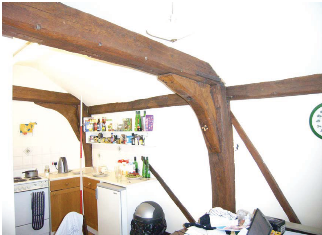
A2.10 Northern internal elevation of converted loft showing apparently in situ late-16 th century framing with open truss to left and closed truss with empty stud mortises in centre (and position of first-floor door to right). The bolted knee-braces are 19 th century insertions.
