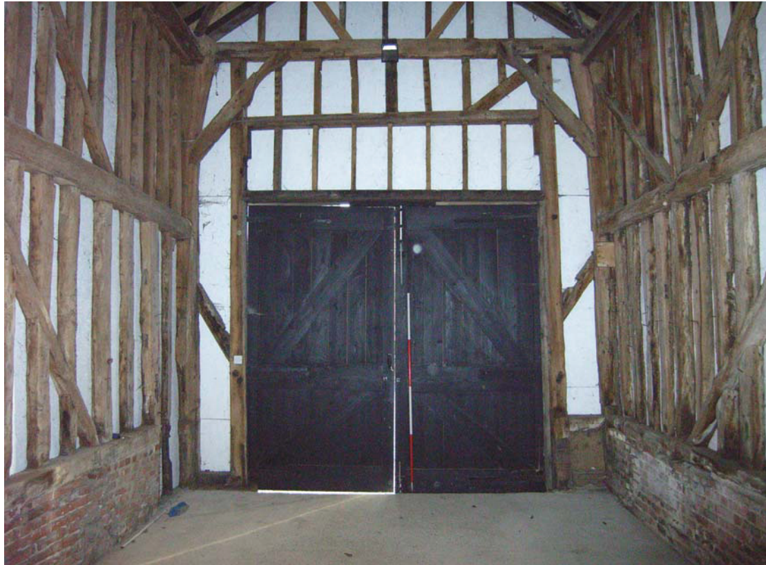
A2.7 Internal southern gable of porch showing corner braces and jambs of original doorway (now reduced in height).
