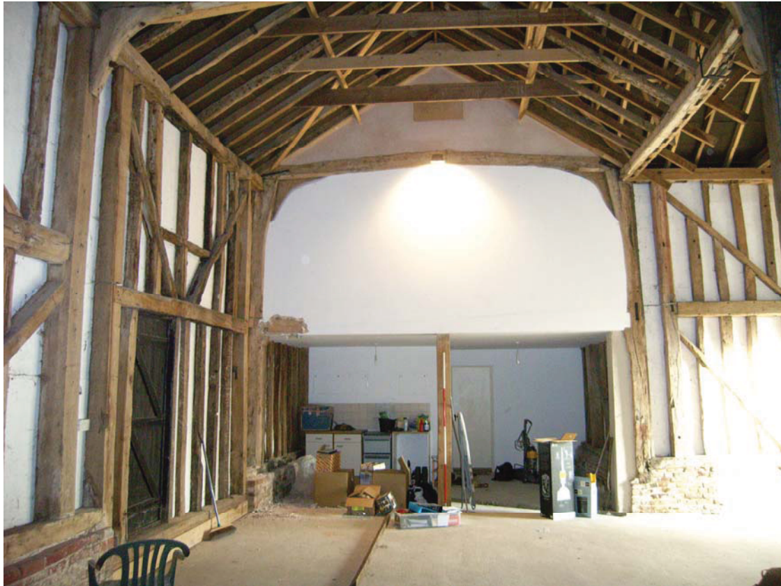
A2.5 Interior from west showing previously converted loft in eastern half of barn with porch to right and blocked northern door to left. The corbel blocks of the storey posts supporting the loft are visible at both sides.
