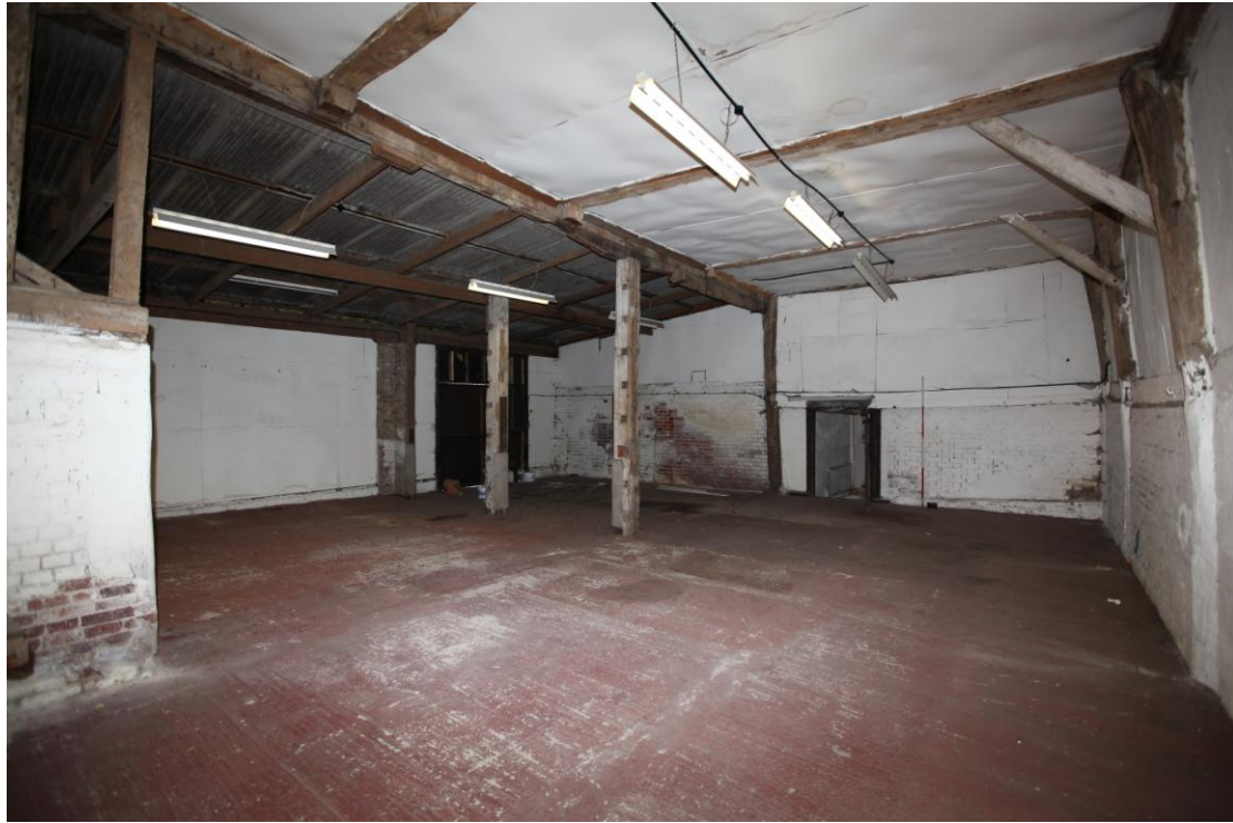
Illus. 13. Interior of 'barn' (G) from eastern gable showing original 16th century timber frame of four bays to right and 20 th century lean-to extension to left. The southern elevation to the left has been largely removed along with the original ceiling but the vertical posts may be its recycled binding joists.
