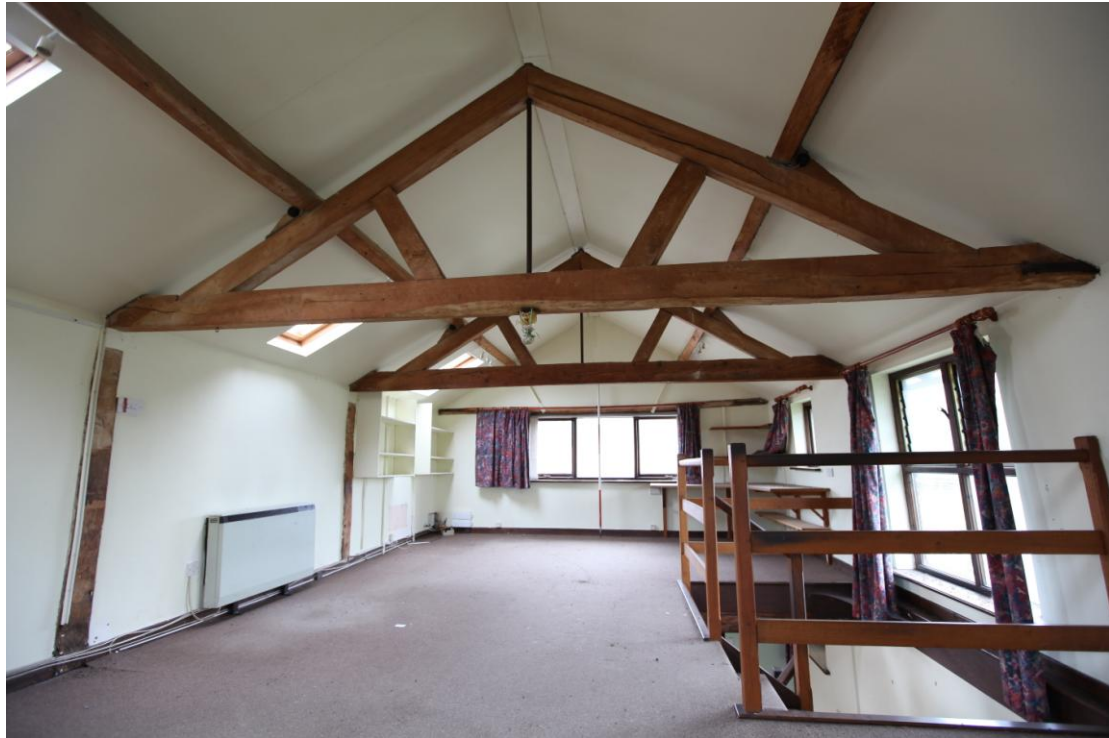
Illus. 7. Converted upper storey of granary (C) from north showing A-frame roof trusses with raking queen struts.
