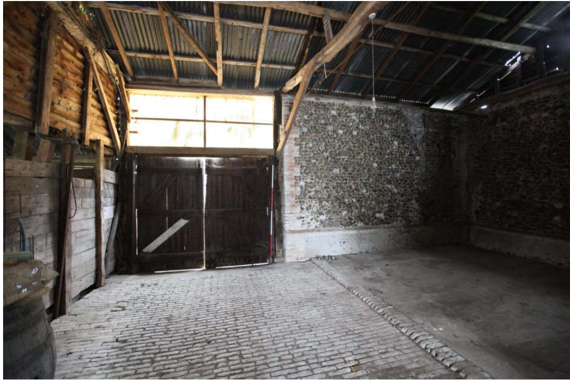
Illus. 11. Eastern interior of the barn (1) showing its gault brick threshing floor and the original entrance doorway to the left.
