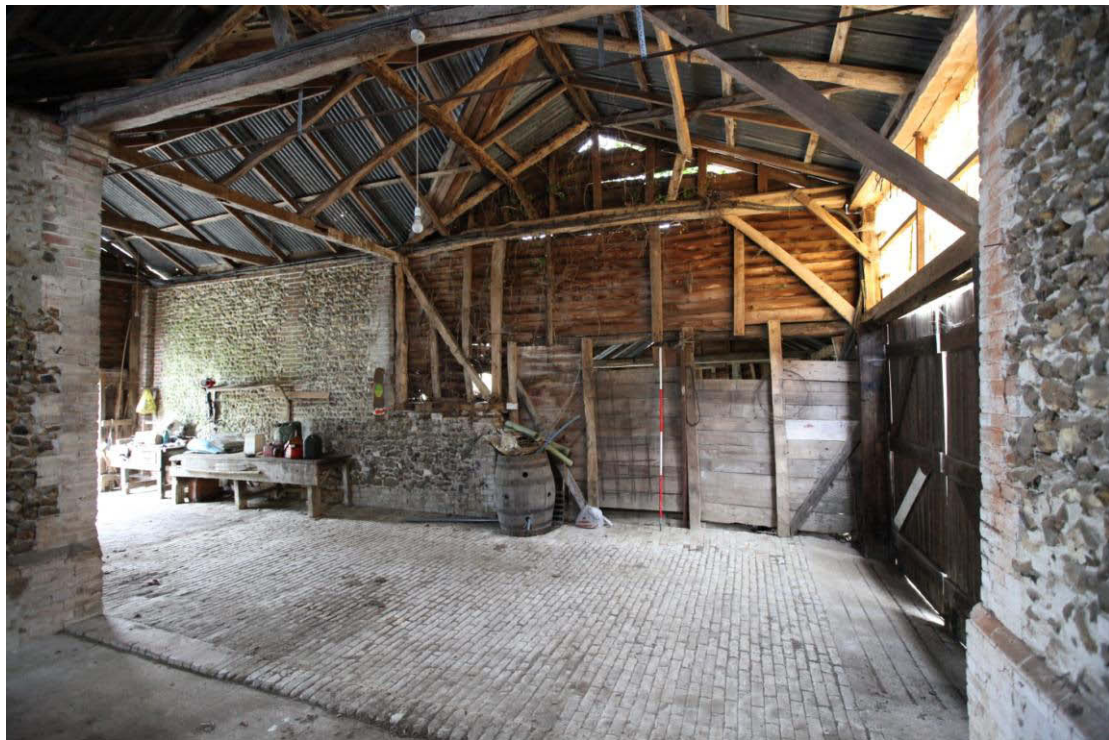
Illus. 10. Interior of the flint barn (1) from the south showing its long flint porch to the left and the boarded partition against the stable (2) to the right. The flint plinth and stud wall in the centre probably reflects the original appearance of the porch before its timber upper walls were rebuilt.
