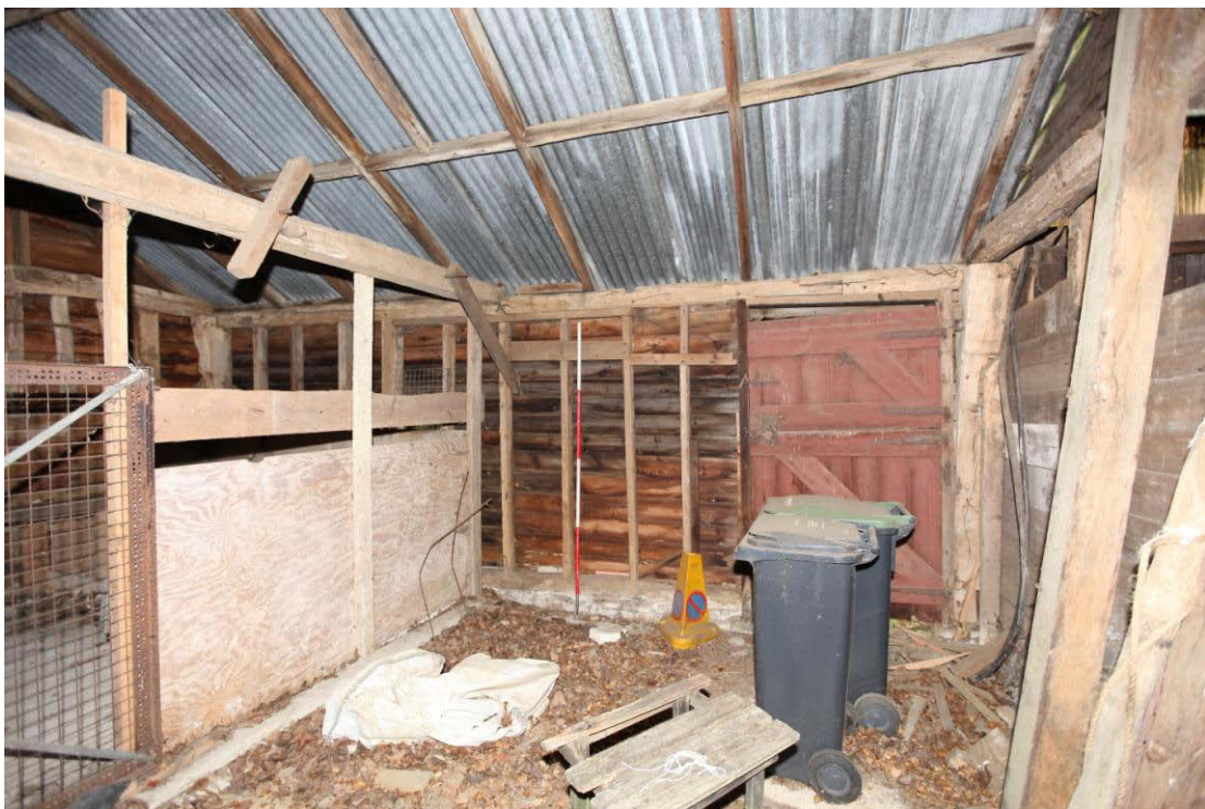
Illus. 8. The eastern interior of the stable (2) showing the external door adjoining the barn (1) to right and narrow 20 th century studs. The recent boarded partition to the left forms a dog kennel with a separate entrance in the western elevation.
