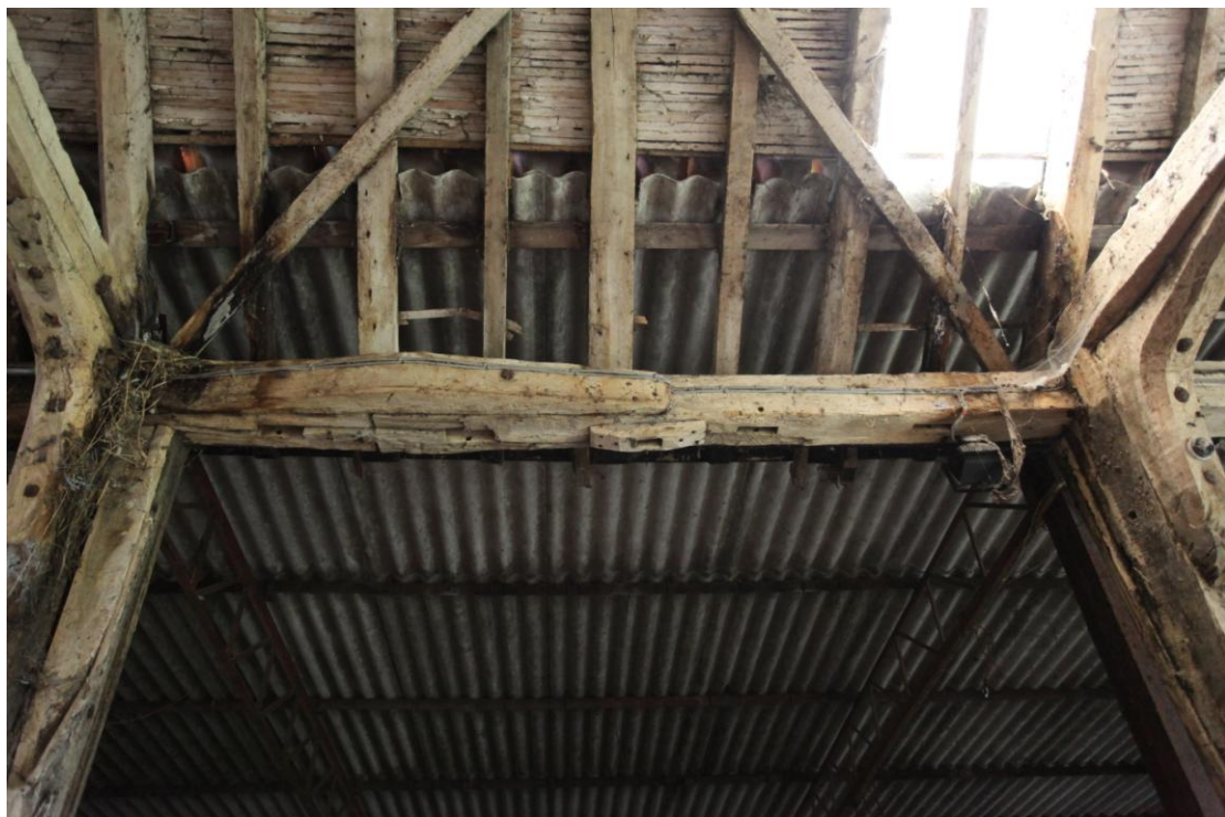
Illus. 8. Western roof-plate of the entrance bay of the barn (5) seen from the east and showing empty stud mortises with a central gap for a narrow rear door. The wooden housing for a door bar is a later addition. An edge-halved and bridled scarf joint is visible to the left (partly hidden by a bolted repair).
