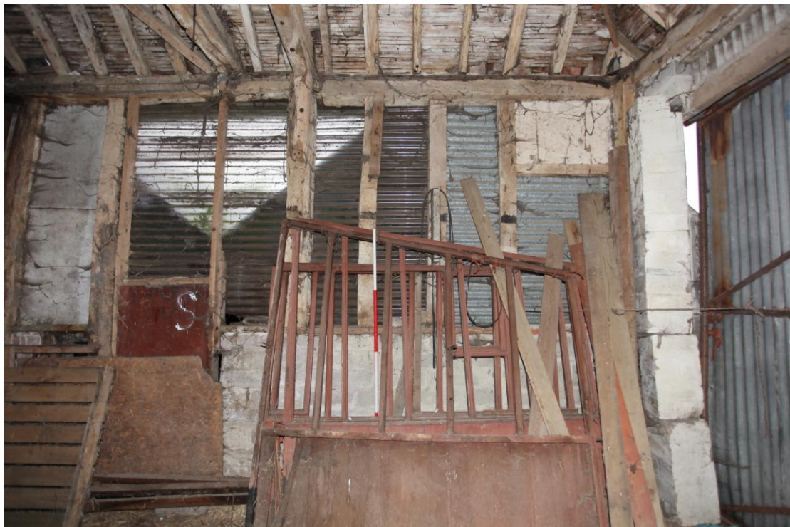
Illus. 10. The eastern interior of the added stable bay (5a) showing the intact diamond mullion window of its hay loft top right and the unpegged stud which probably indicated the position of the original entrance door to the right of the central post which marks the original gable of the barn (5).
