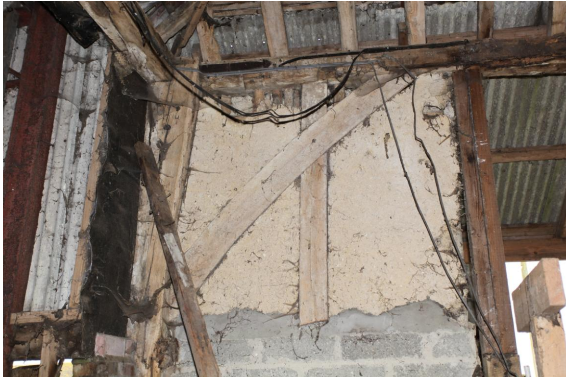
Illus. 7. Detail of the original framing with internally trenched brace in the western section of the northern internal gable of the barn (5). The tie-beam is a re-used replacement of the 19 th century which relates to the present hipped roof.
