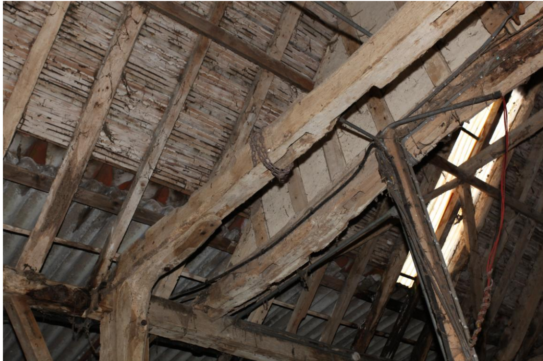
Illus. 9. Detail from the south-east of the original tie-beam of the southern gable of the three-bay barn (5) showing its hip-rafter notches and empty stud mortises. The tie-beam and remaining partition of the stable (which intruded into the barn by 0.5 m) is shown in the rear to the right.
