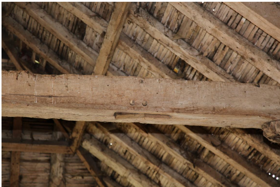
Illus. 12. Detail of the only original open truss tie-beam to survive in the barn (5) – to the north of its entrance bay – showing a pegged mortise for a missing arch-brace in its lower surface and the peg of a queen-post mortise in its upper. Queen post roofs were largely confined to the northern half of central Suffolk in the 16 th century.
