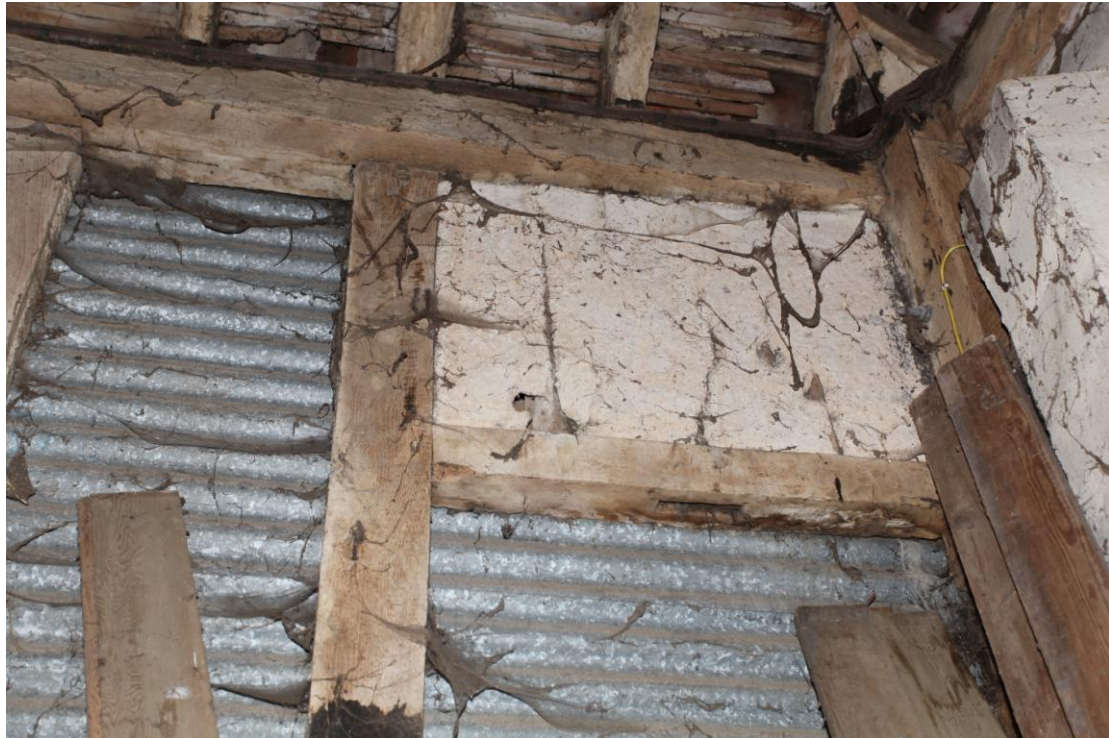
Illus. 11. Detail of the intact original diamond mullion window of the hay loft above the stable (5a), now blocked with clay daub but appearing to retain all three mullions.
