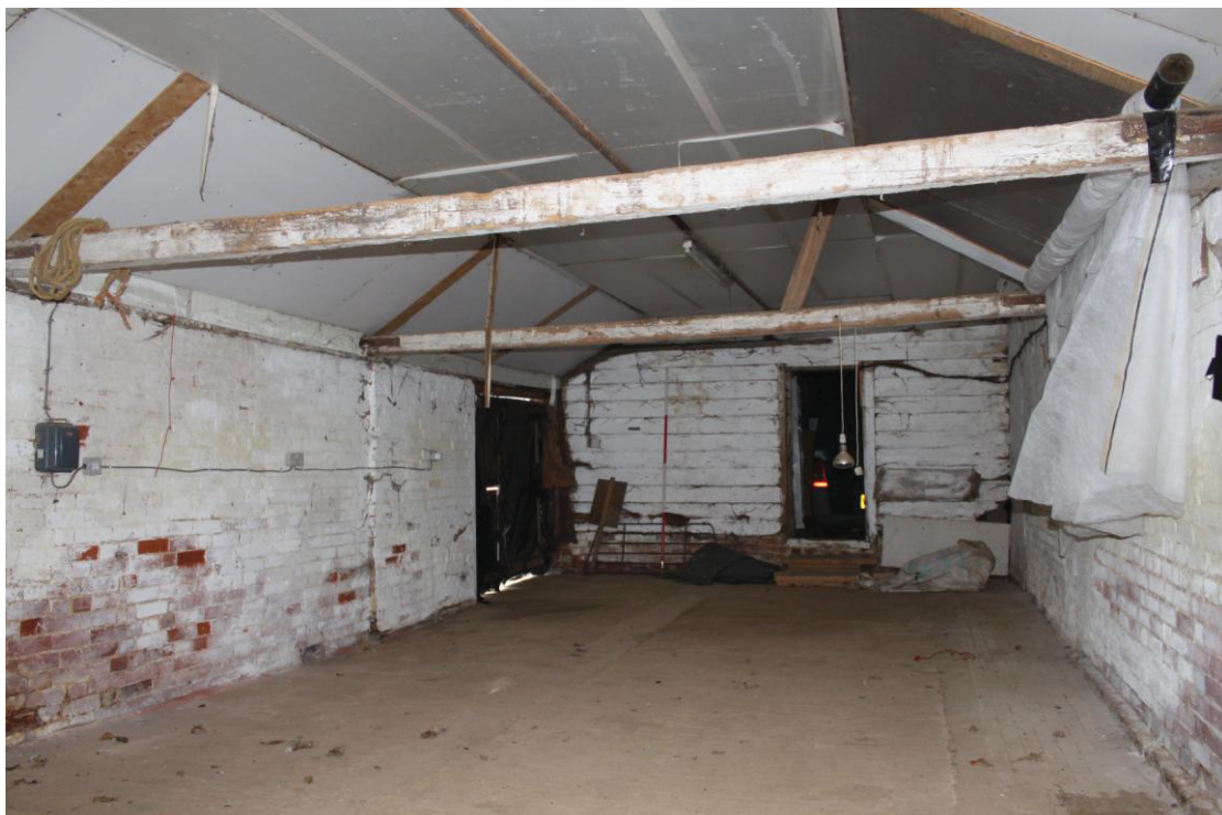
Illus. 6. The interior of the enclosed shed (1) from the east showing the boarded gable and door of the barn (6) in the rear with a butt-joint in the brickwork of the southern elevation to the left. The ceiling consists of modern plasterboard.
