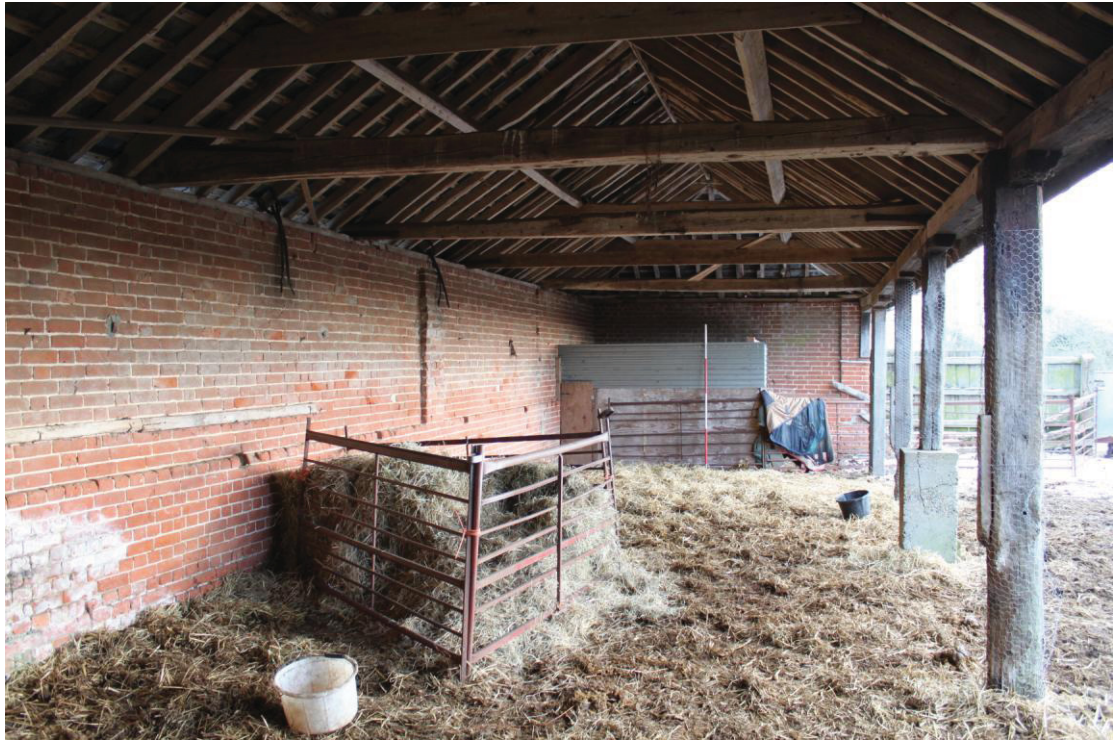
Illus. 9. The interior of the western shelter-shed (4) from the north, showing its original softwood roof and replaced arcade posts to the right. The building was in use as a horse shelter at the time of inspection.
