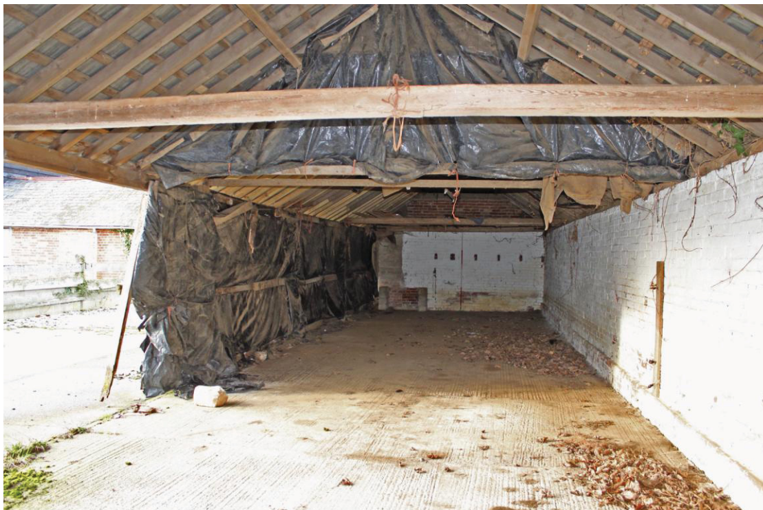
Illus. 8. The interior of the eastern shelter-shed (3) from the south showing its rebuilt roof structure of modern softwood with the solid wall adjoining the corner shed (2) in the rear.
