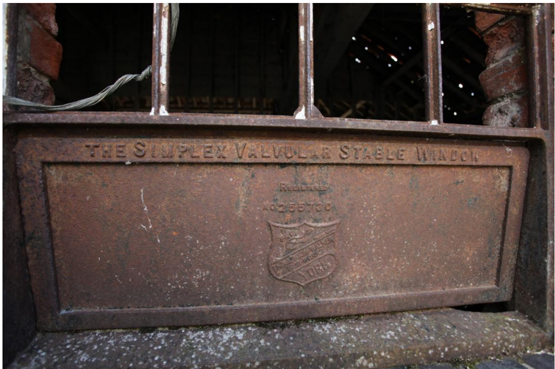
Illus. 12. Detail of a pivoting lower section of the cast iron windows of the western cowshed (5a) bearing a registration number and founder's badge (Thomlinson and Walker Ironworks, York) with the name 'The Simplex Valvular Stable Window'.
