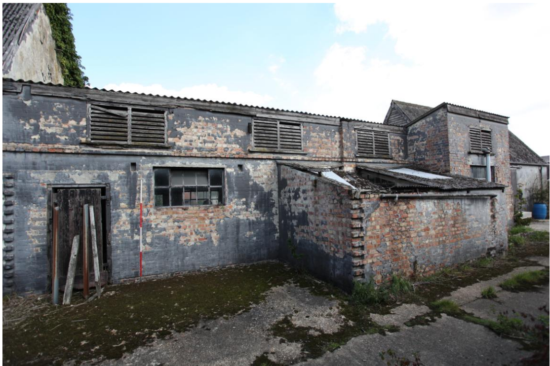
Illus. 8. South-western exterior of the brick milking parlour (2) showing the barn (1) to left & the lean-to shed (2c) to the right with the 18 th century stable (3) to the far right.
