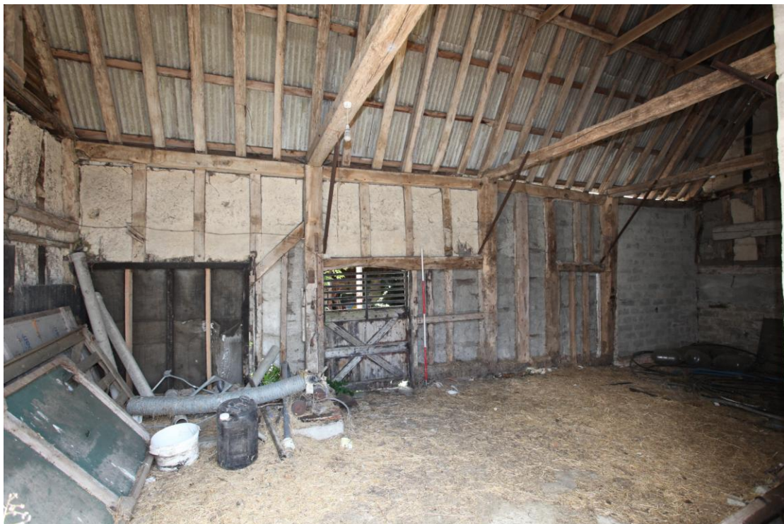
Illus. 10. The north-eastern interior of the 18 th century stable (3) showing its two original doors to right and left (the former blocked but retaining its lintel) with the clamp of its missing hay loft joists visible on the north-western gable to the left.
