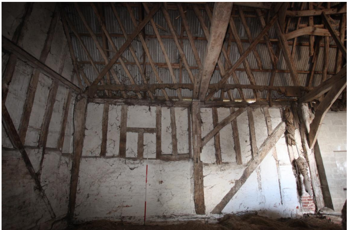
Illus. 4. The north-eastern interior of the stable bay (1b) at the north-western end of the barn showing the blocked window of its removed hay loft and the lintel of its blocked door adjoining the central storey post. The internally trenched brace to the right rose from the corner of the three-bay threshing barn (1a). The rafters have racked to the left.
