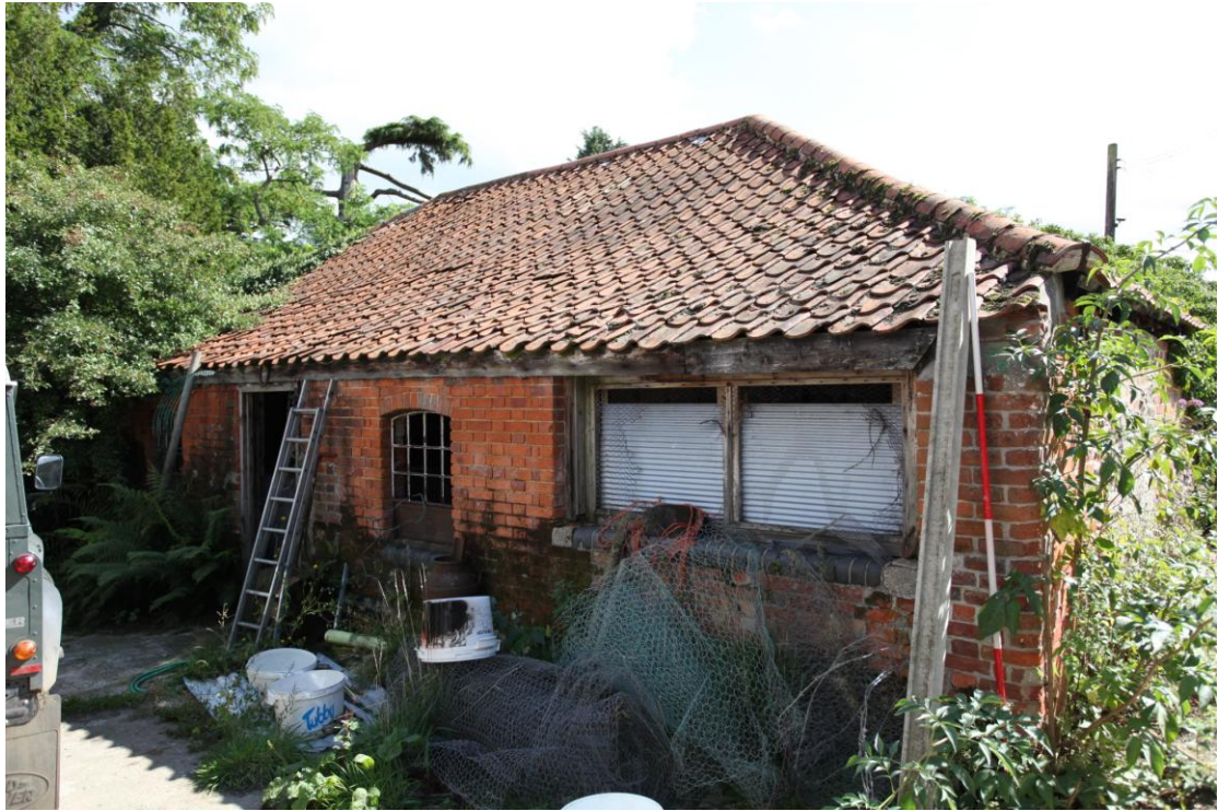
Illus. 11. The north-western exterior of the western 19 th century cow-shed shed (5a) showing its original cast iron windows to the left and a secondary hatch to the right.
