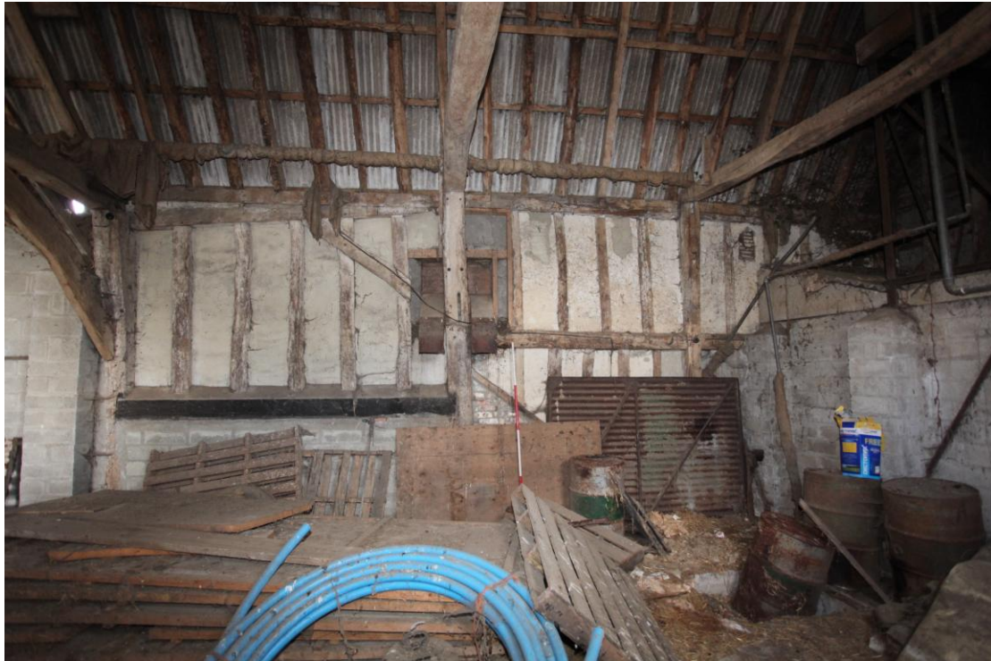
Illus. 5. The southern end of the barn's north-eastern interior showing the junction between the original 16 th century structure without mid-rails to the left and the two-bay 17 th century extension with smaller studs and mid-rails to the right. The ground-floor partition to the right is an intrusion from the adjoining brick milking parlour (2a).
