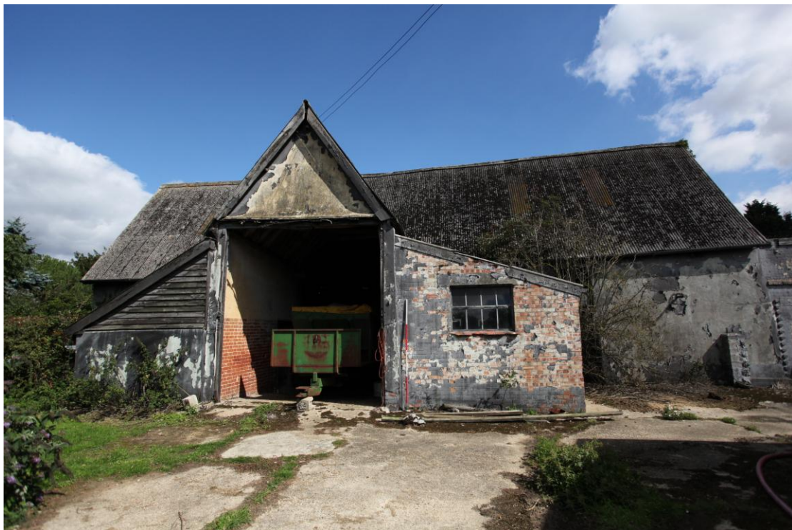
Illus. 2. South western exterior of barn (1) showing 19 th century porch (1d) flanked by lean-to sheds.
