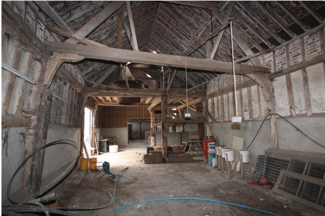
Illus. 5. The interior of the barn (1) from the north showing the 20 th century grain floor and hopper in the entrance bay and the raised walls to right and left (short studs infilled with brick above the original roof-plates).
