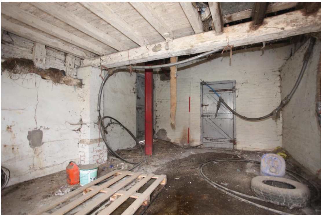
Illus. 10. The interior of southern stable (2b) from the east showing a surviving section of the original ceiling of lodged joists to the left. The door to the right opens onto the 20 th century western shed (4).
