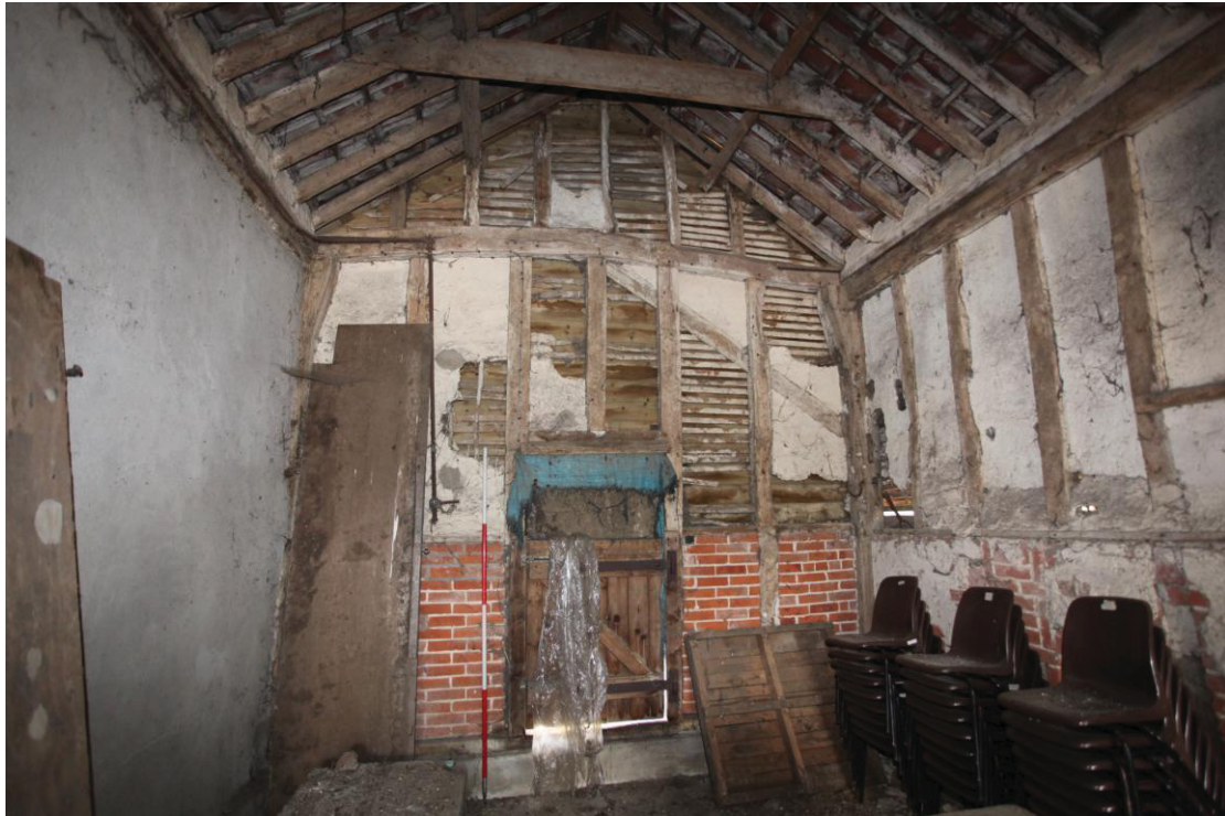
Illus. 7. The internal western gable of the 17th century porch (1a) showing its asymmetrical externally trenched wall brace with the remains of wattle-and-daub infill.
