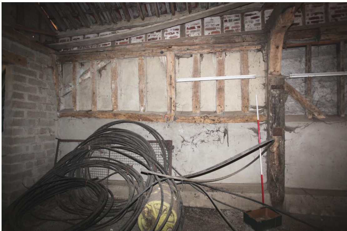
Illus. 6. The fragment of 17th century framing at the northern end of the eastern internal elevation of the barn (1), showing the mid-rail with an externally trenched brace to the left and a central storey post with an empty arch-brace mortise. The 19 th century studwork to the right lacks mid-rails and contains diagonal primary braces that interrupt the studs.
