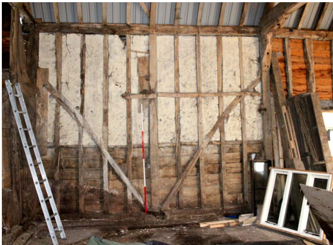
Illus. 10. Interior of northern end of south-eastern elevation showing the intermediate central post with primary diagonal wall braces and the original two-tier cladding of daub above boarding. The horizontal rail is one of many designed to secure the infill panels. The late-20 th door and weatherboarding of the central bay is visible to the right.
