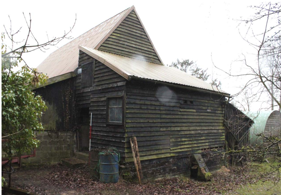
Illus. 5. Exterior of lean-to stable (2) from north-east showing overlap to roof of barn (formerly hidden by thatch).
