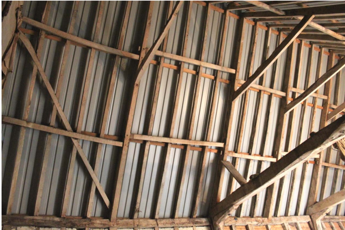
Illus. 9. The intact original roof structure of staggered butt-purlins seen from the north-west. It is steeply pitched at approximately 55 degrees for thatch but is now covered by late-20 th century sheet metal.
