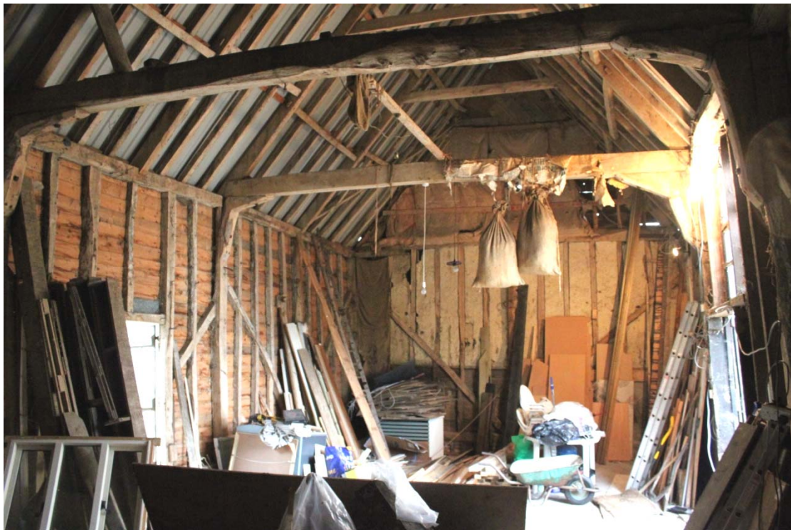
Illus. 8. General view of interior of barn from north-east showing the original bolted knee-braces to the tie-beams which flank the central entrance bay.
