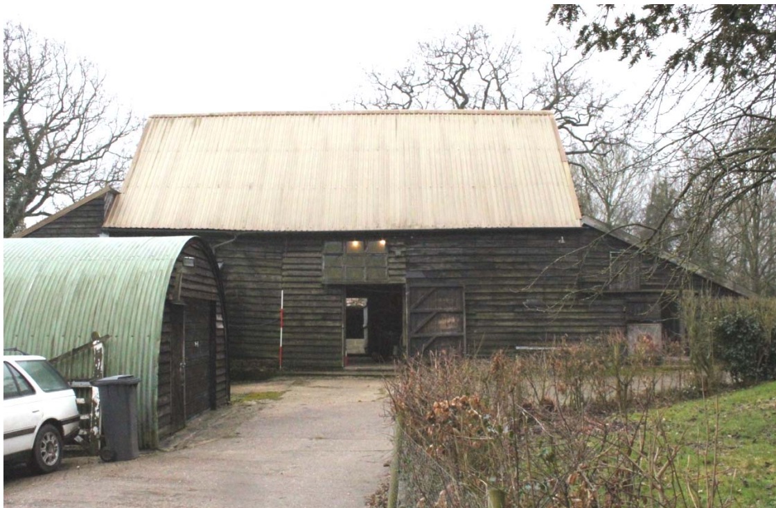
Illus. 2. Exterior of barn from north-west showing sheet-metal roof with lean-to sheds (3 & 4) to right and lean-to stable (2) behind Nissen hut to left. The barn doors in the central bay of this elevation were reduced in size during the 20 th century.
