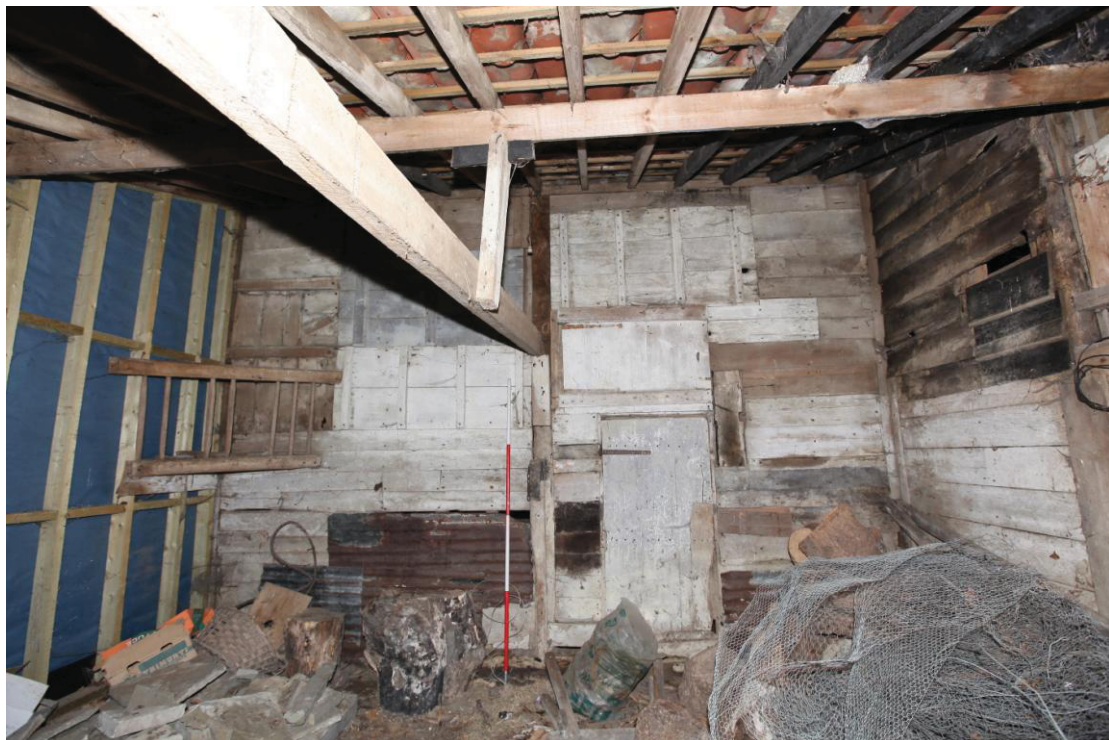
Illus. 12. The interior of the eastern section of the southern shed (2a) viewed from the east, showing the unusual partition of re-used 17 th century doors to the western section (2b). The recently rebuilt southern gable is visible to the left and the weatherboarded corner of the earlier barn to the right.
