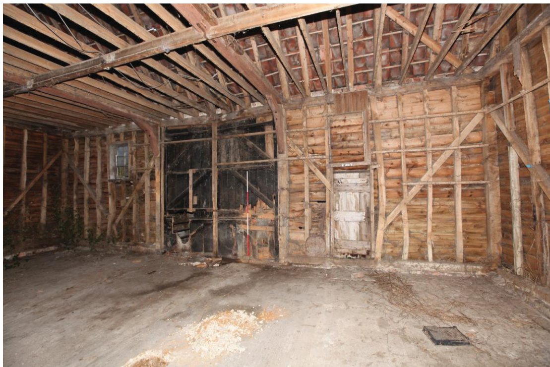
Illus. 8. The northern interior of the barn (1) showing the bolted knee-braces to the tie-beams flanking the original entrance doors (now blocked by the adjoining shed, 3) and the inserted door & (blocked) upper window of the eastern bay to the right.
