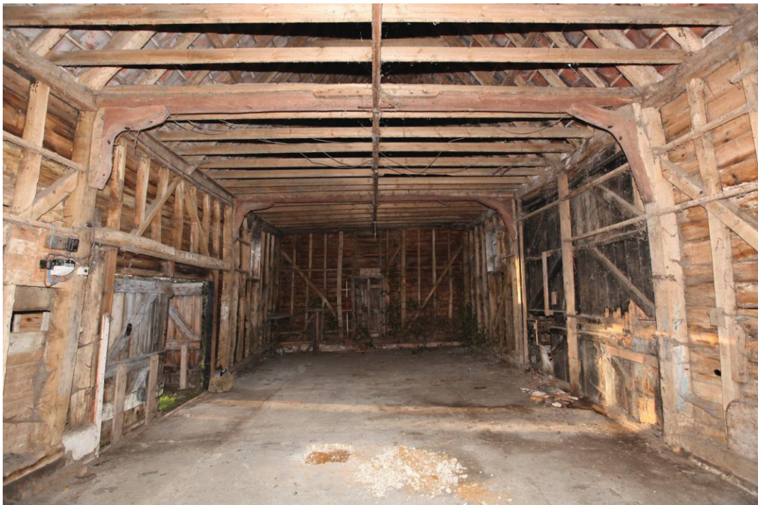
Illus. 6. The interior of the main barn (1) from the east showing its secondary ceiling at eaves height with the blocked original northern entrance to the right & the lower rear door to the left. The bolted knee-braces flanking the entrance bay and straight, primary wall braces are typical of the second quarter of the 19 th century.
