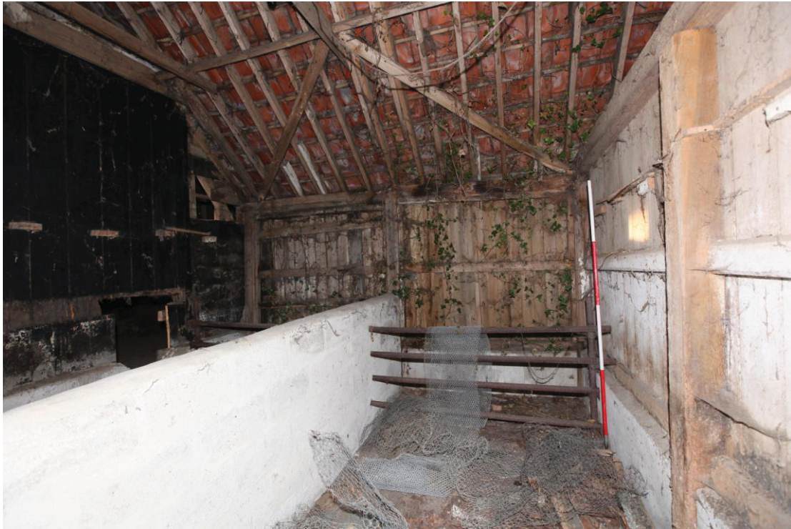
Illus. 5. The interior of southern loose box (3c) in the roadside shed of circa 1900 seen from the east and showing the iron bars and cement-block wall of the late-20 th century probable sow crates with the blocked original doors of the main barn (1) to the left.
