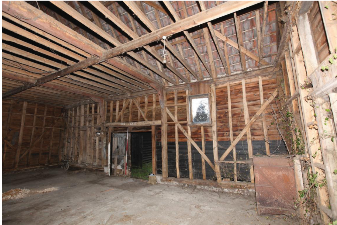
Illus. 9. The southern interior of the barn (1) from its north-western corner showing the original proportions of the low, wide rear doorway in the central bay and an inserted glazed window to the right.
