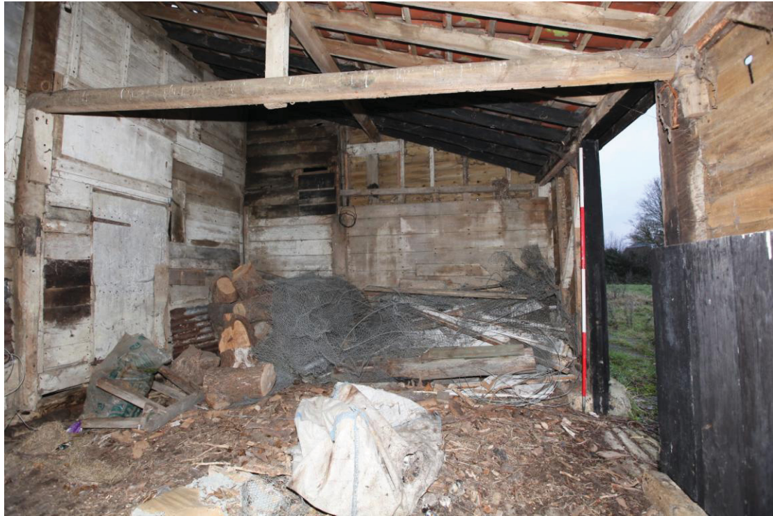
Illus. 11. The interior of the eastern section of the southern shed (2a) from the south showing the boarded south-eastern corner of the barn (1) to the left and the external door in the rebuilt eastern elevation to the right.
