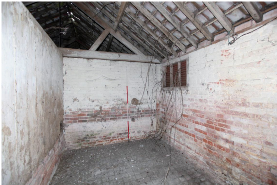
Illus. 14. Interior from the west of the south-eastern stall (Duke) of the western stable (5b) showing the original window to the southern yard to the right. The horizontal band of unpainted brick indicates the position of a missing manger but there is no evidence of a hay rack, which would have obstructed the window. Instead, a pair of curved abrasion marks to the left of the scale rod indicates the position of a hanging hay basket.
