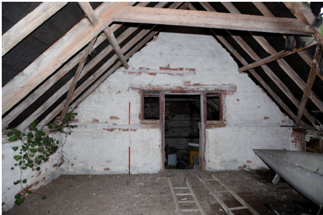
Illus. 6. Internal southern gable of the first-floor granary (1) showing the rendered brickwork with red pigment to the door and window frames (beneath later whitewash) and the roof structure of staggered butt-purlins.
