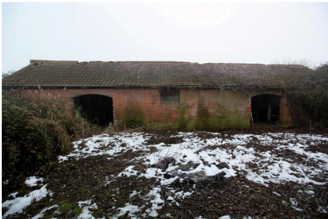
Illus. 10. Southern exterior of the single-storied stable (5) showing the arched entrance of the eastern stable (5a) to the right and the western stable (5b) to the left. The louvered window in the centre lights the south-eastern stall of the western stable (Duke).
