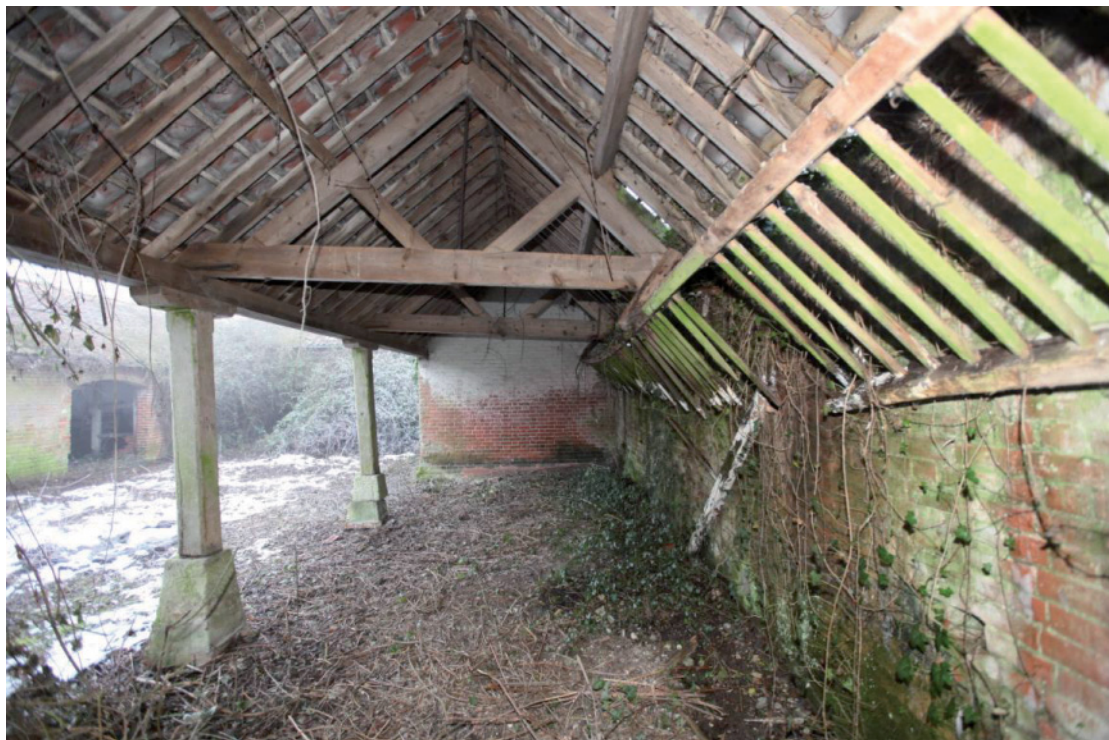
Illus. 8. Interior of the shelter-shed (6b) from the west showing the long hay rack to the right and timber posts on stone blocks adjoining the horse yard to the left.
