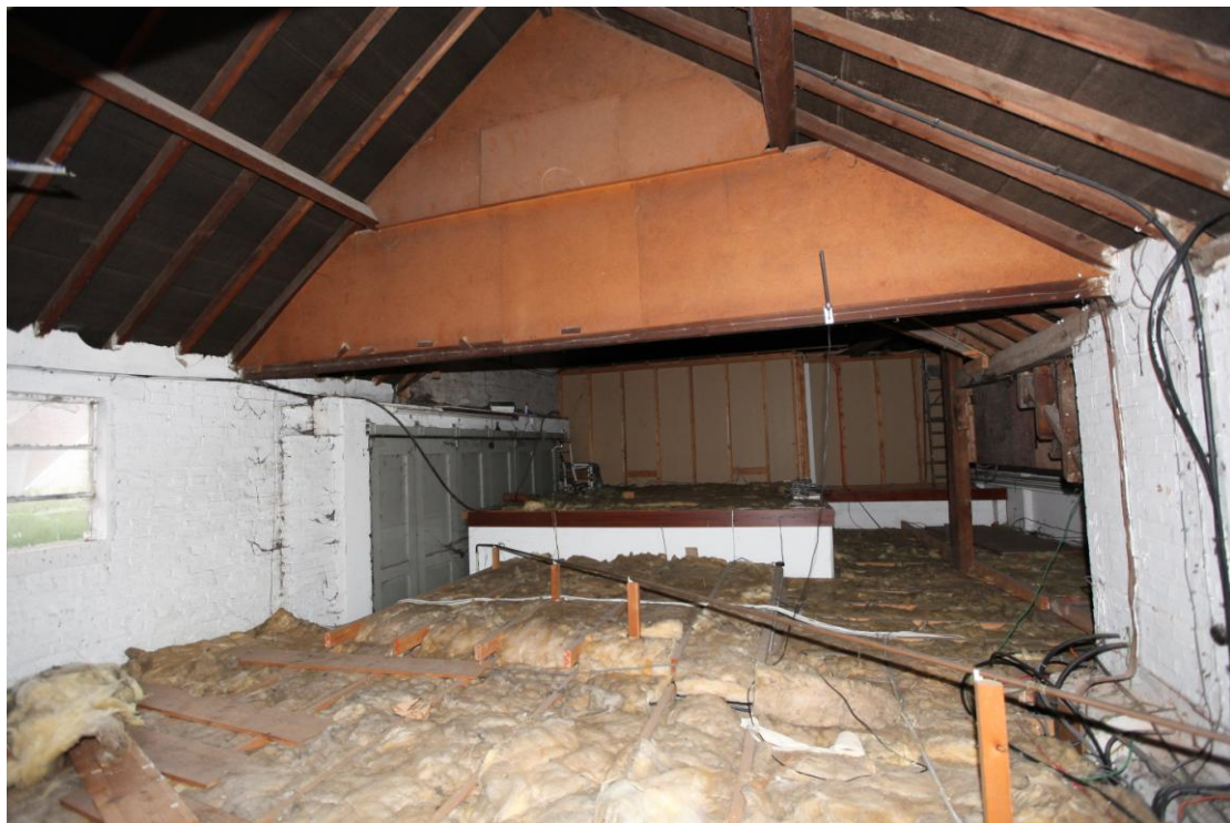
Illus. 12. The southern end of the first-floor malting range (5) showing its junction with the street range with the large 20th century vehicle doors to left blocked by late-20 th century internal partitions.
