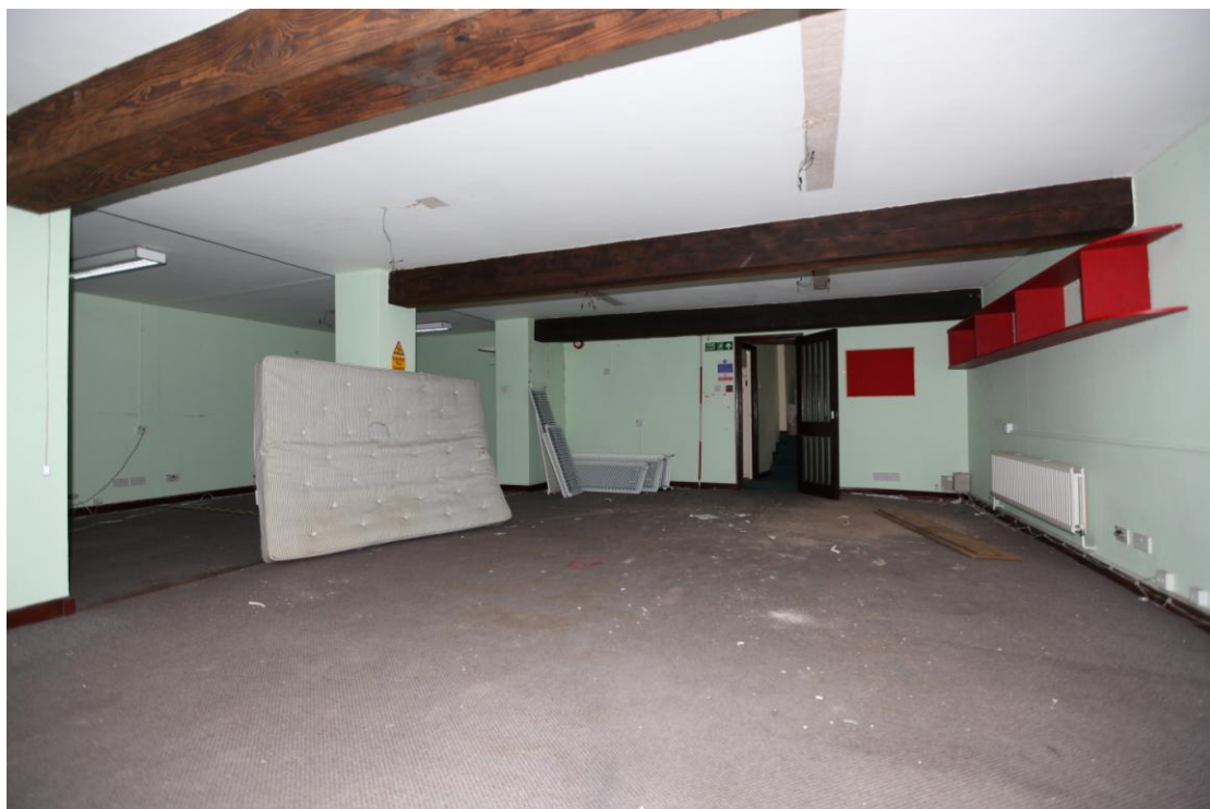
Illus. 8. The interior of the 19 th century street range (3) from the west, showing the original pine binding joists. The historic fabric is otherwise entirely concealed by the dry-lining of a modern office (including the flint-rubble northern wall to the extreme left).
