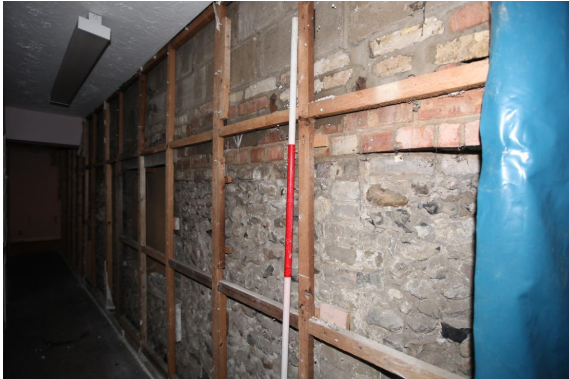
Illus. 9. The corridor of the 20 th century rear office (4a) from the west showing the recently exposed flint fabric of the northern external wall of the street range (3) to the right. This wall contains evidence of two blocked windows (each with brick dressings) but has been rebuilt above in 20 th century cement block-work and Fletton brick.
