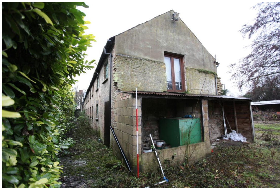
Illus. 6. The truncated northern external gable of the malting range (1) showing the remains of an outward step in the eastern elevation to the left-hand corner. The earlier brick fabric in the gable (beneath the modern cement render) probably illustrates the original height of the eaves. The laurel hedge marks the boundary with The Mill House.
