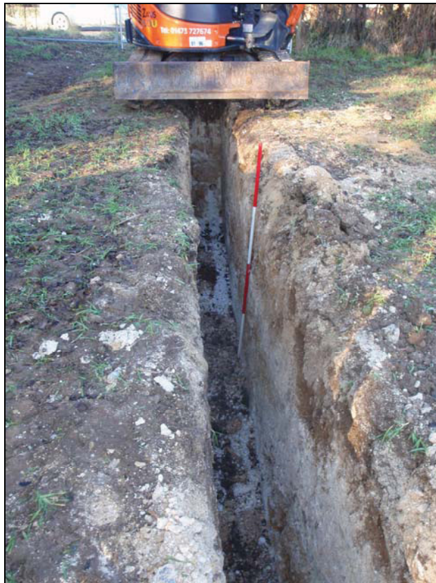
Plate VII. filter drain trench, west end, showing chalky till over solid chalk at the base, camera facing west (ref. HGK 68)
