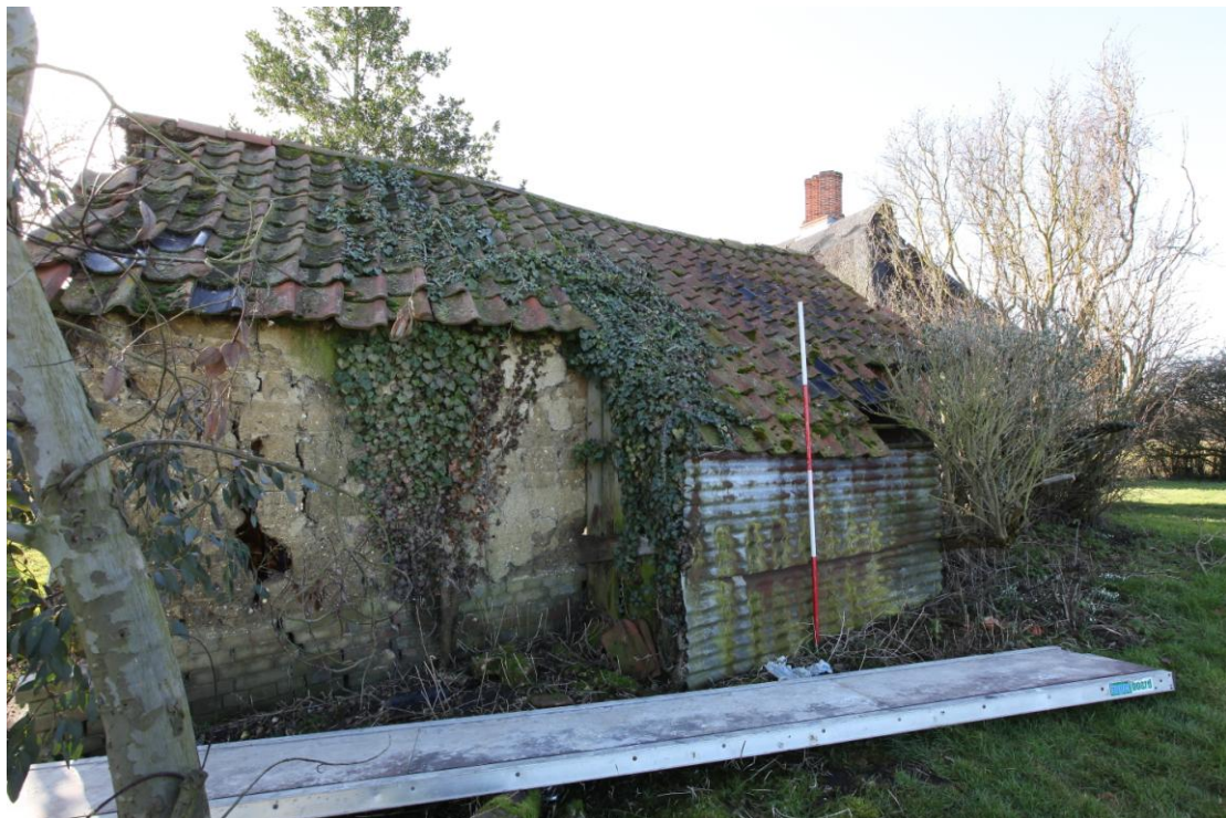
Illus. 6. The northern exterior from the north-east, showing 20th century lean-to extension to the central vehicle shed (5) with the farmhouse in the rear. The eastern end of the elevation has lost its render and the clay blocks are exposed.
