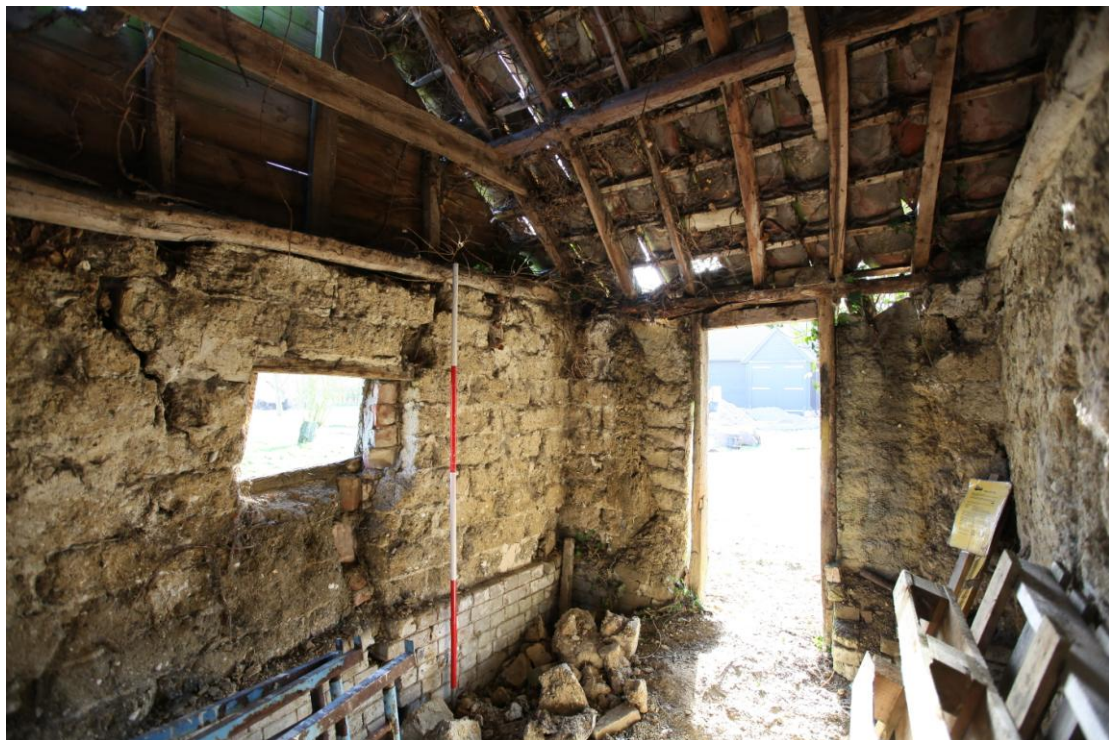
Illus. 12. The interior of the eastern shed (4) from the north showing the original southern entrance door and the softwood clapped-purlin roof structure with nailed collars.
