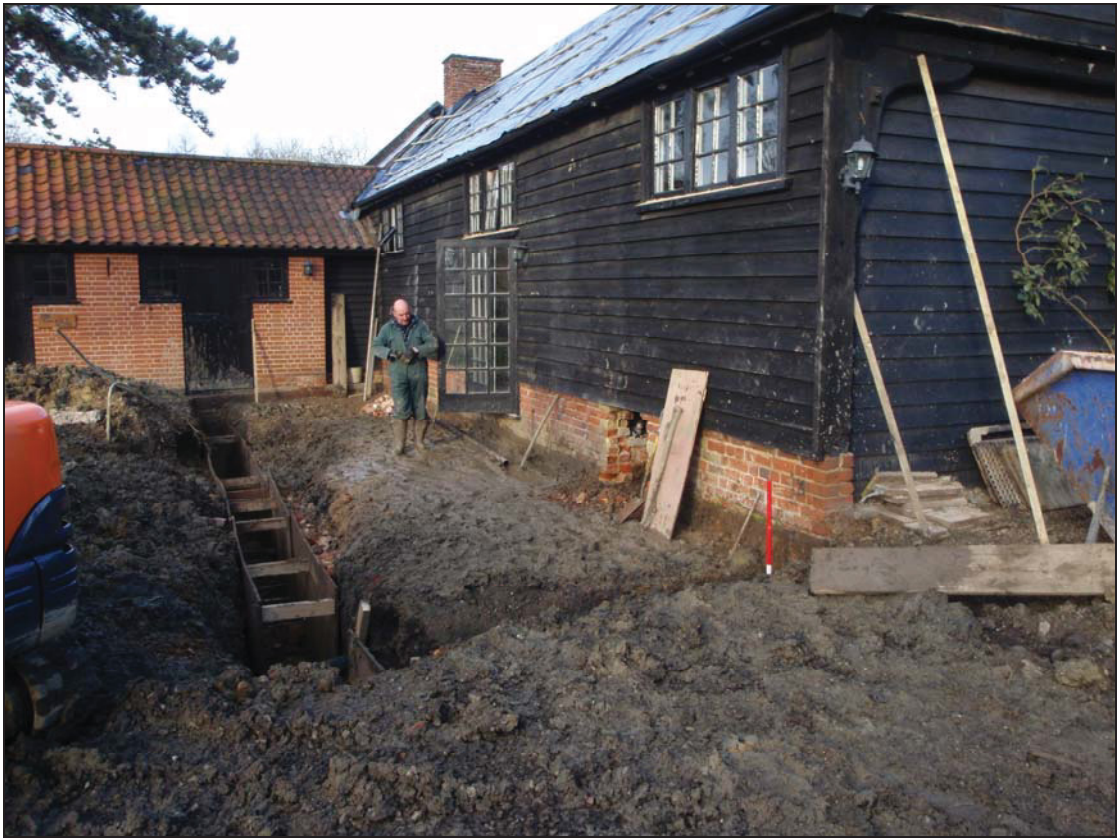
Plate I. general view of the area of the new extension (camera facing north)
