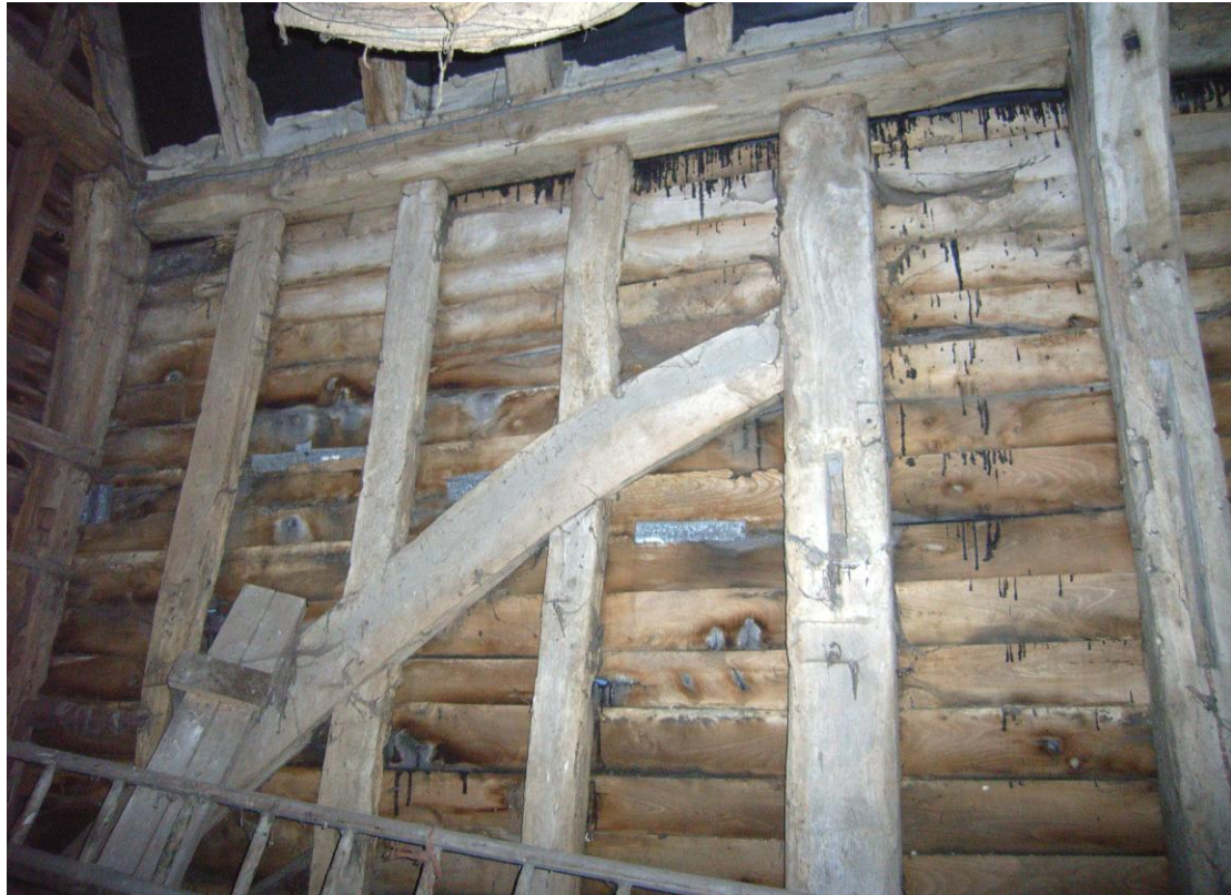
Illus. 13 Detail of barn (5) showing the unusual curved primary brace in the southern bay (re-used in the 18 th century extension and possibly taken from a contemporary stable)
