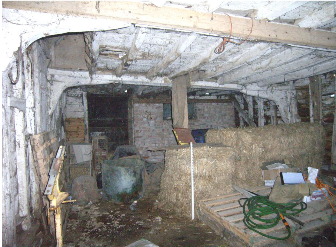
Illus. 7 Interior of the granary (2) from north, showing the loft supported by knee-braces (including a metre scale rod in centre)
