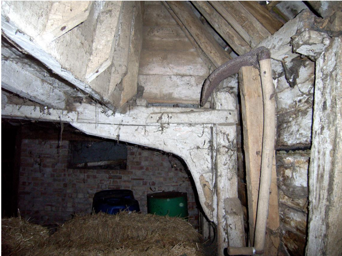
Illus. 9 Detail of granary (2) from north, showing the triangular aperture between the loft wall to left and the western elevation to right
