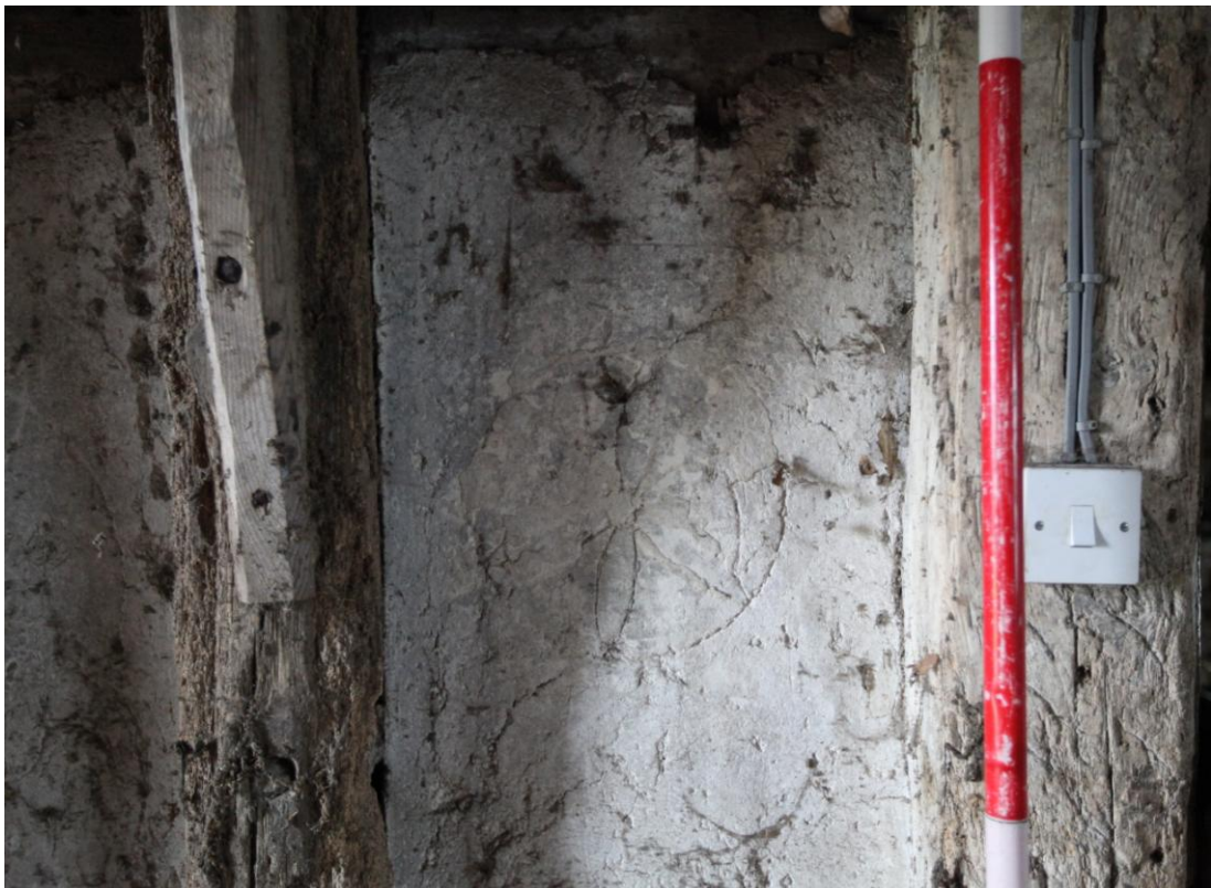
Illus. 16 Detail of the circular 'daisy-wheel' apotropaic mark incised into the clay daub of the northern interior of the porch in the barn (5). Such symbols were believed to avert evil and protect both animals and crops.
