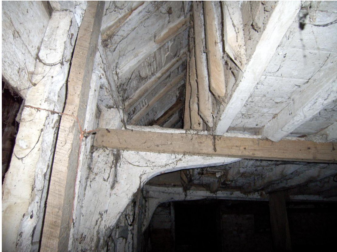
Illus. 8 Detail of granary (2) from north, showing the triangular aperture between the loft wall to right and the eastern elevation to left
