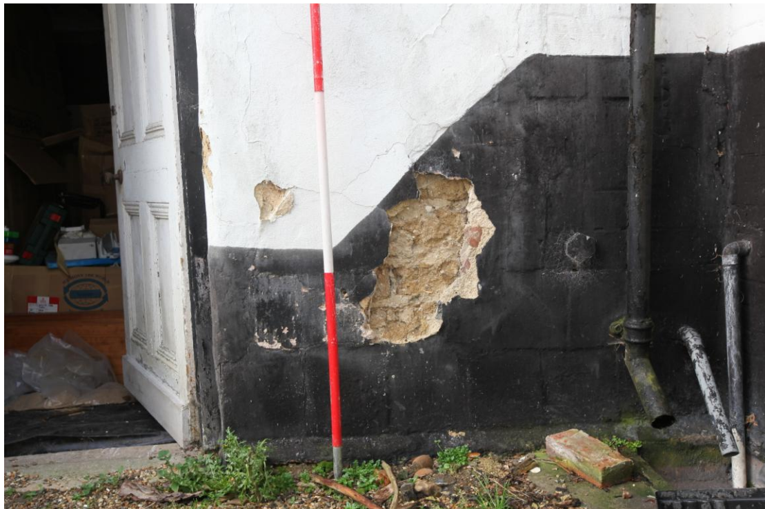
Illus. 6. Detail of the exposed clay-lump fabric in the eastern exterior to the north of the bakery door (3). This is the only exposed section of clay-lump in the building.
