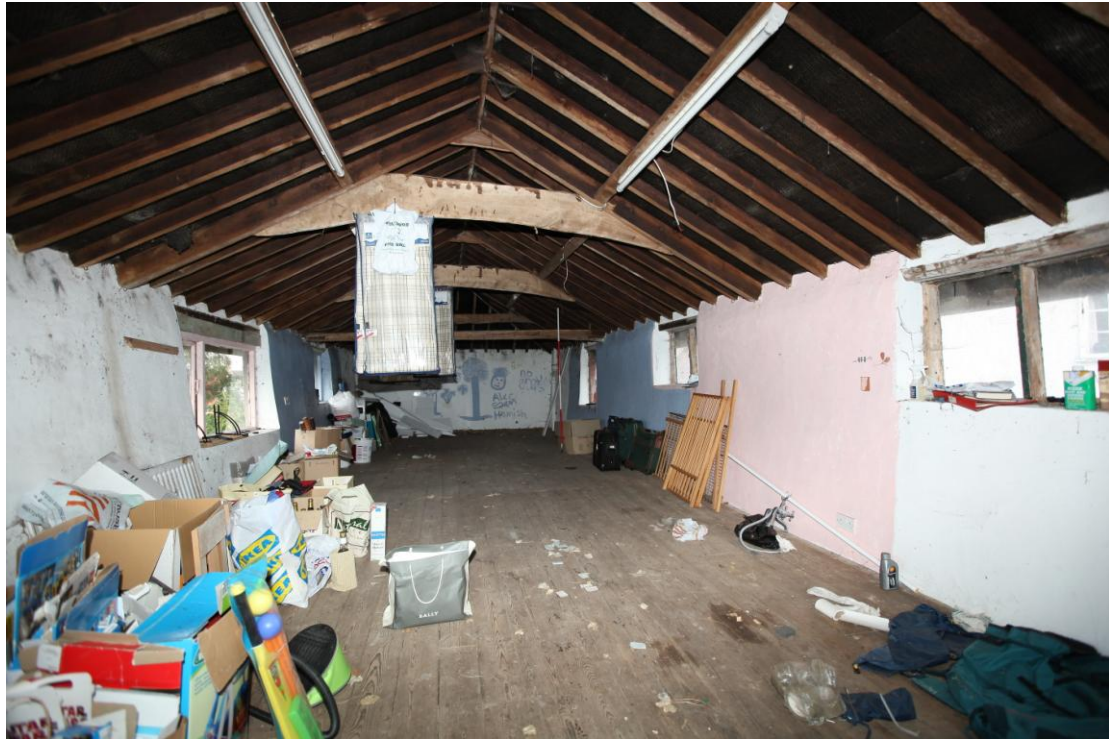
Illus. 7. The interior of the undivided upper storey seen from the south, showing its sloping clay-lump walls and the 20th century clasped-purlin roof structure of softwood joists and re-used collars.
