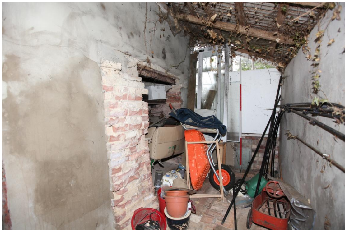
Illus. 10. The interior of the lean-to shed (4) from the east showing the truncated bread oven of Fletton brickwork to the left with cement-rendered walls and corrugated asbestos roof.
