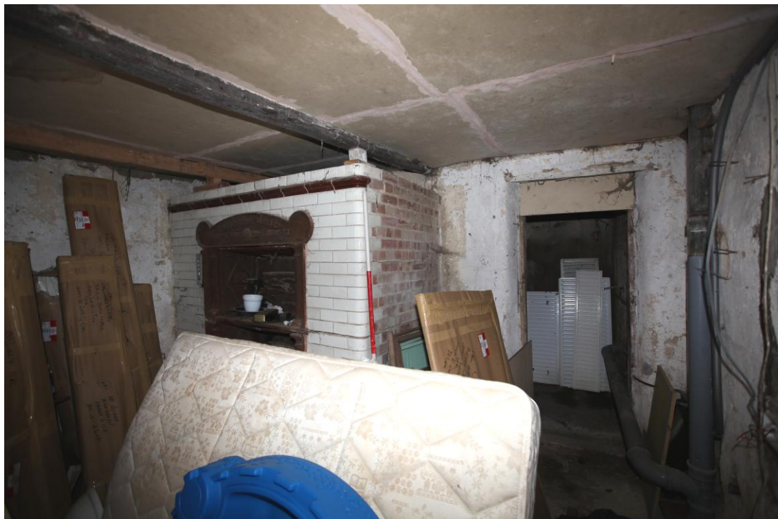
Illus. 8. The interior of the bakery (3) from the south showing the door to the gable lean-to (4) to the right and the bread oven of Fletton brick with white-glazed tiled facade to the left.
