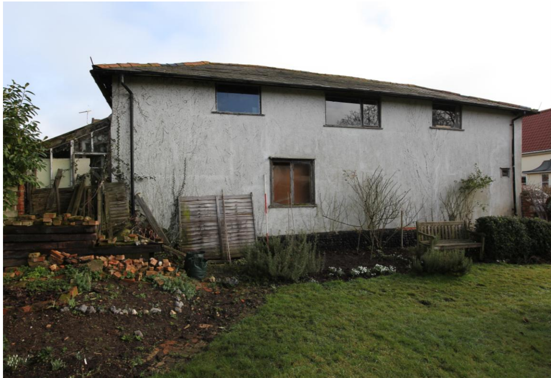
Illus. 4. The western exterior of the clay-lump outbuilding showing its shallow-pitched slate roof with late-20th century cement render and windows. The glazed lean-to shed adjoining the northern gable is visible to the left.
