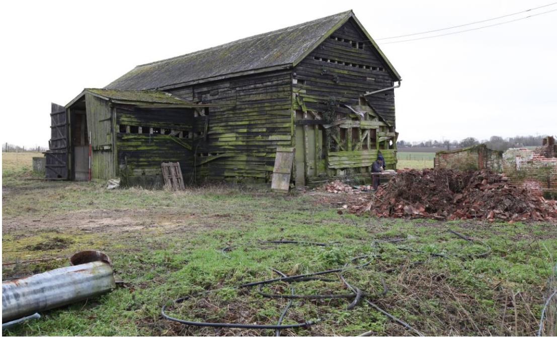
Illus. 7. Exterior of the barn (1) from the north-west showing its 20 th century corrugated asbestos roof and northern porch with the scar of the demolished shed (2) adjoining its western gable to the right.
