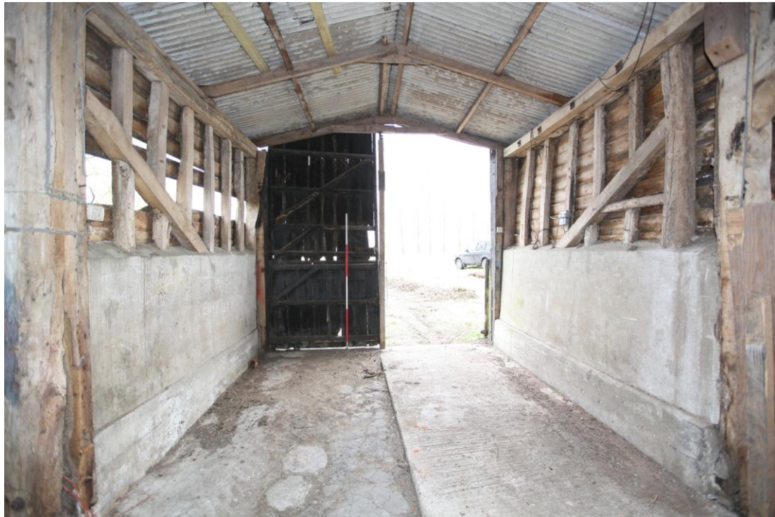
Illus. 12. The interior of the original northern porch of the barn (1) seen from the south and showing its 20th century concrete and bitumen floor. The porch was designed to increase the length of the threshing floor rather than as a principal entrance.
