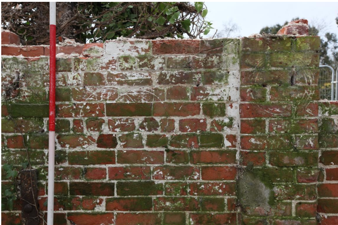
Illus. 6. Detail of the apotropaic circles to the southern interior of the largely demolished shed (2) which adjoined the western gable of the barn.
