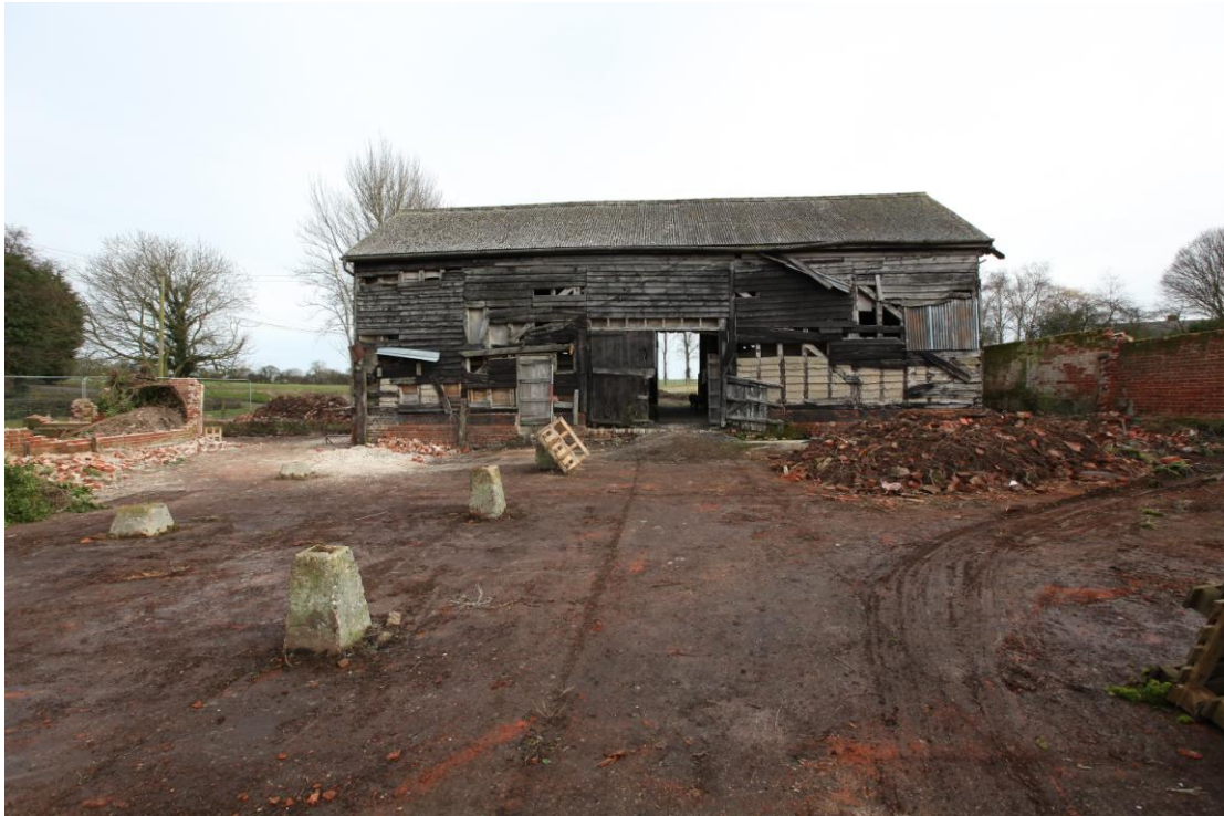
Illus. 5. The interior of the walled yard (3) from its southern entrance, showing the concrete pads of the demolished shelter-shed to the left and the scar of a central yard roof on the barn (1).
