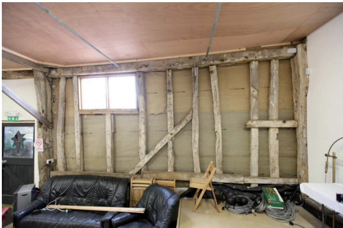
Illus. 10 The western interior of the barn's northern bay (1a) showing empty trenches for a missing wall brace to the right and later framing with a diagonal primary brace in the style of the 18 th and 19 th centuries to the left.
