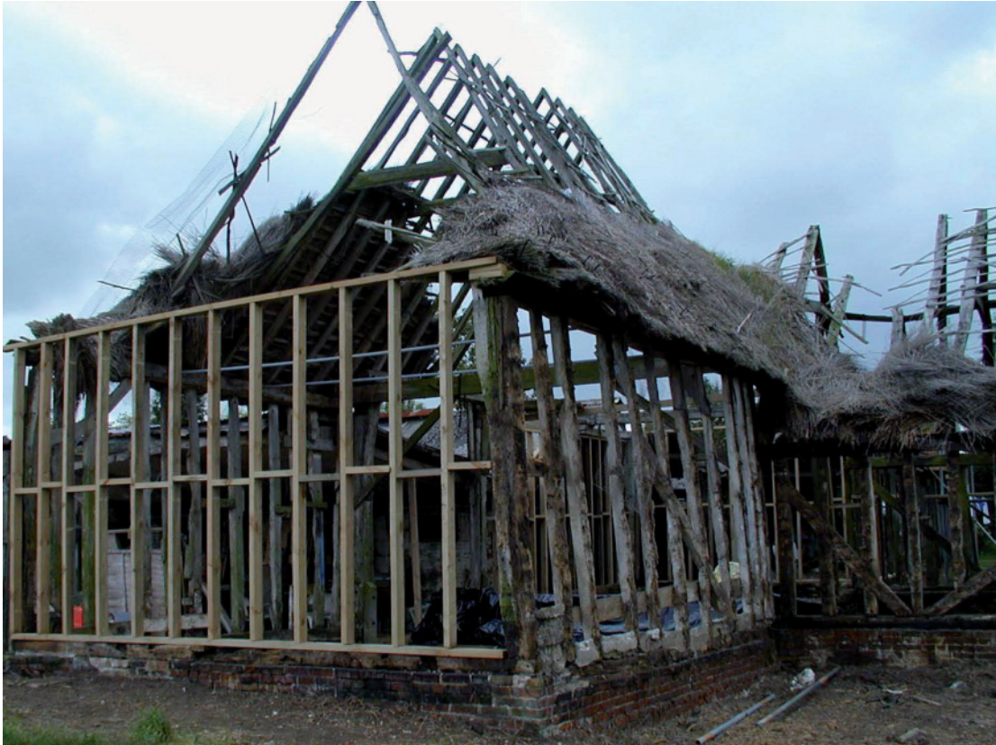
Illus. 2 Circa 1990s old photograph. The exterior of the barn (1) from the north-west during storm repairs showing the remains of its original thatched clasped-purlin roof.
