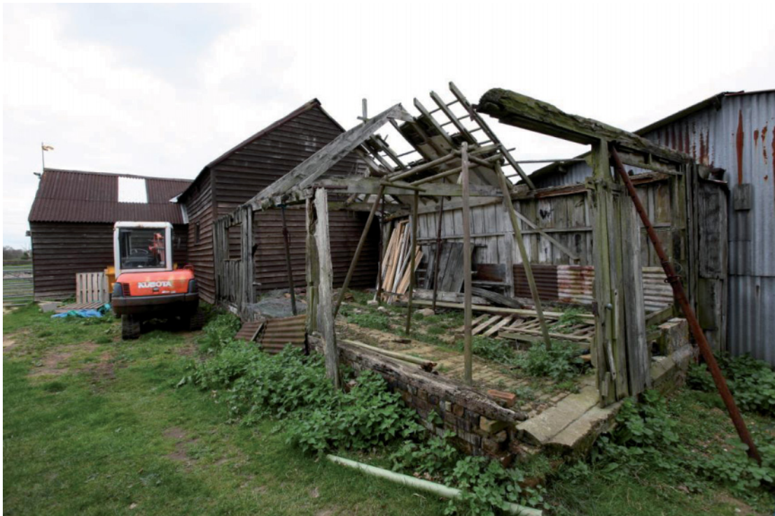
Illus. 6 The exterior of the partly dismantled southern shed (4) from the south-west showing its post-and-rail wall fabric with the barn (1) to the left and the corrugated iron southern yard shed (5) to the right.
