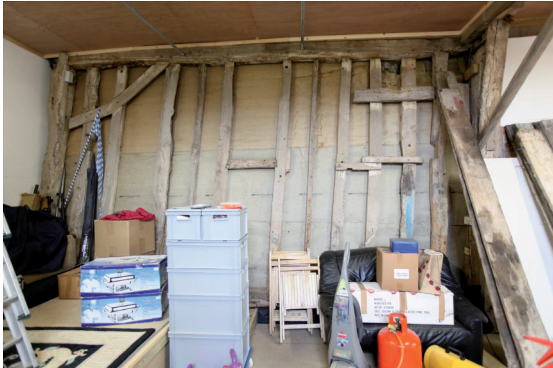
Illus. 9 The eastern interior of the barn's northern bay (1a) showing the intact early-17th century frame with original reverse-cranked trenched brace to left. A number of additional studs have been inserted between the original timbers.
