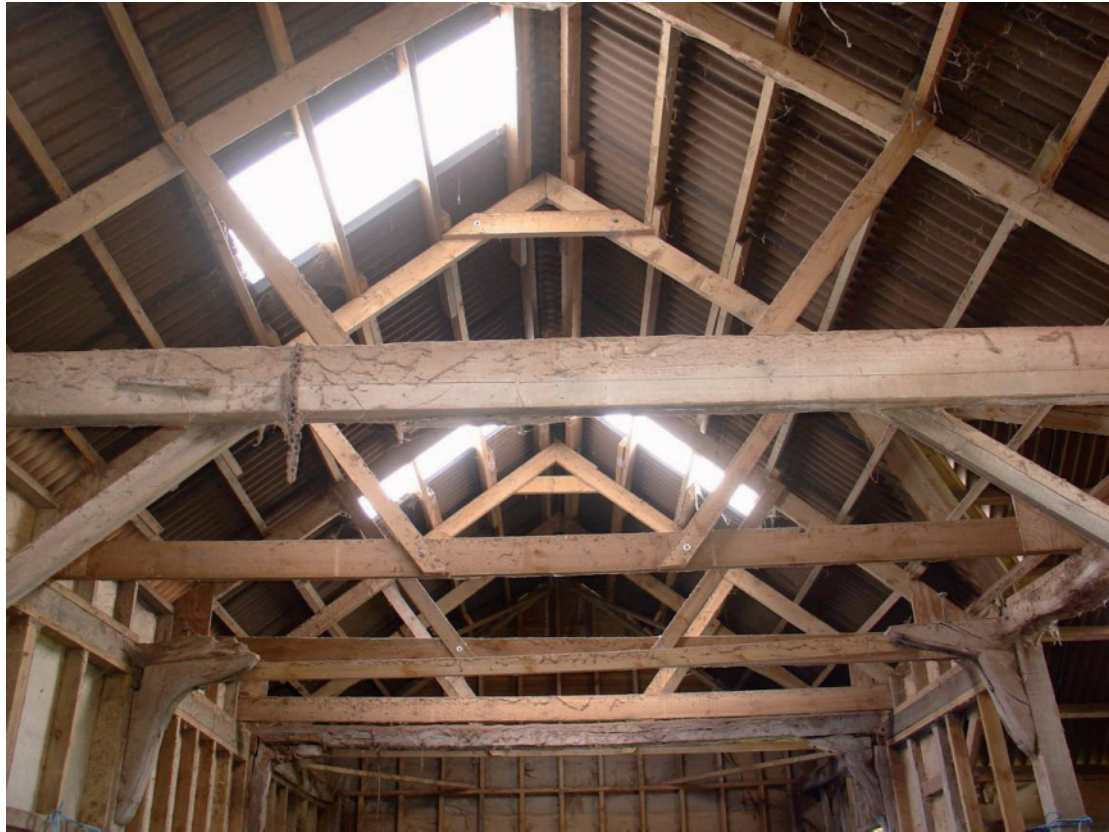
Illus. 3 2006 old photograph. The interior of the barn (1) from the north showing the largely 20 th century softwood timber of its walls and roof (all hidden by boarding at the time of inspection)
