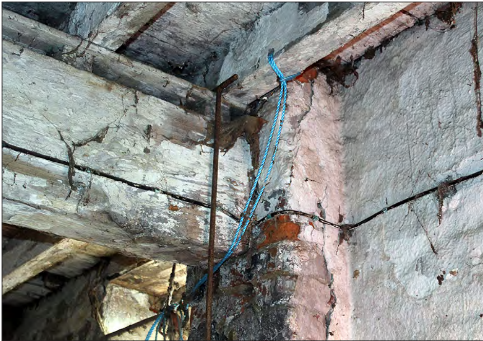
Plate 96. Building 5, interior. Ground floor west side room, ceiling cross-beam and joists. View looking southeast
