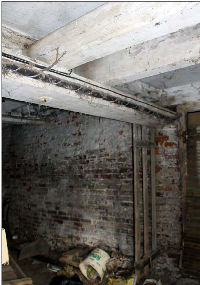
Plate 103. Building 5, interior. Ground floor east side room, east elevation. View looking north
