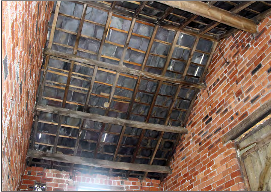
Plate 193. Building 8, interior. First floor of the east side room, roof structure. View looking north
