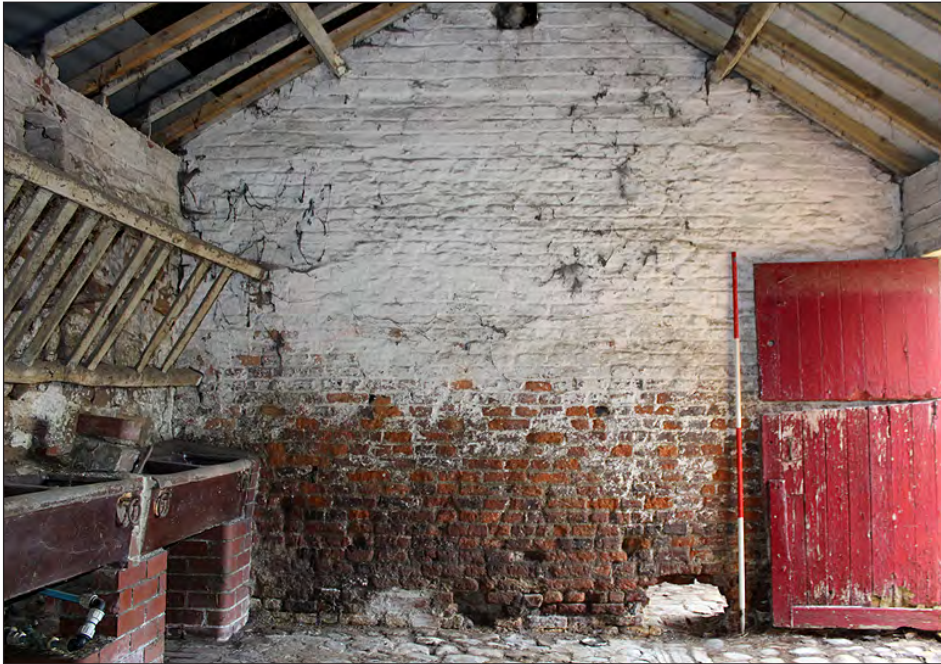
Plate 157. Building 7, interior. South elevation of the north side room. View looking south-southeast
