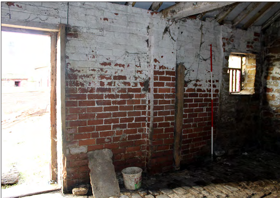
Plate 158. Building 7, interior. West elevation of the north side room. View looking northwest
