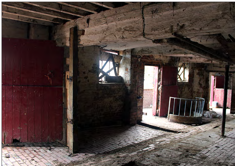
Plate 88. Building 5, interior. Ground floor west side room, south elevation. View looking southeast
