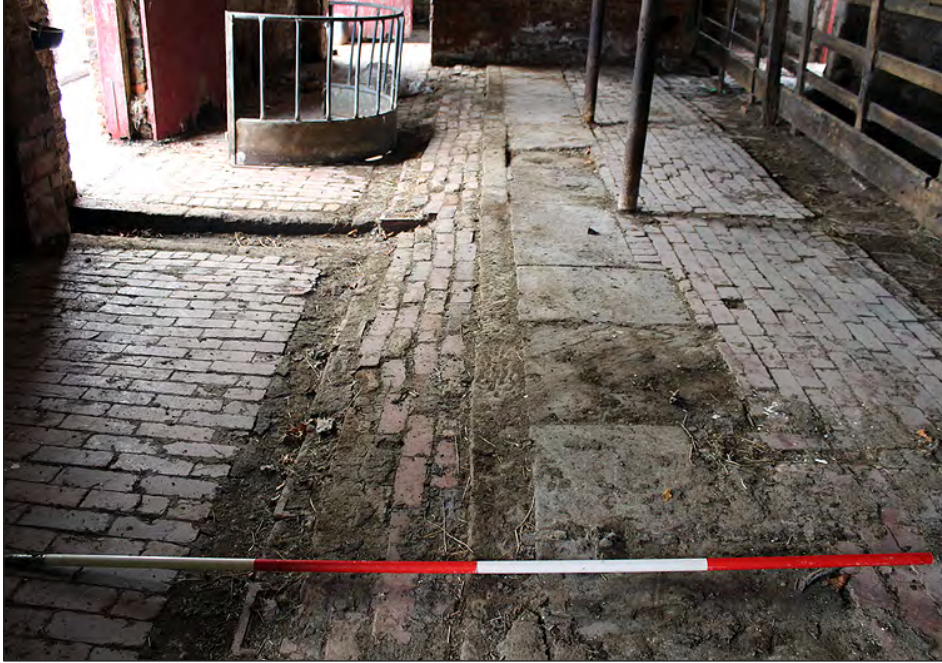
Plate 93. Building 5, interior. Ground floor west side room, floor surface. View looking west-southwest
