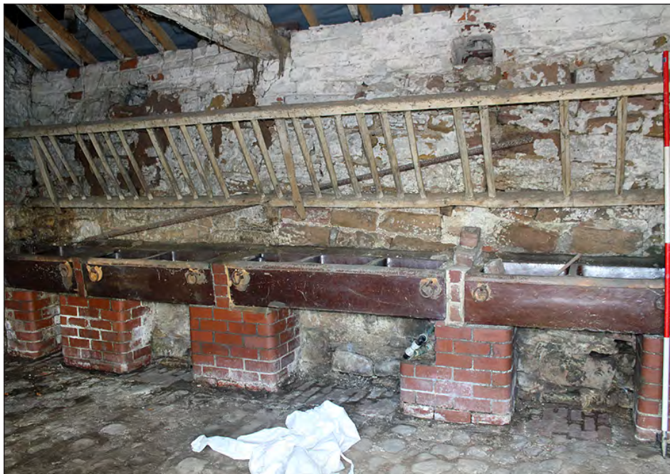
Plate 156. Building 7, interior. East elevation of the north side room. View looking northeast
