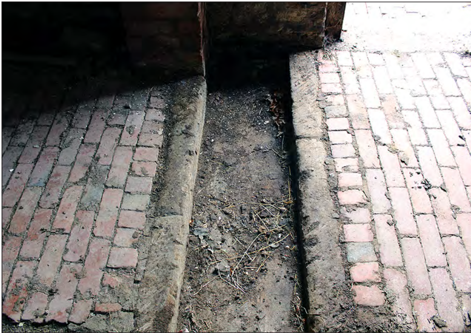
Plate 94. Building 5, interior. Ground floor west side room, floor surface drainage channel. View looking south
