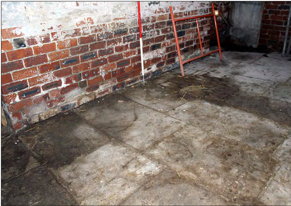
Plate 188. Building 8, interior. Floor surface of the east side room. View looking northwest
