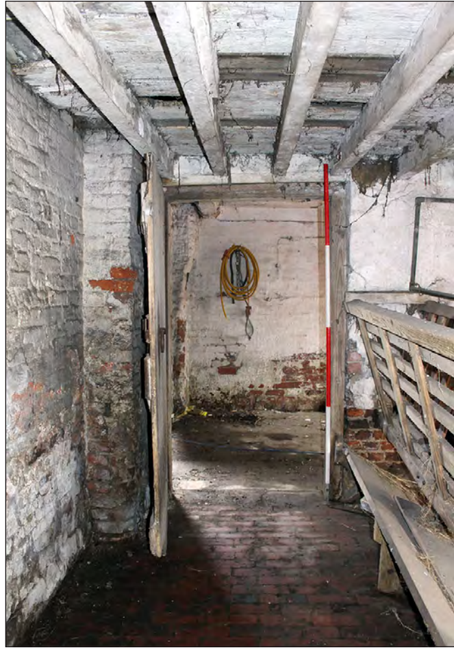
Plate 87. Building 5, interior. Ground floor west side room, north side doorway on the east elevation. View looking east-northeast
