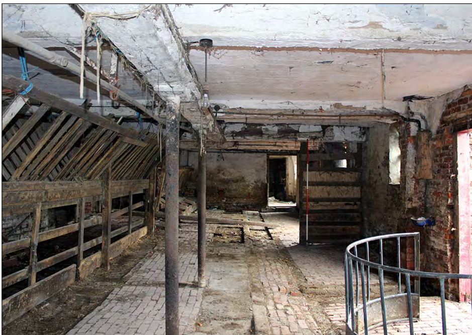
Plate 86. Building 5, interior. Ground floor east end of the west side room. View looking east-northeast
