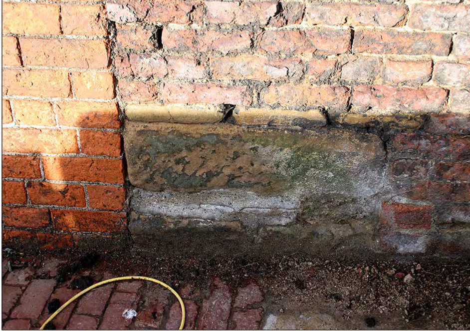
Plate 77. Building 5. Stone masonry to the east side of the threshing door opening. View looking north-northwest
