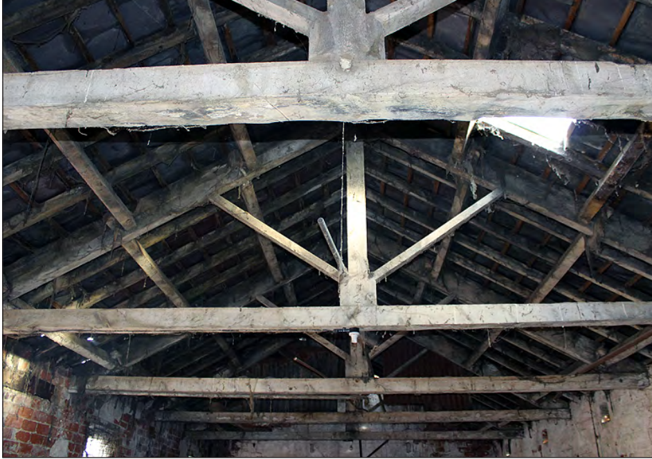
Plate 181. Building 8, interior. Roof structure of the west side room. View looking east-northeast
