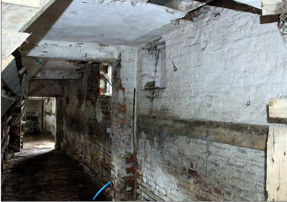
Plate 81. Building 5, interior. Ground floor west side room, view along north elevation. View looking west-southwest
