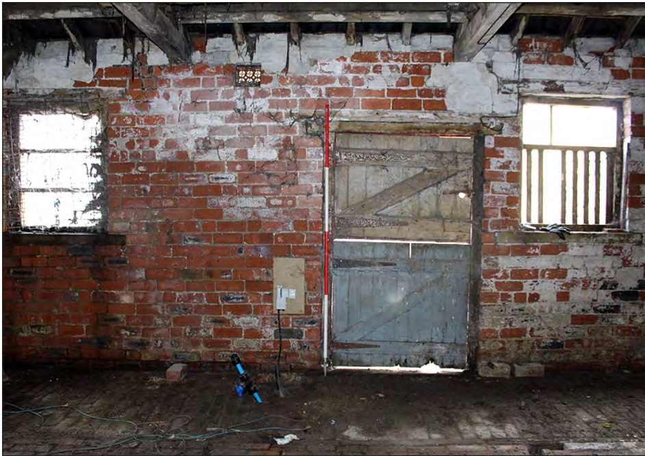
Plate 174. Building 8, interior. East end of the north elevation of the west side room. View looking north-northwest
