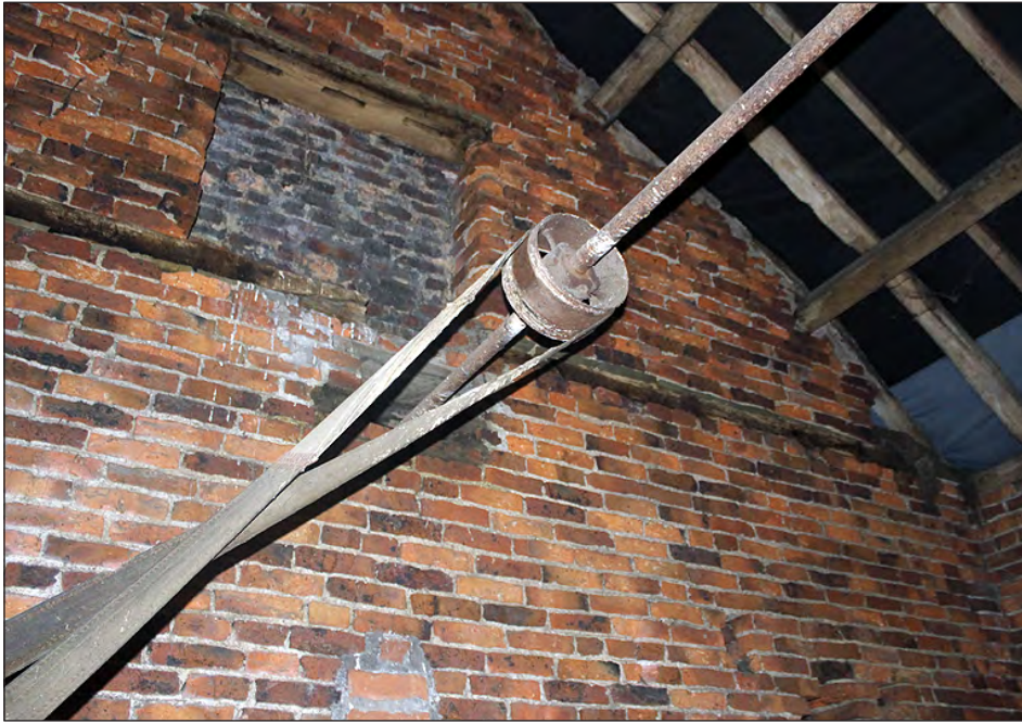
Plate 115. Building 5, interior. In situ drive belt, wheel and line shaft. View looking southeast
