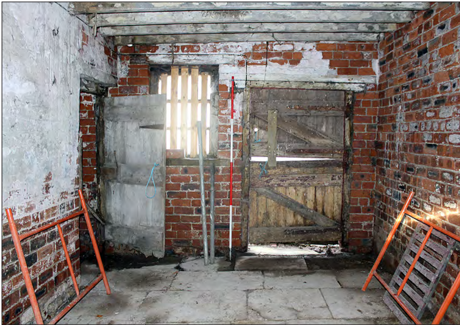
Plate 182. Building 8, interior. North elevation of the ground floor east side room. View looking north-northwest
