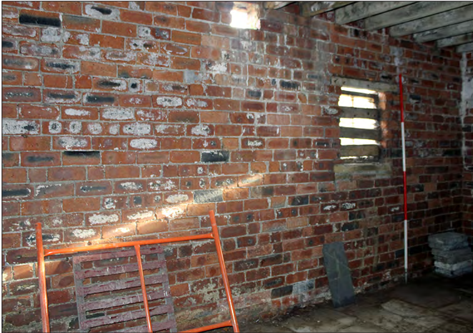
Plate 183. Building 8, interior. East elevation of the ground floor east side room. View looking northeast
