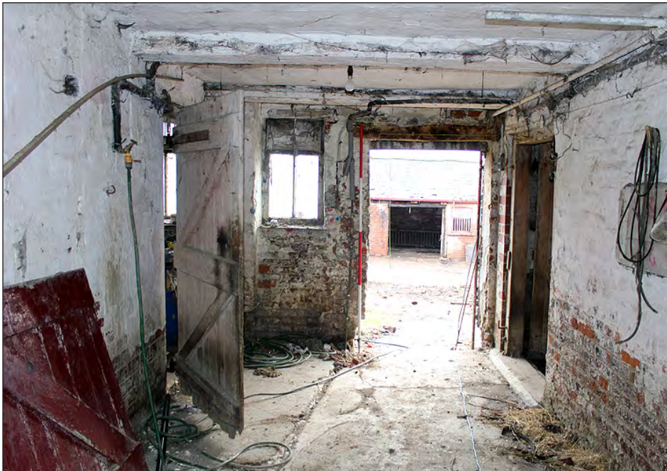
Plate 98. Building 5, interior. Ground floor, south side of the cross-passage. View looking south-southeast
