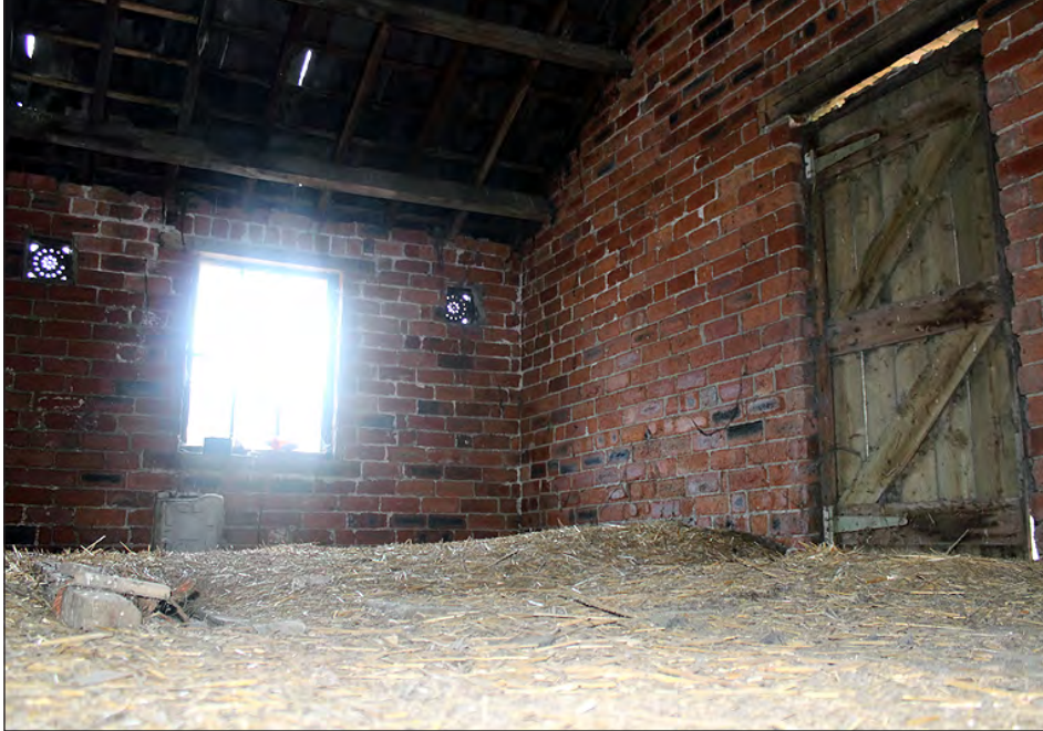
Plate 191. Building 8, interior. First floor of the east side room. View looking north
