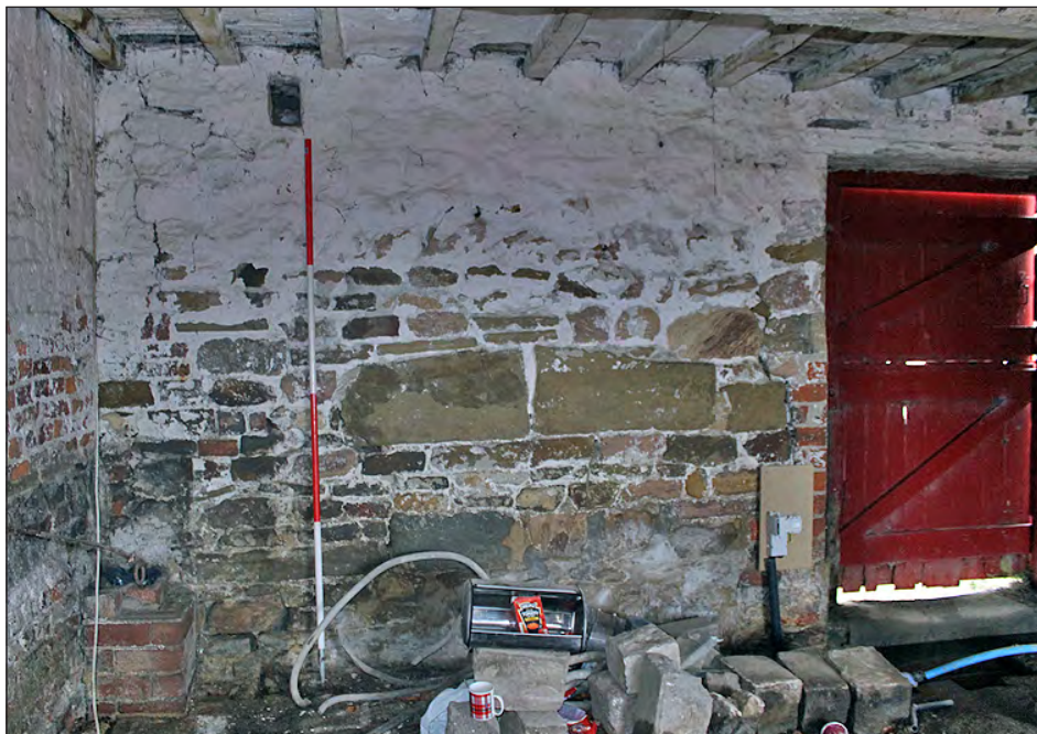
Plate 44. Building 4, interior. North elevation of the ground floor west side room. View looking north-northwest
