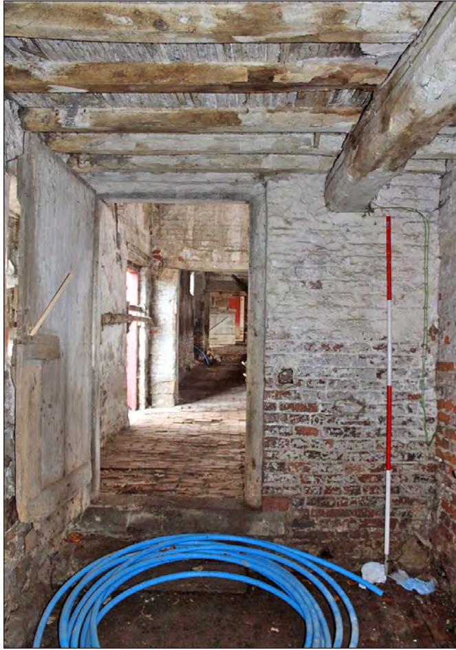
Plate 45. Building 4, interior. North end of the east elevation of the ground floor west side room. View looking east-northeast
