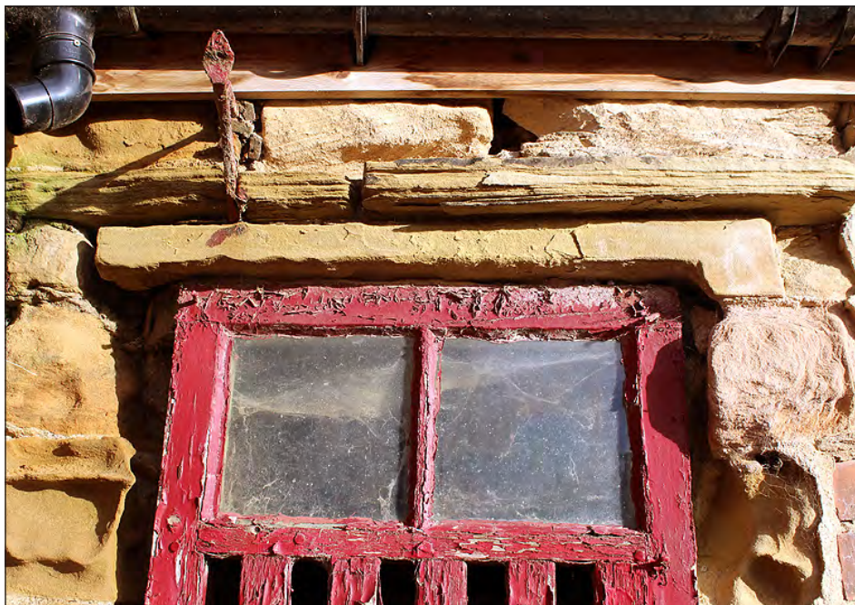
Plate 154. Building 7. North end of west elevation, showing window detail. View looking east-northeast
