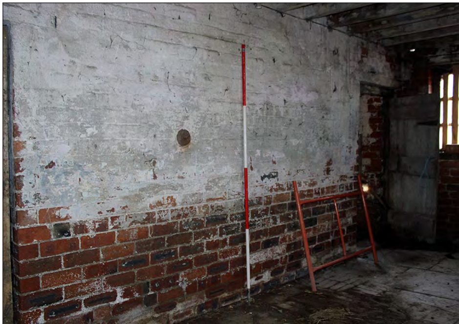
Plate 186. Building 8, interior. West elevation of the ground floor east side room. View looking northwest
