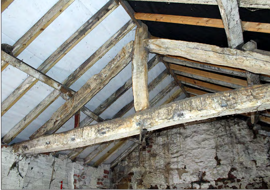
Plate 161. Building 7, interior. Roof structure of the north side room. View looking northwest
