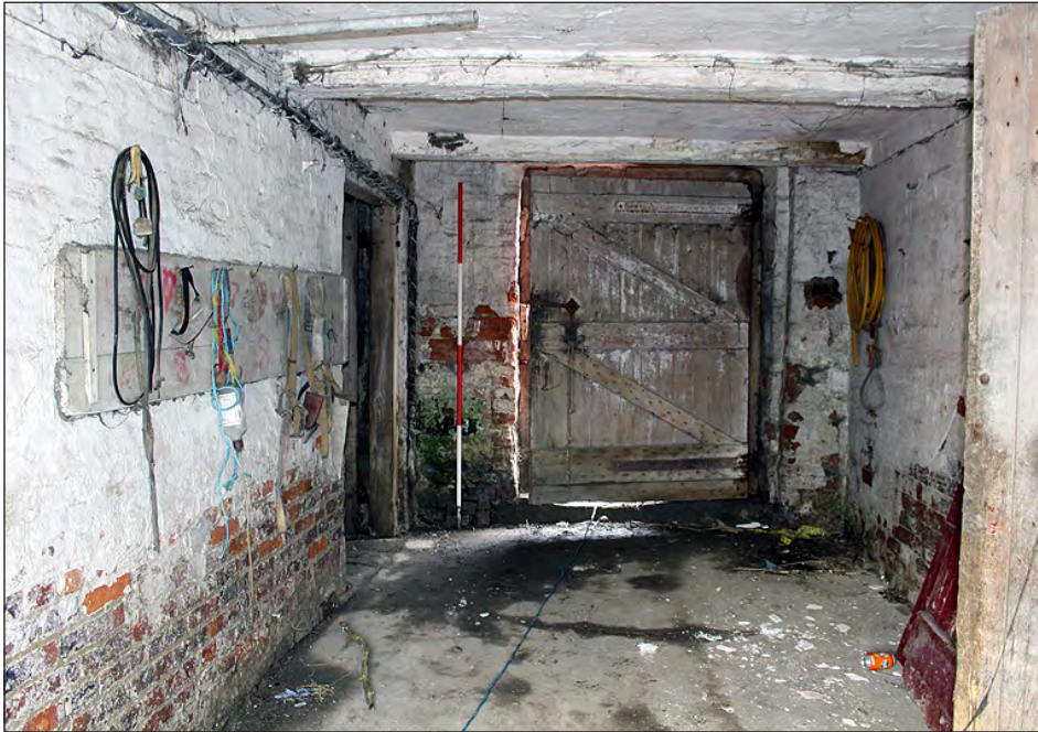
Plate 97. Building 5, interior. Ground floor, north side of the cross-passage. View looking north-northwest
