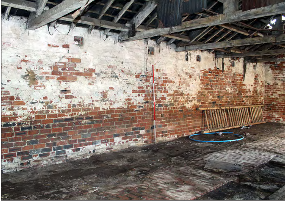
Plate 177. Building 8, interior. South elevation of the west side room. View looking southwest
