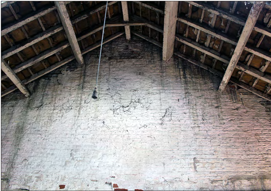
Plate 52. Building 4, interior. Upper section of the east elevation of the east side room. View looking east-northeast
