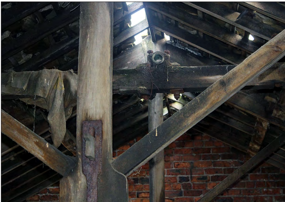
Plate 148. Building 6, interior. In situ plumbers block bearing for a line shaft, leading to former engine location. View looking northeast
