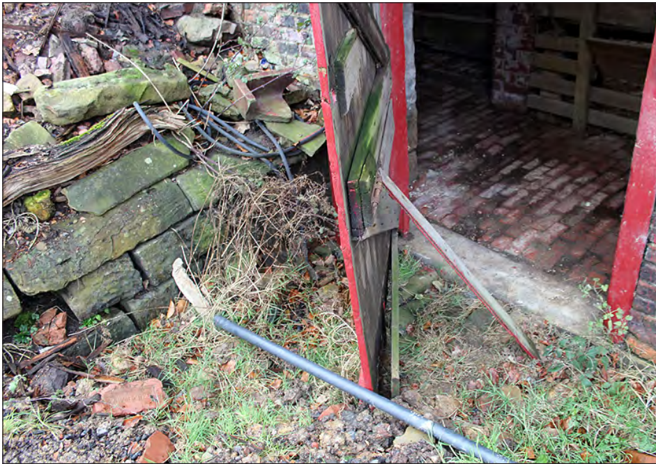
Plate 38. Building 4. Wall abutting the north elevation and partially visible cobble surface. View looking southeast
