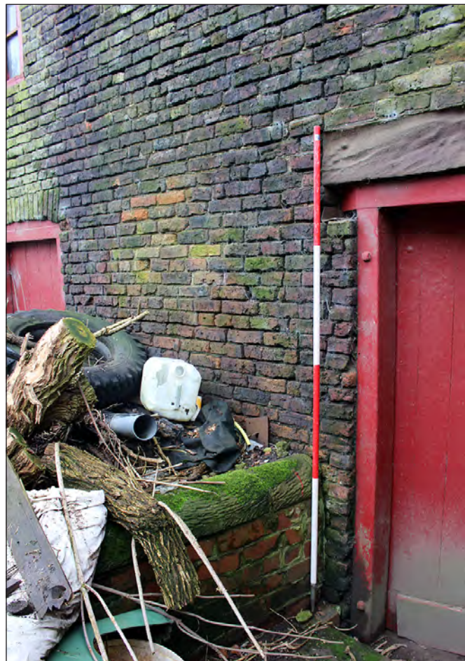
Plate 72. Building 5. Wall abutting north elevation towards the east end. View looking south-southeast
