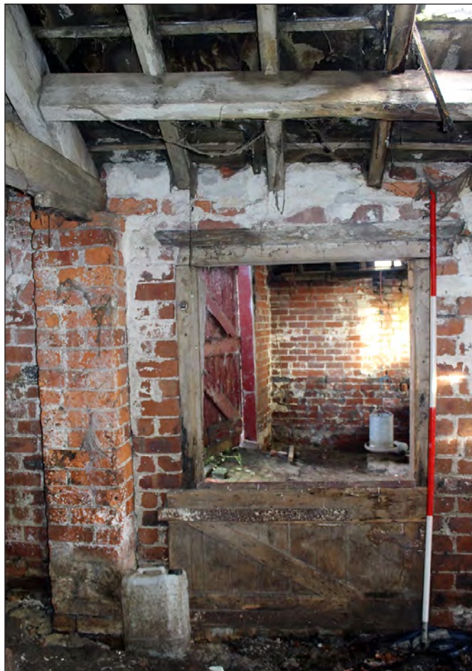
Plate 216. Building 10, interior. Doorway on the east elevation, leading to Building 9. View looking east-northeast
