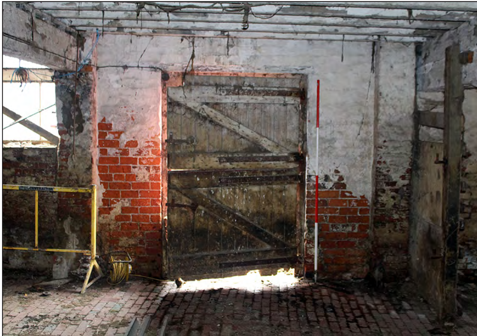
Plate 90. Building 5, interior. Ground floor west side room, south side threshing door. View looking south-southeast
