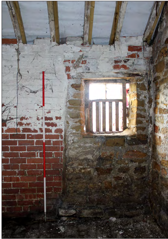
Plate 159. Building 7, interior. North end of the west elevation of the north side room. View looking west-southwest
