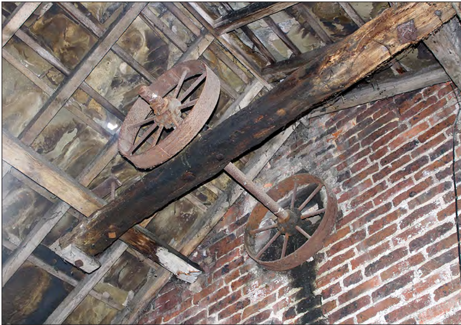
Plate 146. Building 6, interior. In situ line shaft and wheels. View looking west-southwest
