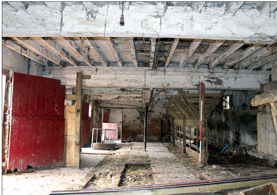
Plate 92. Building 5, interior. Ground floor, west end of the west side room. View looking west-southwest
