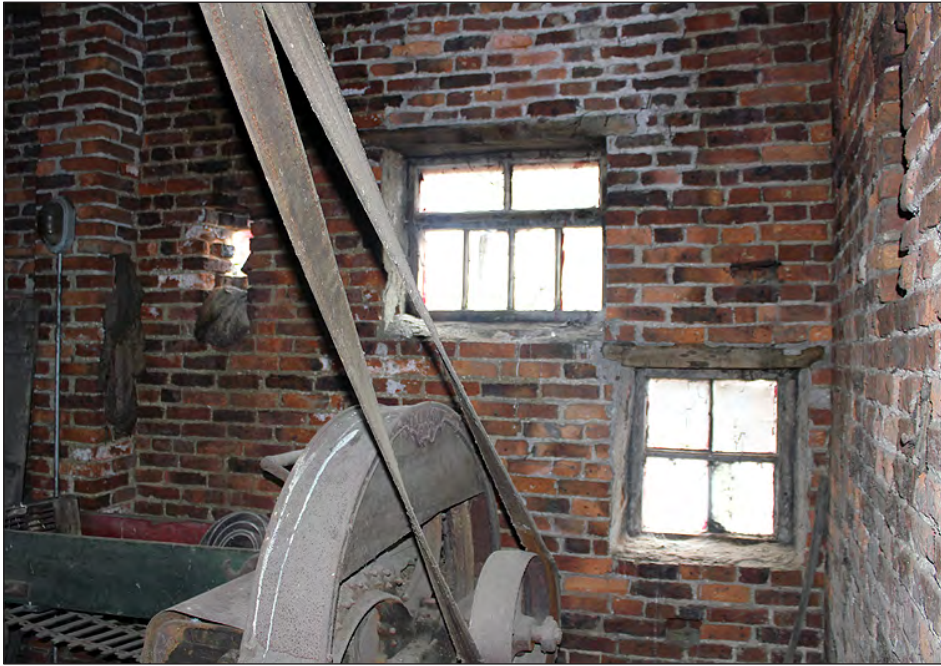
Plate 107. Building 5, interior. First floor, east end of the north elevation. View looking north-northwest
