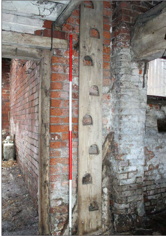
Plate 85. Building 5, interior. Ground floor west side room, showing Jacob's ladder. View looking north
