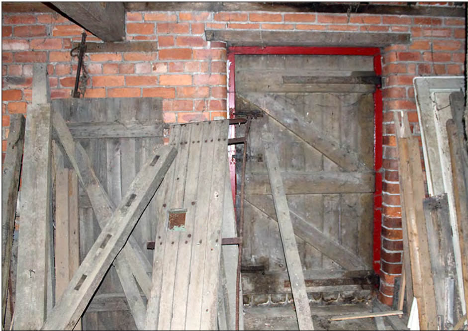
Plate 30. Building 3, interior. Taking-in door on the north wall of the first floor. View looking north-northwest
