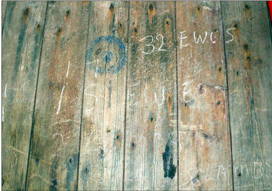
Plate 101. Building 5, interior. Ground floor cross-passage, graffiti on the south side door. View looking south-southeast
