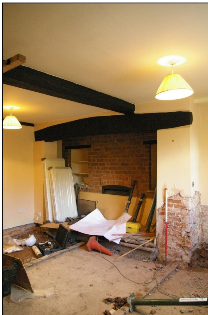
Plate 5. Room 1, looking south-east, showing the spine beam T4 supported on the fireplace bressumer T6.
