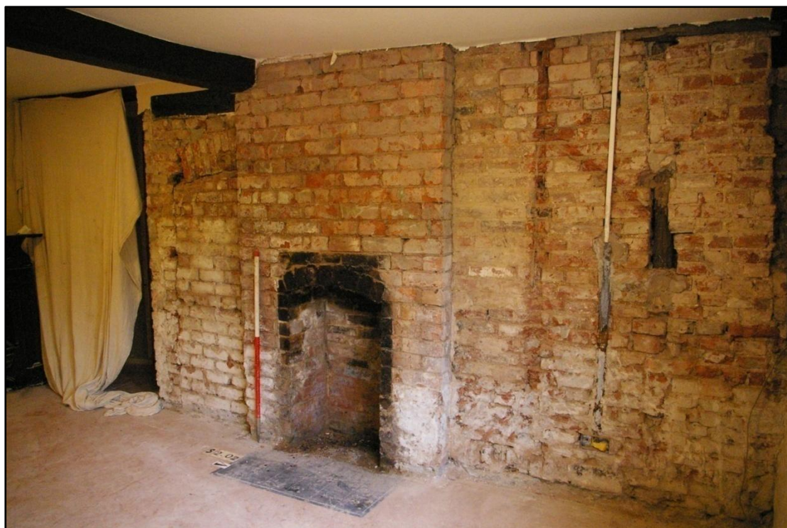
Plate 6. Room 2, looking south-west, showing the spine beam T8 at ceiling level and remnants of wall framing T10, T11 and T12 embedded in the brickwork of the west wall of Room 2.
