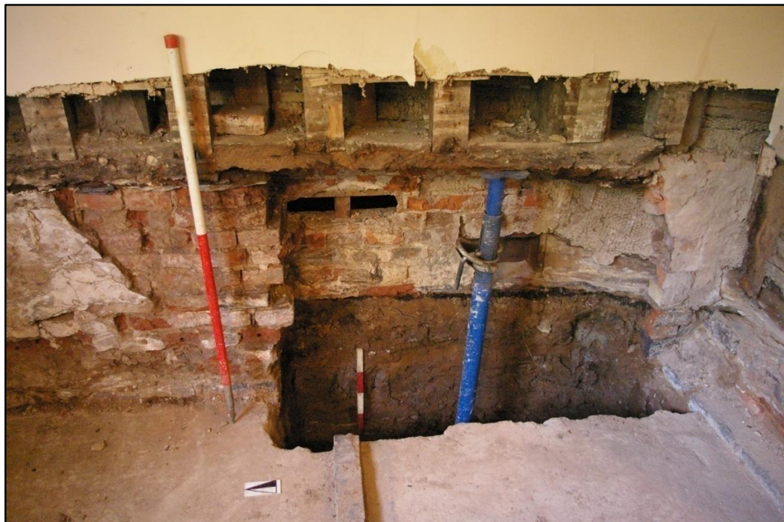
Plate 4. Room 1, west wall. Sill beam T1 and studs T2 and T3, partially obscured by later studwork to lath and plaster wall covering.
