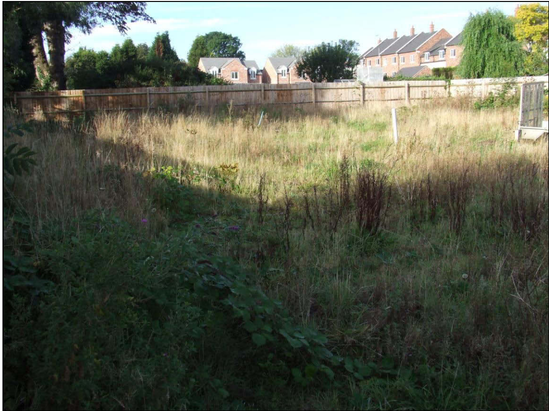
Figure 2 Rear of the site looking west, showing new fencing and spoil heap behind.
