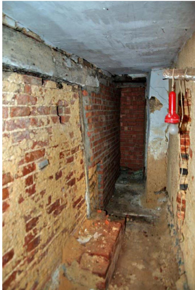
Figure 13 Looking east. Note recent brick wall to rear left hand side and rear; doorframe lintel to rear; stone (plastered) east wall forming door opening to rear right hand side. Broken brickwork visible behind inspection lamp is where the wall to the right hand side was broken through for access.
