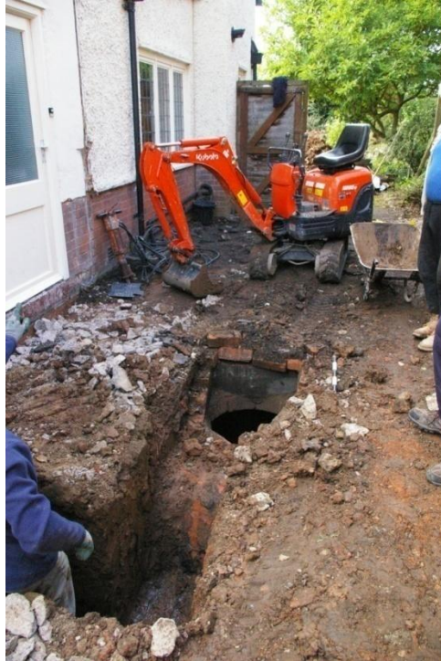
Plate 3: Modern brick bell-pit soft water tank found within foundation trench (Looking west)
