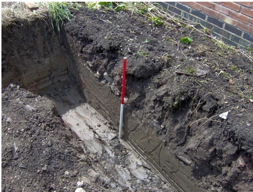
Figure 4: The south-west corner of the footing, looking south, showing stone layer (3) resting on natural clay (5)
